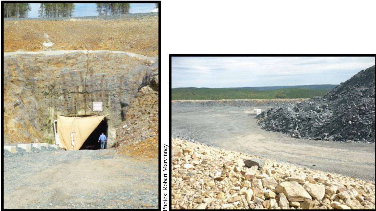
Waste rock management at a modern mine. Halfmile Mine, New Brunswick, opened in 2012. Entrance to underground mine on left. Pad for potentially acid-generating waste rock on right. Every 1,000 tons of waste rock (about 10,000 cubic feet) is tested for acid-generating potential. Waste rock with a high potential to generate acid will be returned to backfill the mine as mining progresses.
