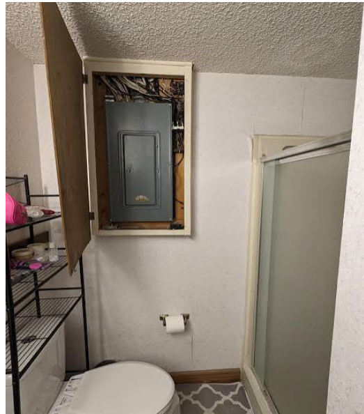
EXAMPLE VIOLATION OF NEC ARTICLE 240.24
