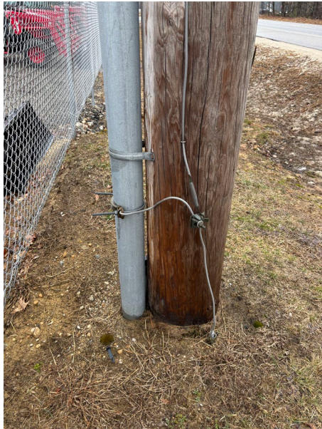
EXAMPLE OF PROPER CONDUIT GROUNDING ON THE SERVICE LATERAL
