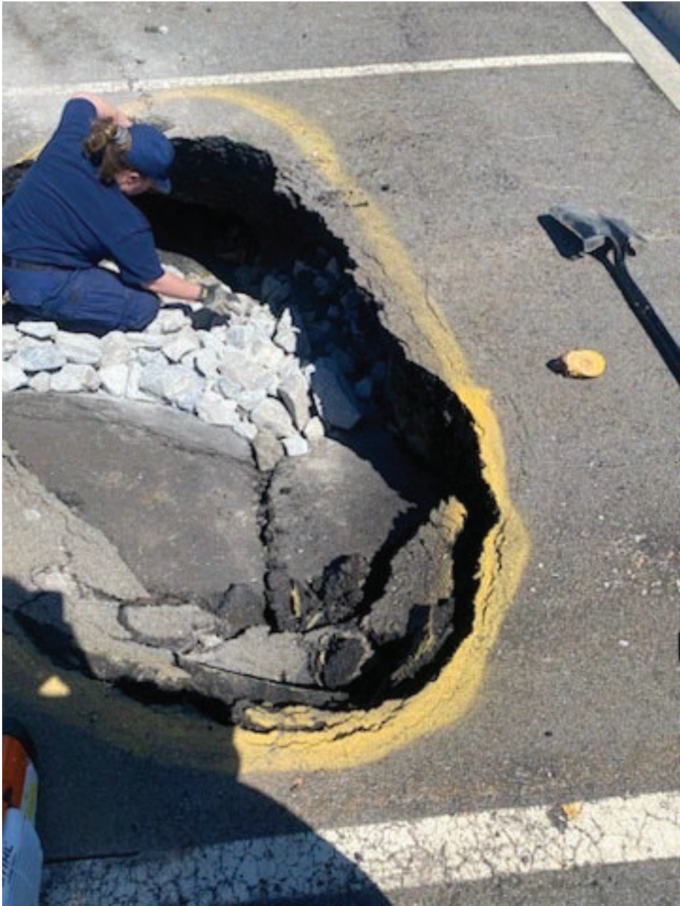
Large sink hole
