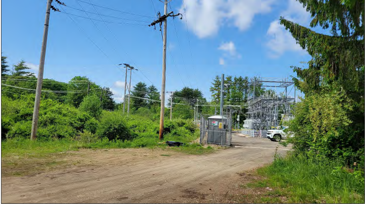
Figure 14. View south of existing Bolt Hill substation.
