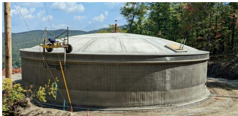
New Water Association Reservoir
