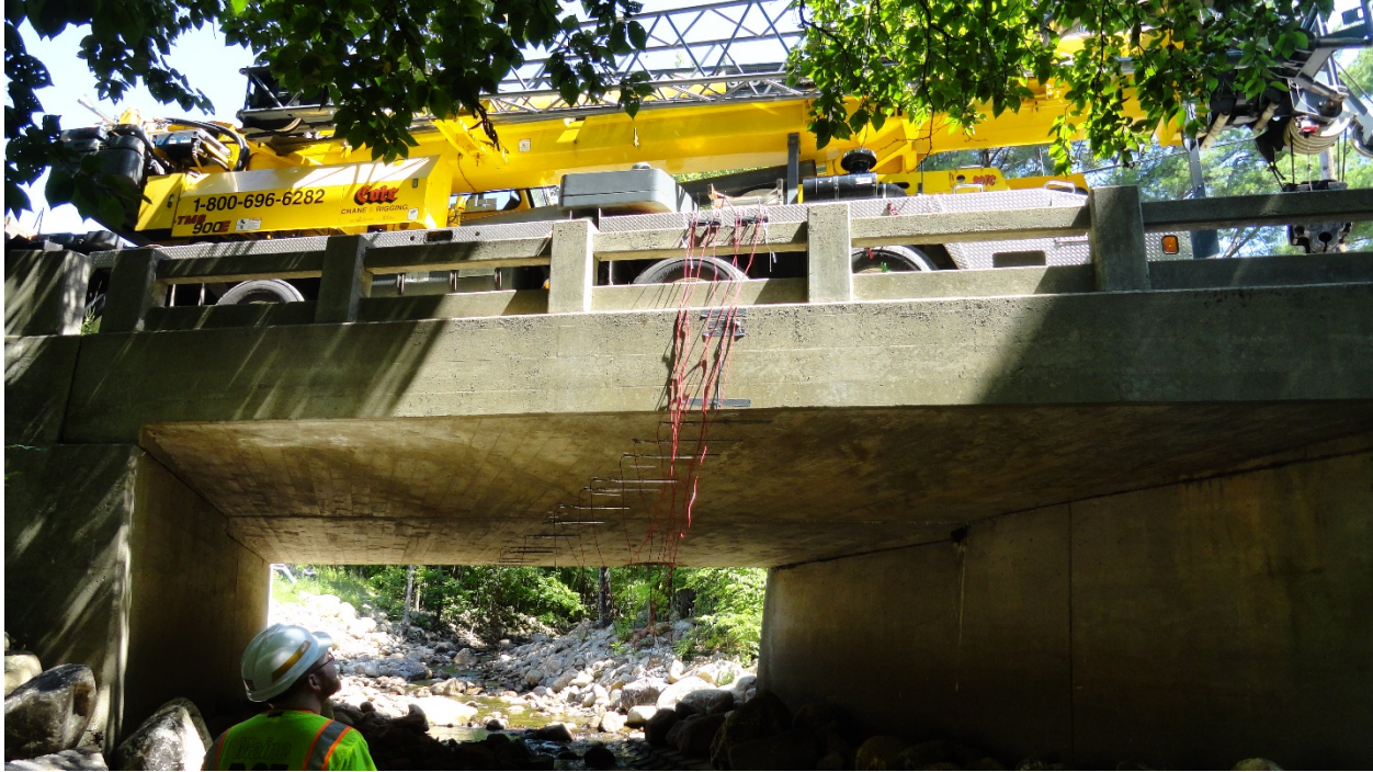
Figure 7: Weld No. 5361 general condition
