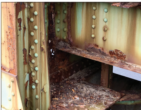
Holes in the floor beam.
