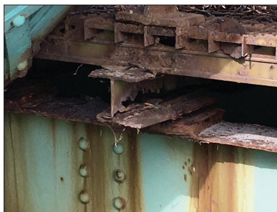
Severe corrosion to a beam near span one of the non-sidewalk truss.
