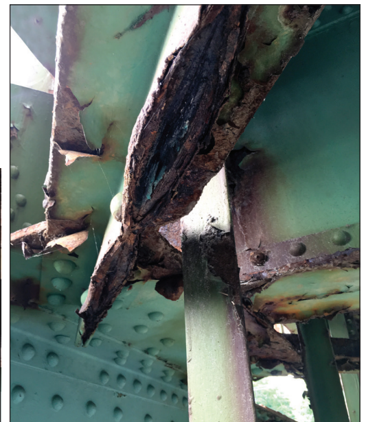
Severe corrosion to the rivets as well as corrosion and rust between the floor beams and the cover plate.
