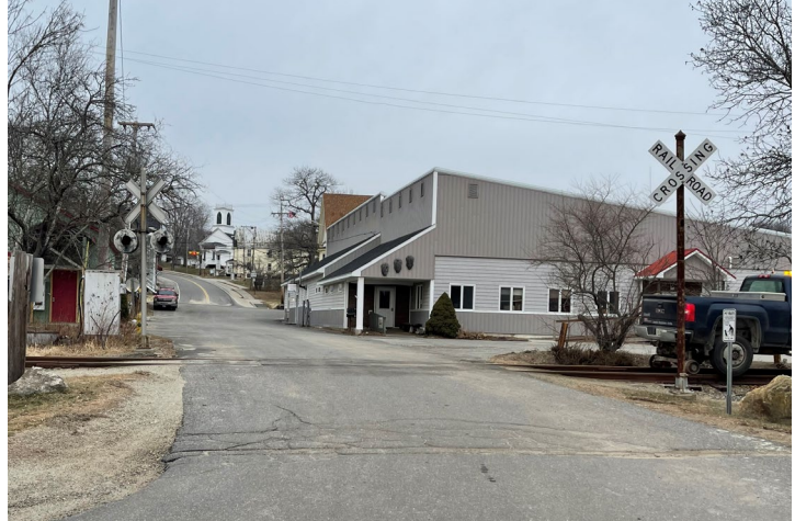
Example of non-functioning AHCW System equipment on Main St in Bowdoinham at MP 36.98
