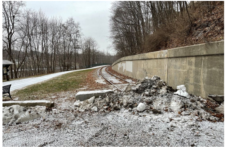
End of the existing track under the Veteran's Memorial Bridge (looking south) at MP 62.34
