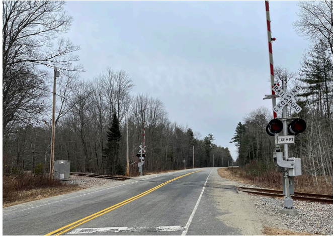
Functioning AHCW system on Rt. 24 in Bowdoinham at MP 40.55
