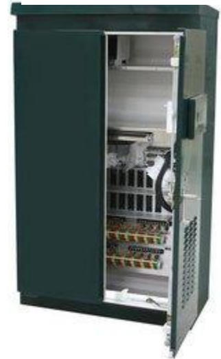
Figure 11. ATC Traffic Controller Cabinet
