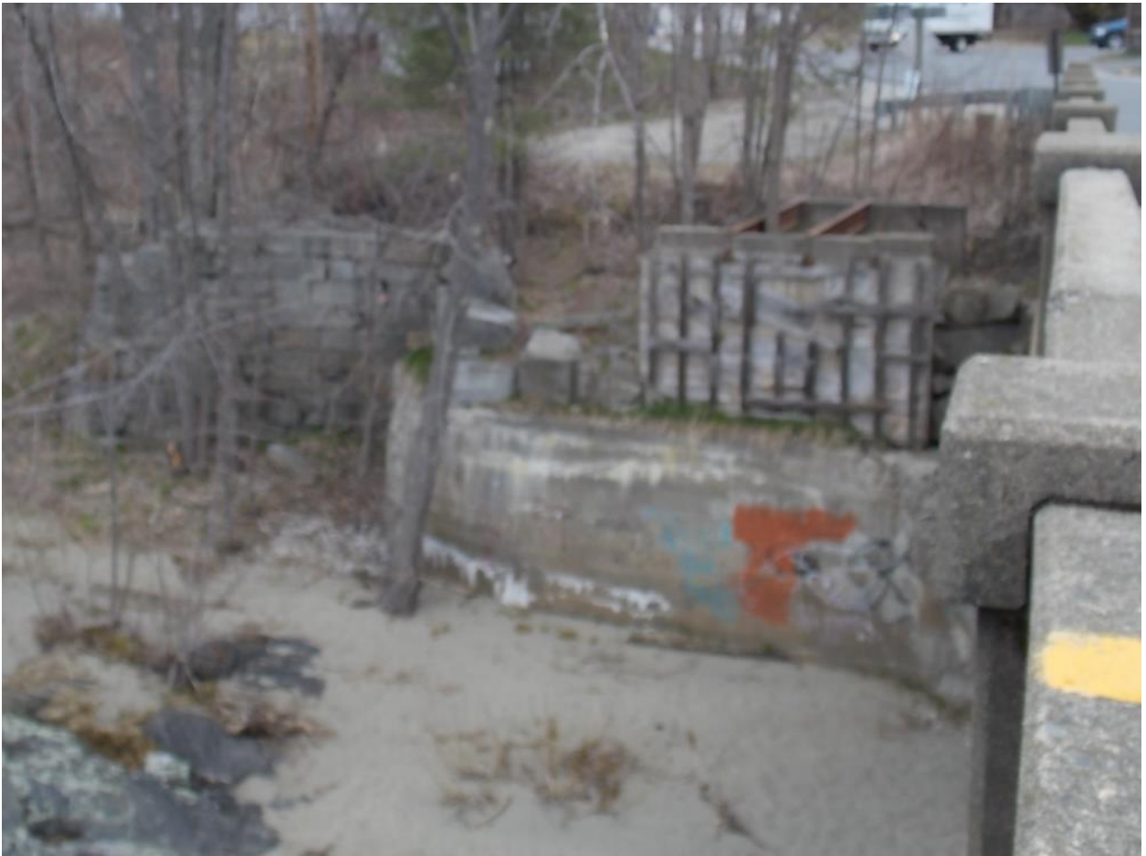
Figure 8 - Old concrete foundation and cut granite block walls located at the northwest corner of the existing bridge
