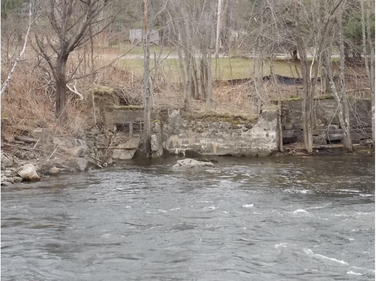
Old foundations southwest of the existing bridge (area closer to the existing bridge)
