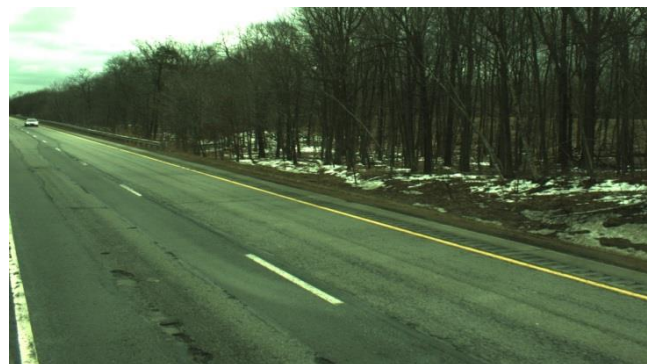
Figure 30: Pavement analysis pot holes joint failure
