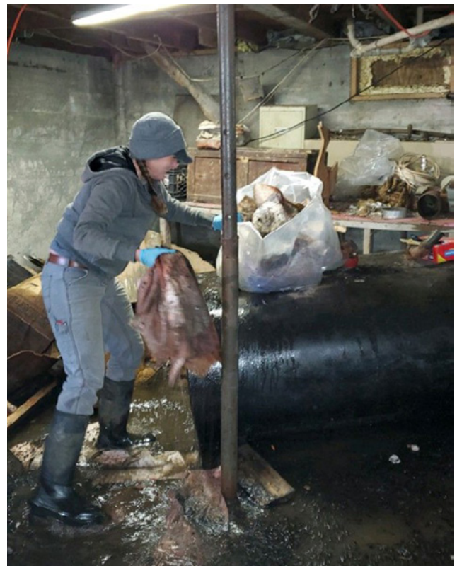
Maine Department of Environmental Protection storm remediation responders work to clean up an oil spill inside a basement in Bingham, Maine following the historic storms of 2024. Credit: Maine DEP
