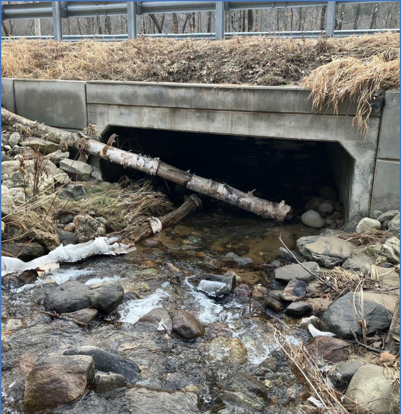
A stream crossing on Route 2 near New Sharon was improved in 2023 and survived the flooding that December. Credit: Maine DOT
