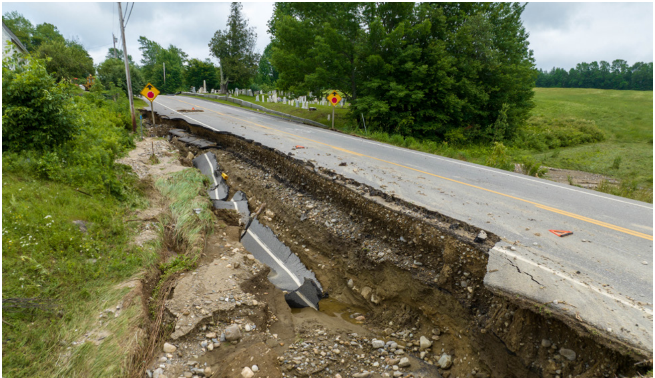
Parts of Route 133 in Jay, Maine sustained heavy damage from runoff during an historic summer rainfall in June 2023 that required months of repairs. Credit: Maine DOT
