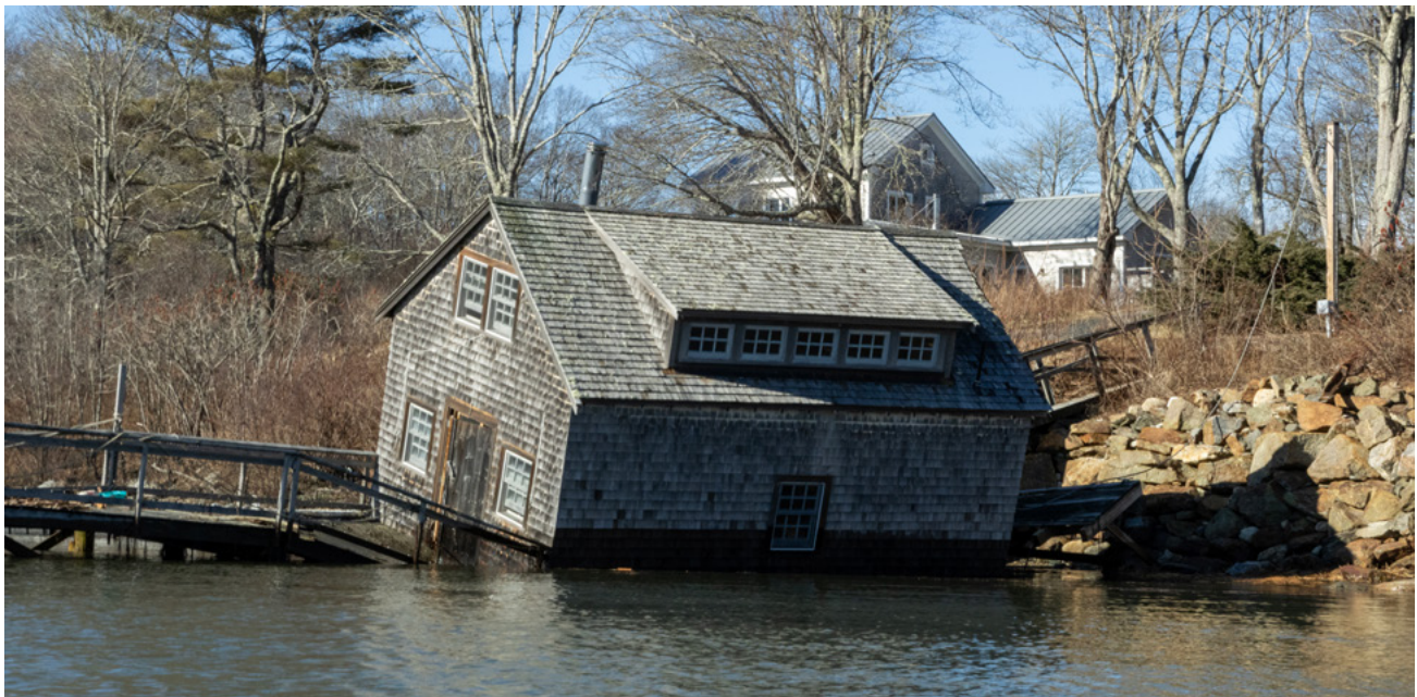
Damaged working waterfront structures in New Harbor show the force of storm surge on waterfront infrastructure. Credit: Island Institute
