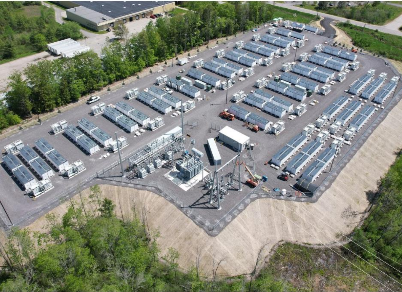
Cross Town Energy Storage in Gorham. Plus Power photo
