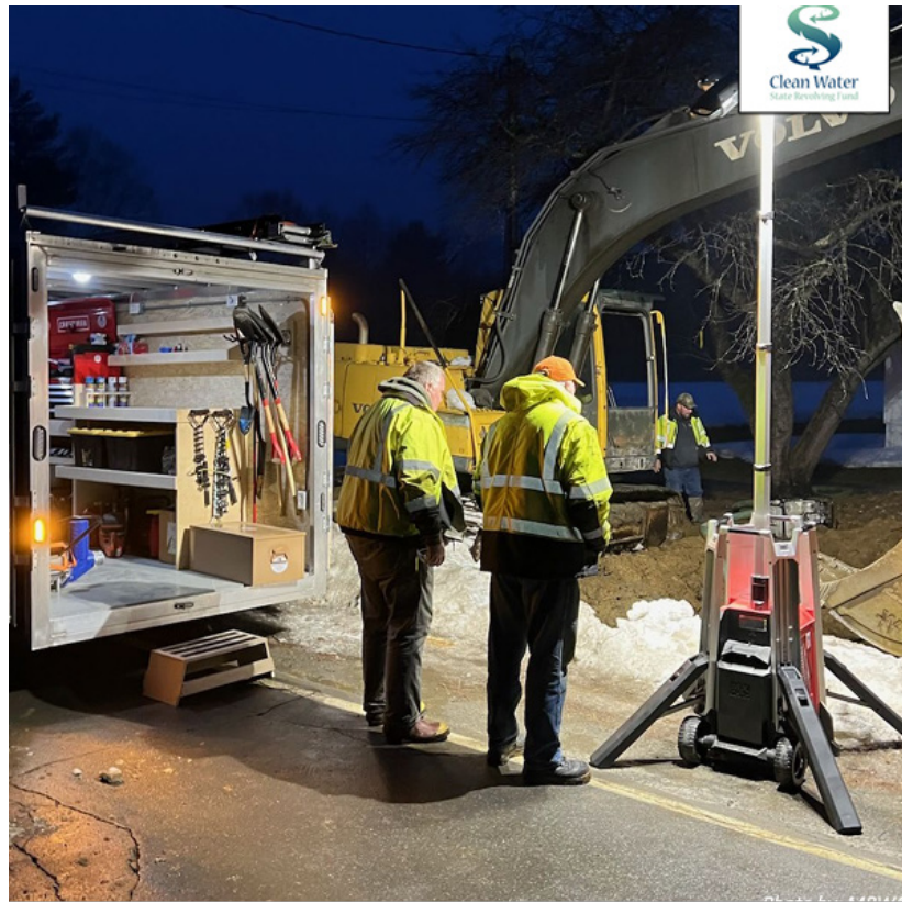
Wastewater workers utilize the Maine Rural Water Association's new emergency training and response trailer
