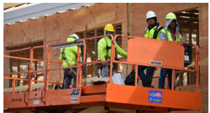
Workers at the Snow School project in Fryeburg constructing 28 affordable homes for older Mainers. Earlier this year, Governor Mills and the Legislature approved $70 million in additional funding to build similar affordable housing units across the state. (Photo credit: Avesta Housing)
