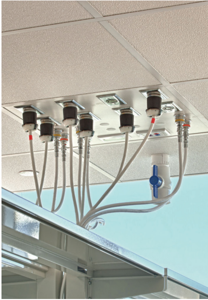
Ceiling Interface Panels [CIPs] are configured to the exact requirements of your lab; with the ability to accommodate future expansions.
