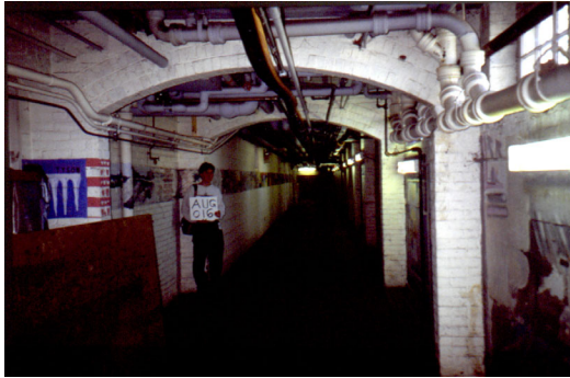
Much of the infrastructure of the complex utilizes basement tunnels such as this.
