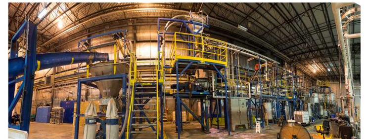
1 tpd Biomass to Bioproducts Pilot Plant (B 2 P 2 )
