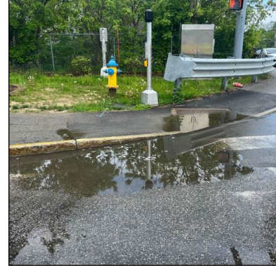
Drainage issues affect the street and sidewalk located at the southeast corner of State St and North Main Street.
