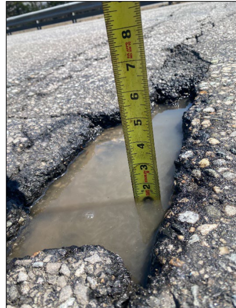
A pothole slowly deepens on I-295 in Cumberland County.
