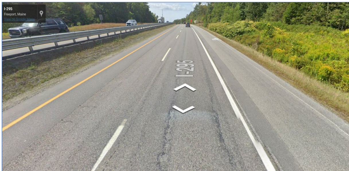
This screenshot from MaineDOT's Map Viewer via Google Streetview showing the surface condition of a segment of I-295 in Freeport. The surface of the right lane is severely deteriorating, creating elongated ruts in the pathway of vehicle wheels.
