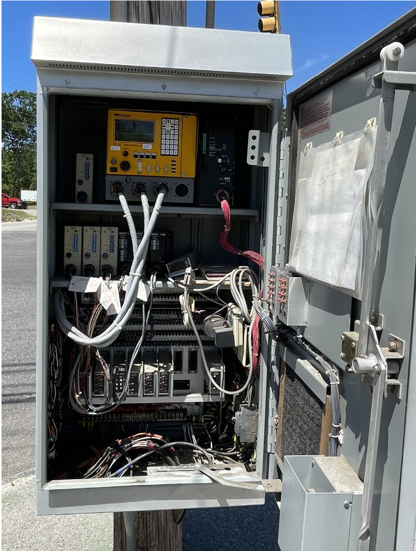
Existing 025321.00 Pole Mounted "Stretch M"-Type TS-1 Intersection Control Cabinet
