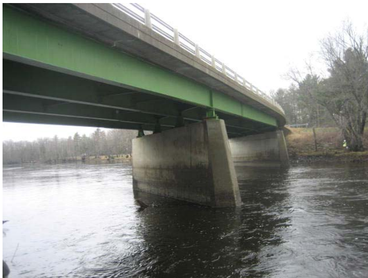
Scour Critical Feature at Low Water
