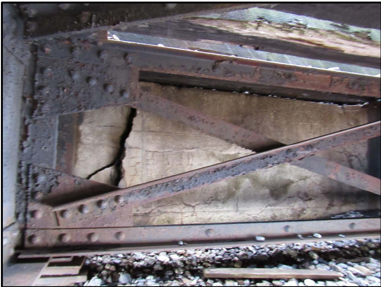
Full-Height Crack and Backwall Tipping Forward at East (Track North) Abutment
