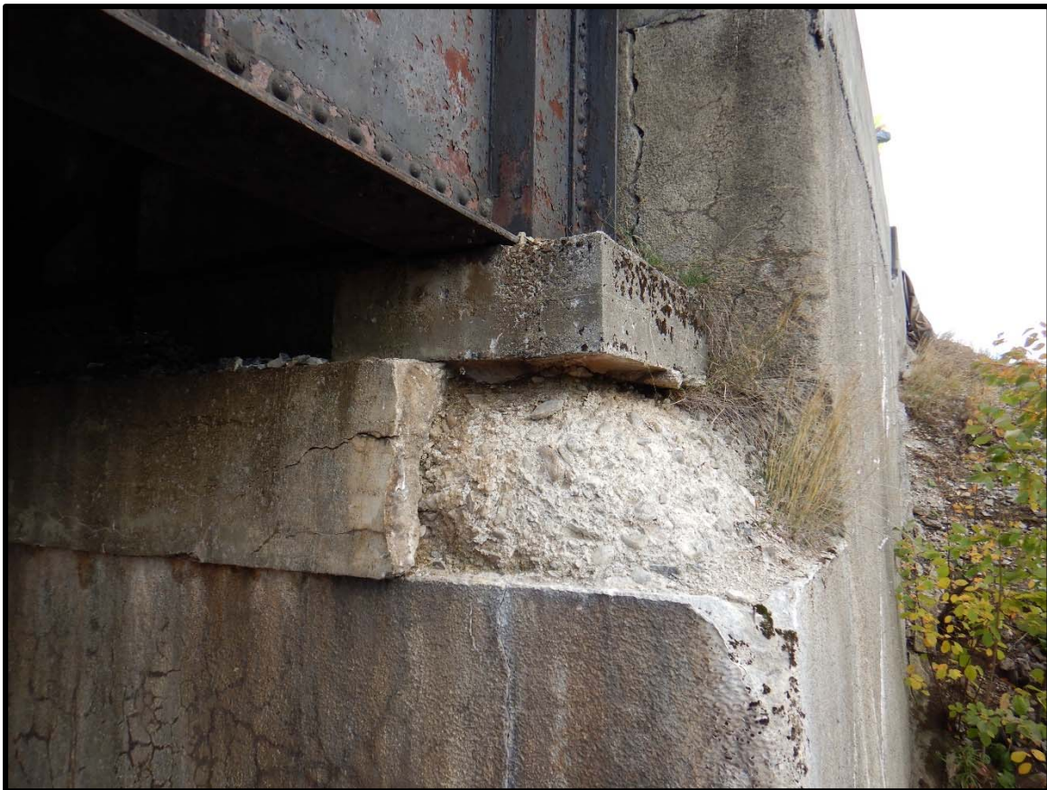
Coping Along Face of Bridge Seat Heavily Deteriorated at East Isle Abutment
