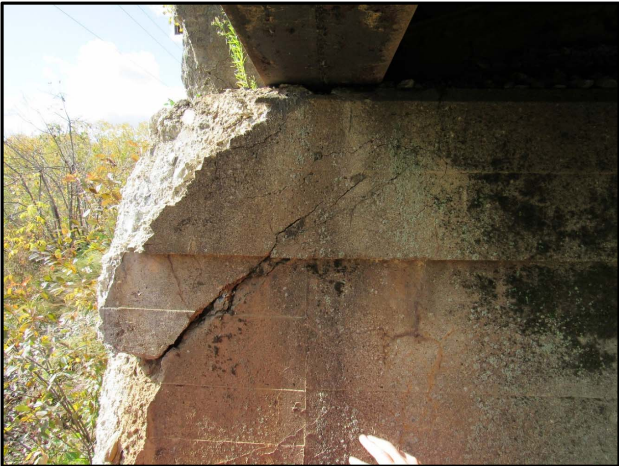
Shear Crack in Bridge Seat Under South Girder on West (Track South) Abutment
