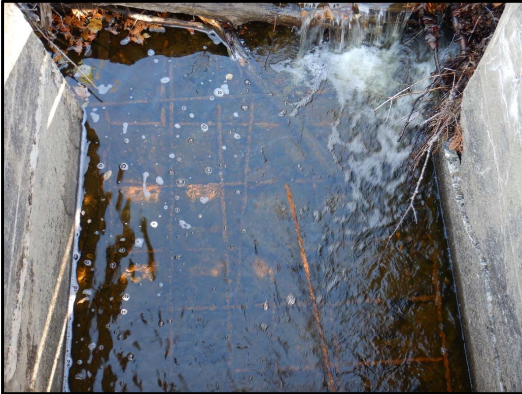
Invert Slab of North Span Completely Deteriorated
