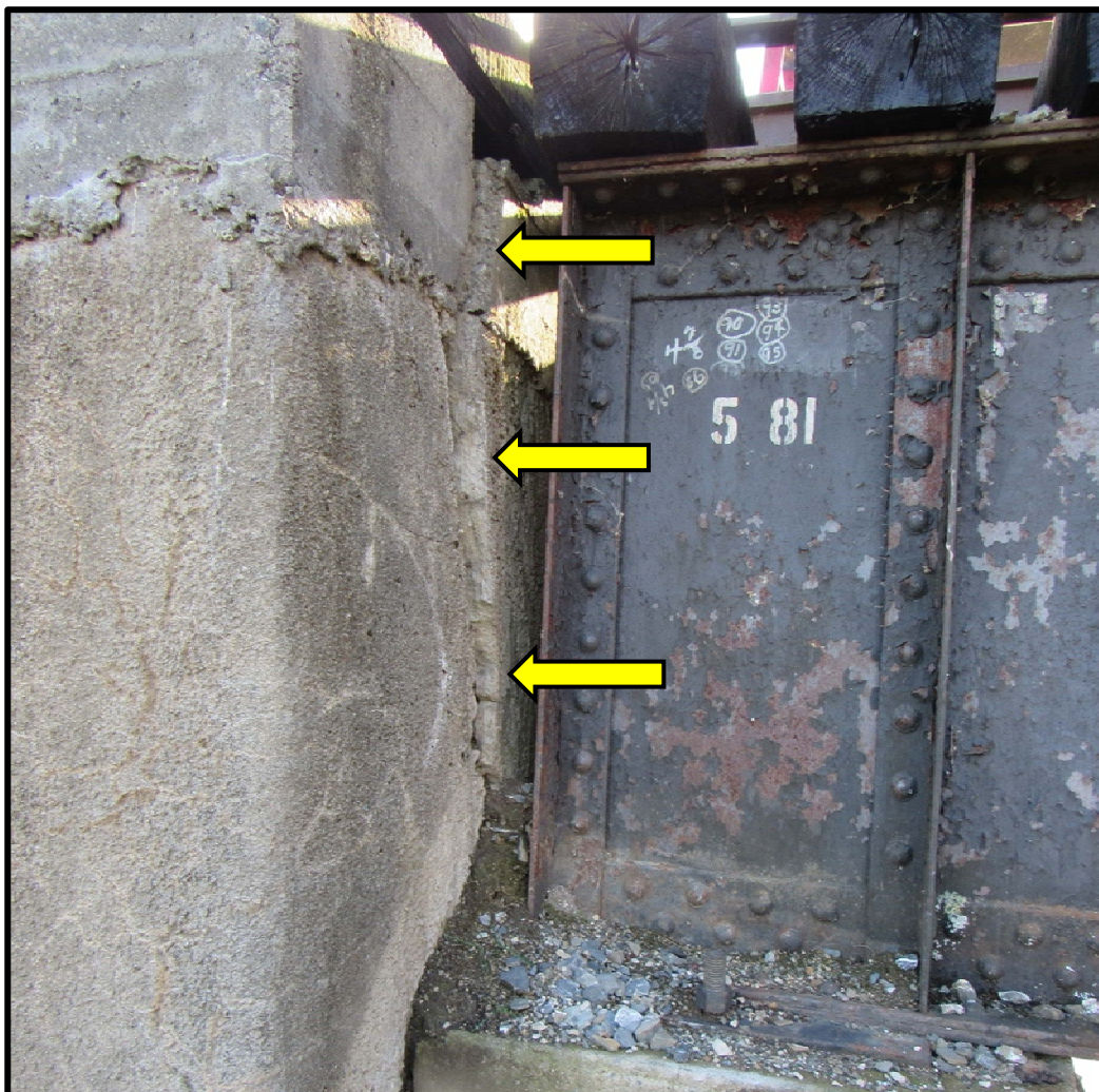
Full-Height Crack with Ballast Spilling Thru and Backwall Tipping Forward on the East Abutment
