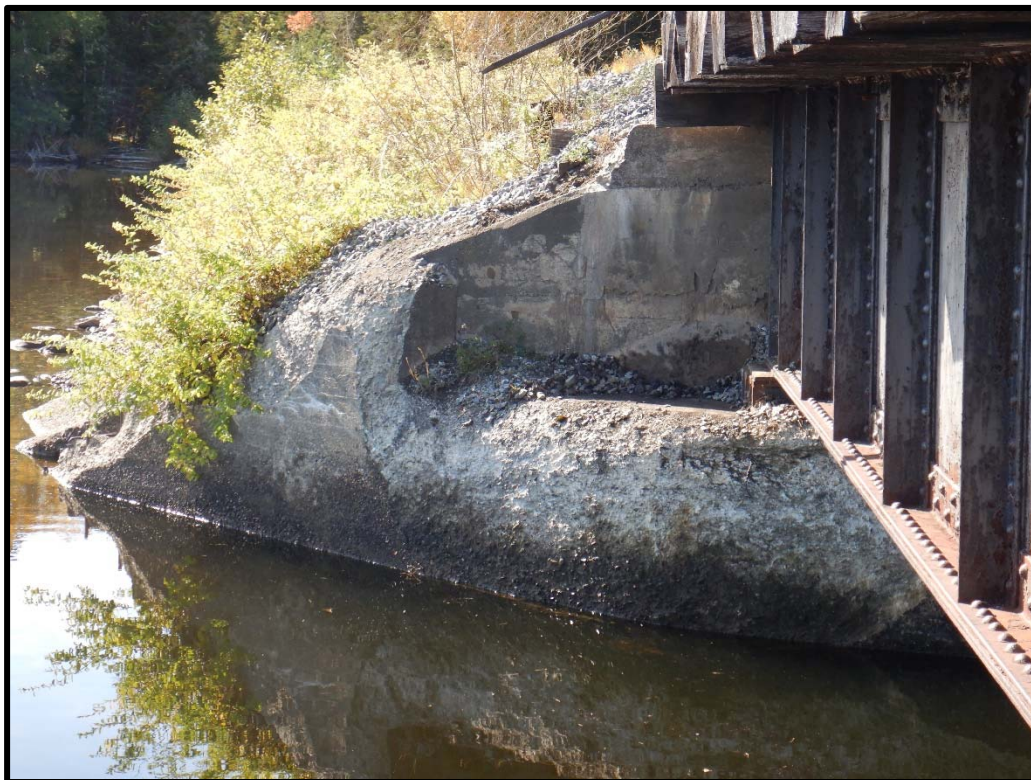
Heavy Deterioration on the Southwest Corner of Bridge Seat and Wingwall
