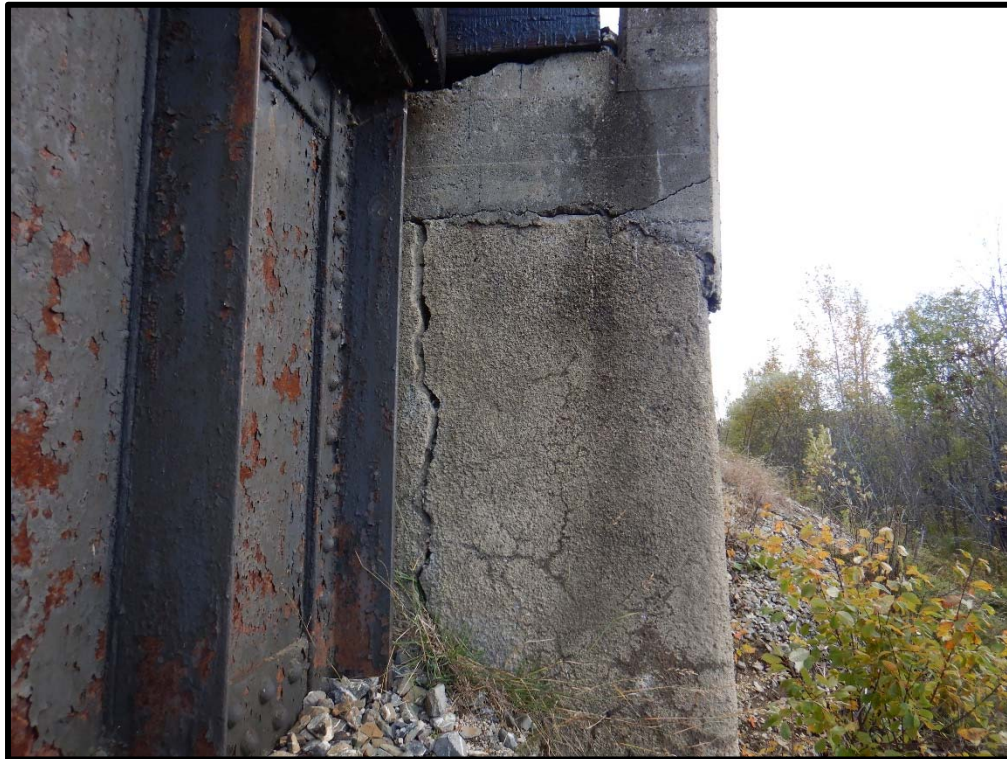
Half Inch Full-Height Crack in Backwall of East Abutment
