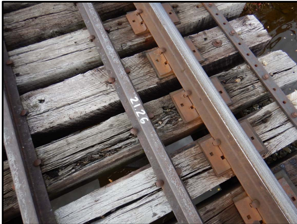
Bridge Timbers in Poor Condition
