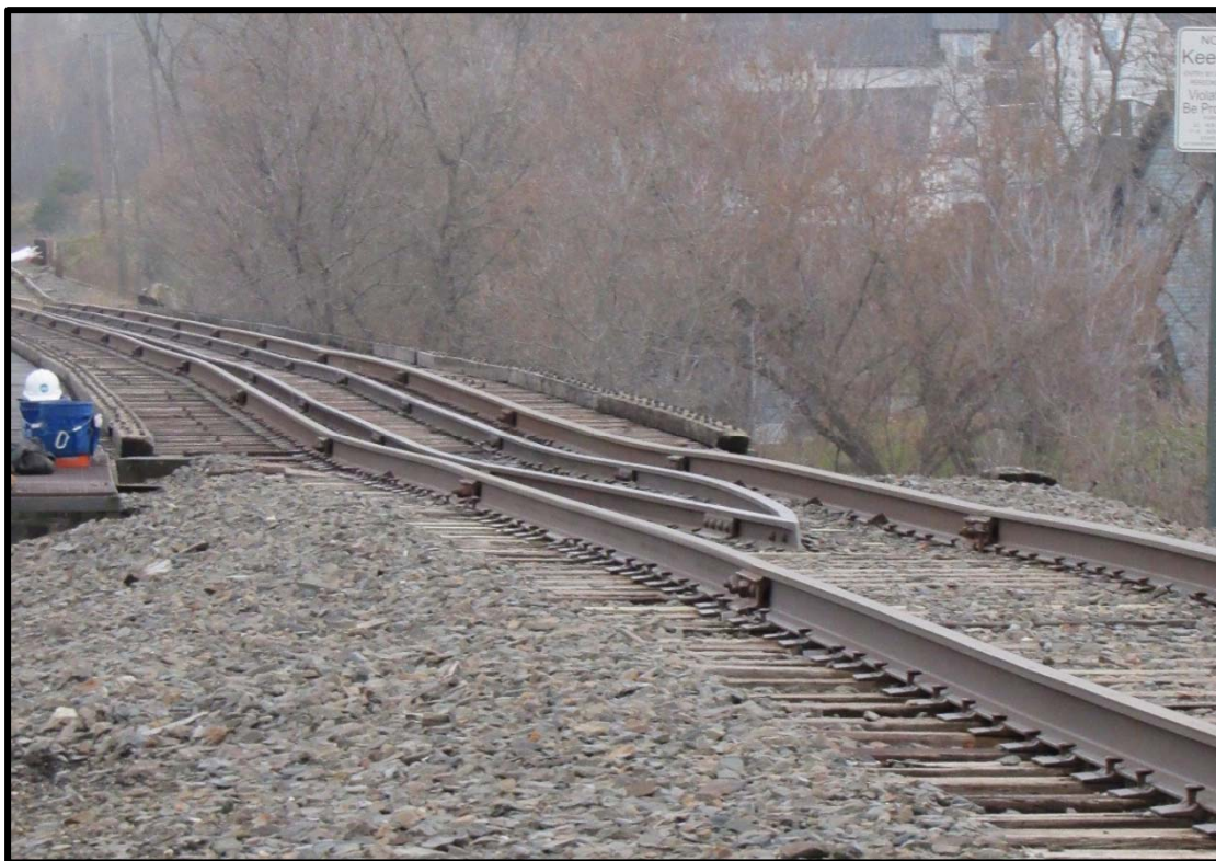
Settlement in Approach Track Just Prior to South Abutment (Looking North)
