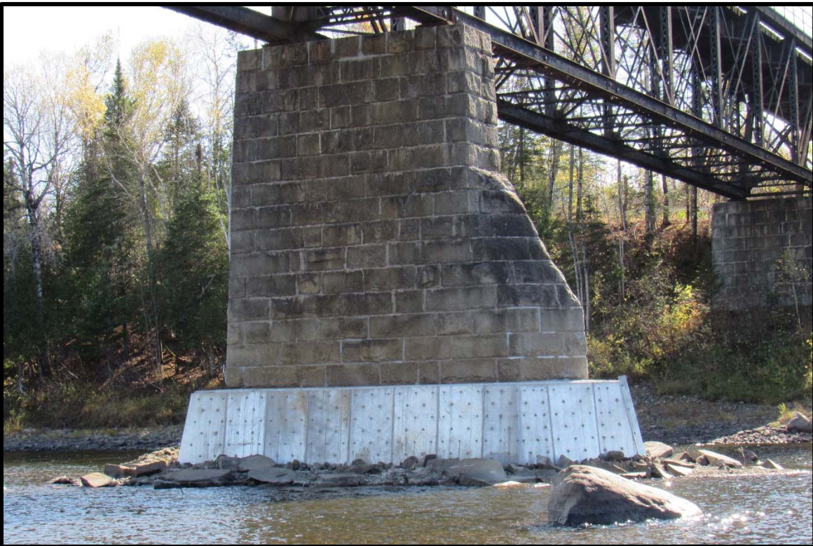
Sample – Steel Plated Footing Apron Repair on Sheridan Truss in Ashland on Madawaska Subdivision
