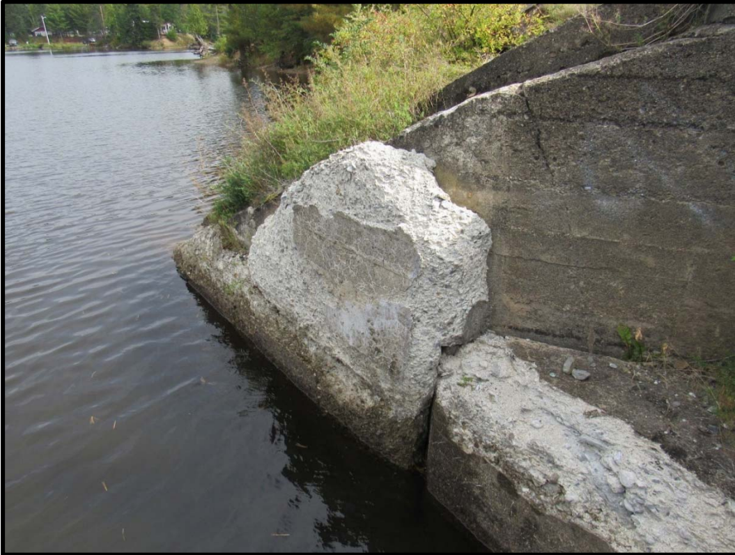
Heavy Deterioration and Cracking at Northeast Corner of Bridge Seat and Wingwall
