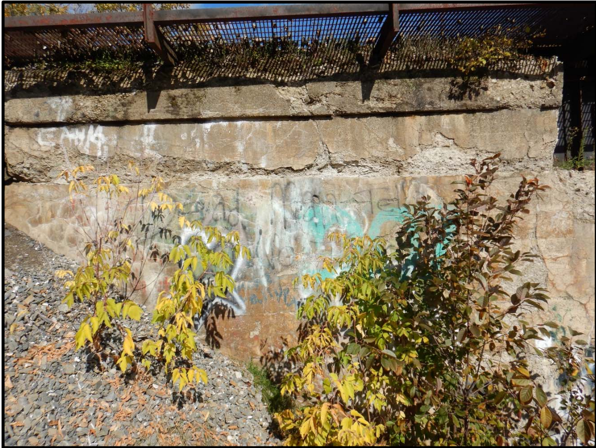
Deteriorated and Delaminated Concrete Along the Upper Portion of the Southwest Wingwall
