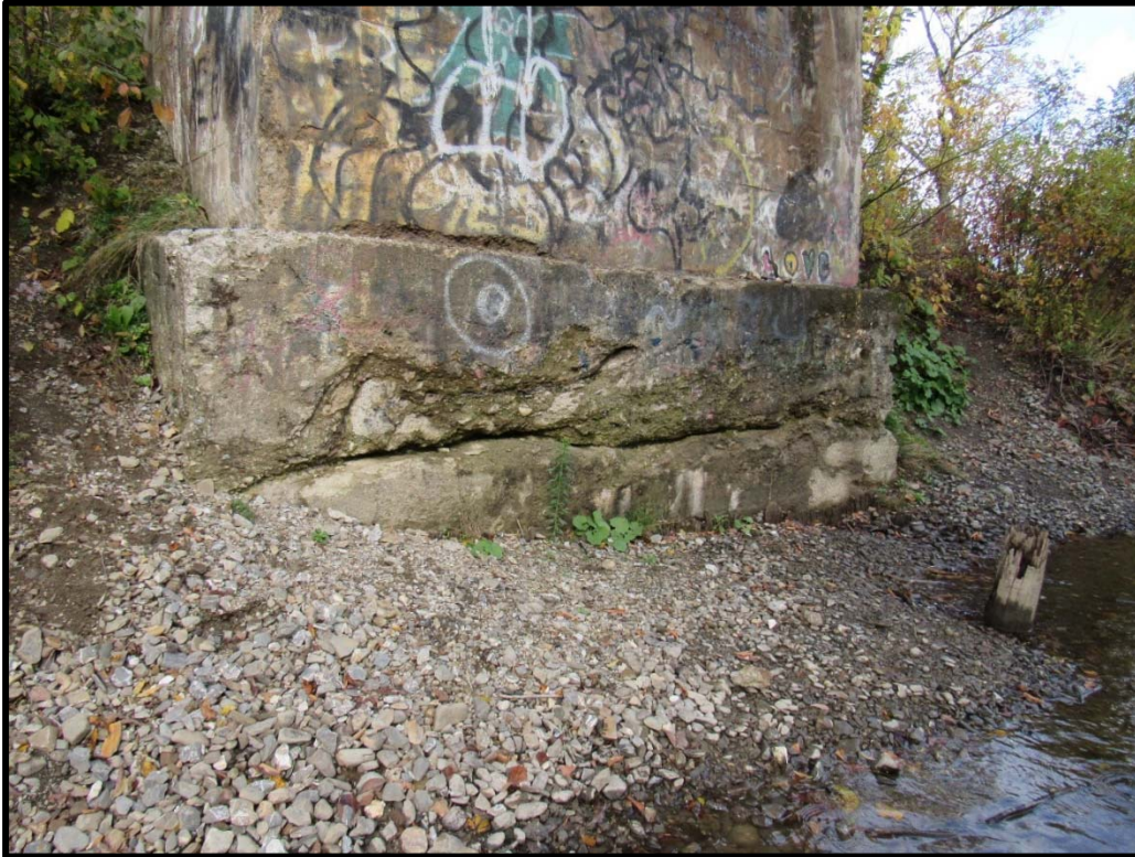
Heavy Deterioration and Abrasion on the Base of the West (Track South) Abutment
