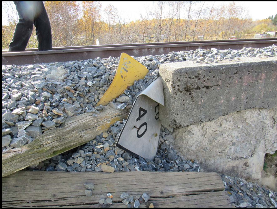
Failed Ballast Retainer behind the East Abutment
