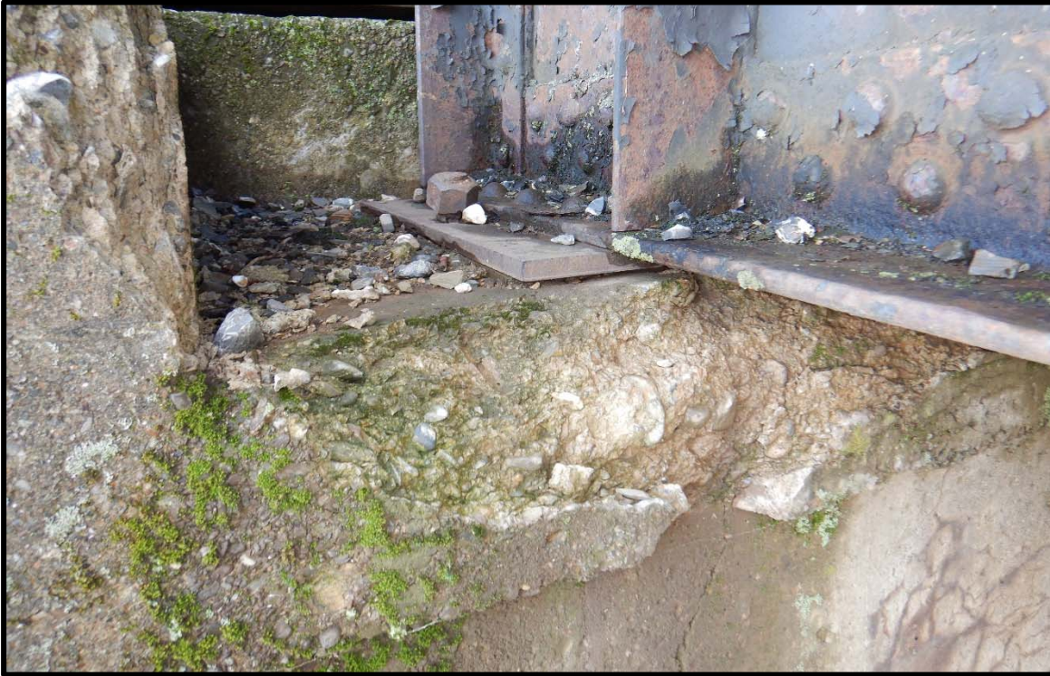
Bent/Corroded Anchor Bolts and Deteriorated Concrete on Bridge Seat of East (Track North) Pier
