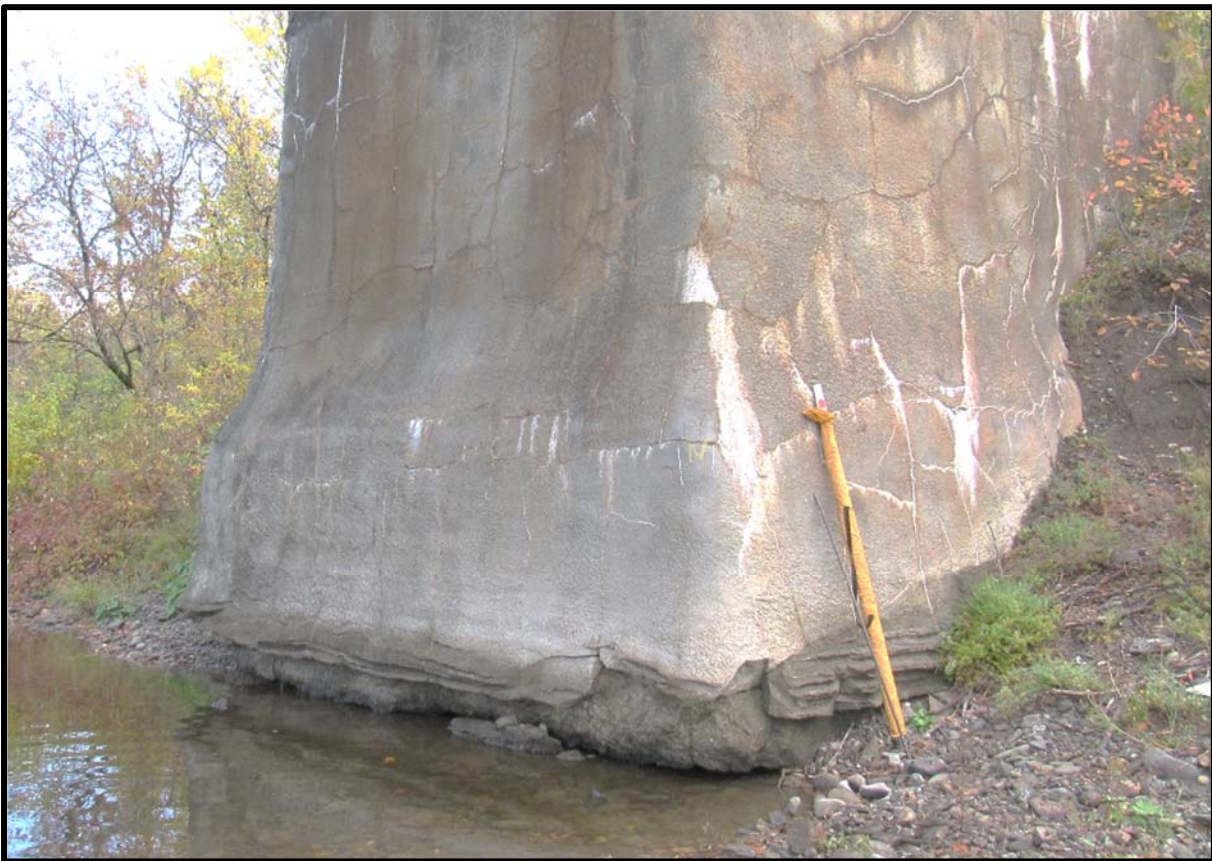
Abraded and Deteriorated Concrete Along the Base of the East (Track North) Abutment
