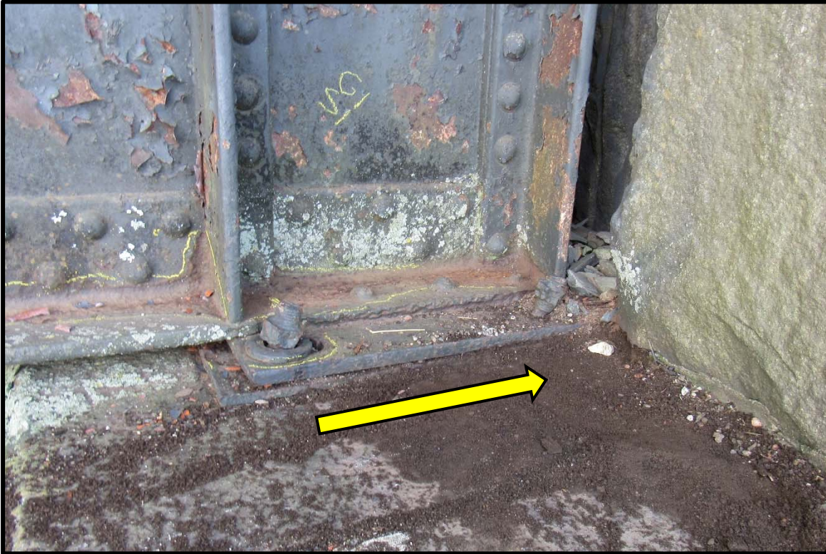
At South Abutment, Anchor Bolts Bent and Bearing Plates Overextended Towards Backwall
