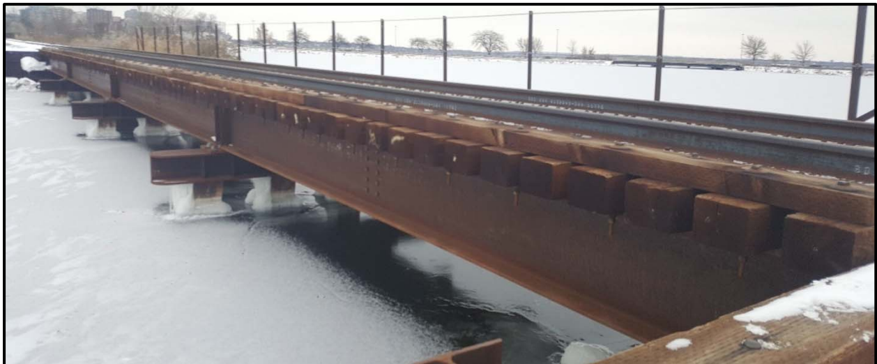
2017 Construction: Steel Girders on Steel Pile Bents on Wisconsin Southern Railroad (WSOR)- Madison WI
