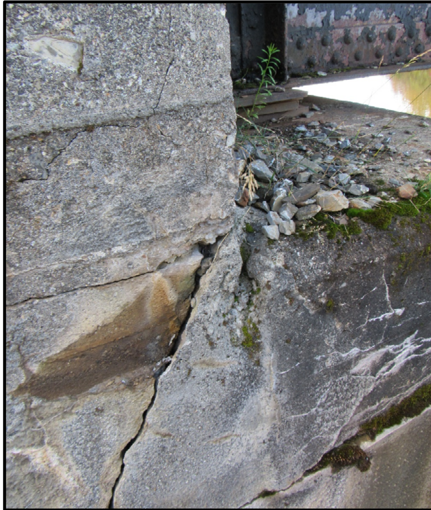
Cracking at Backwall and Wingwall Interface on East (Track North) Abutment
