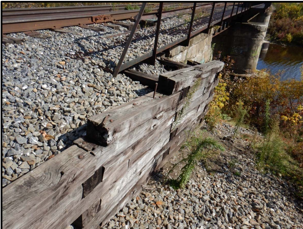
Failed Ballast Retainer behind the Southwest Wingwall
