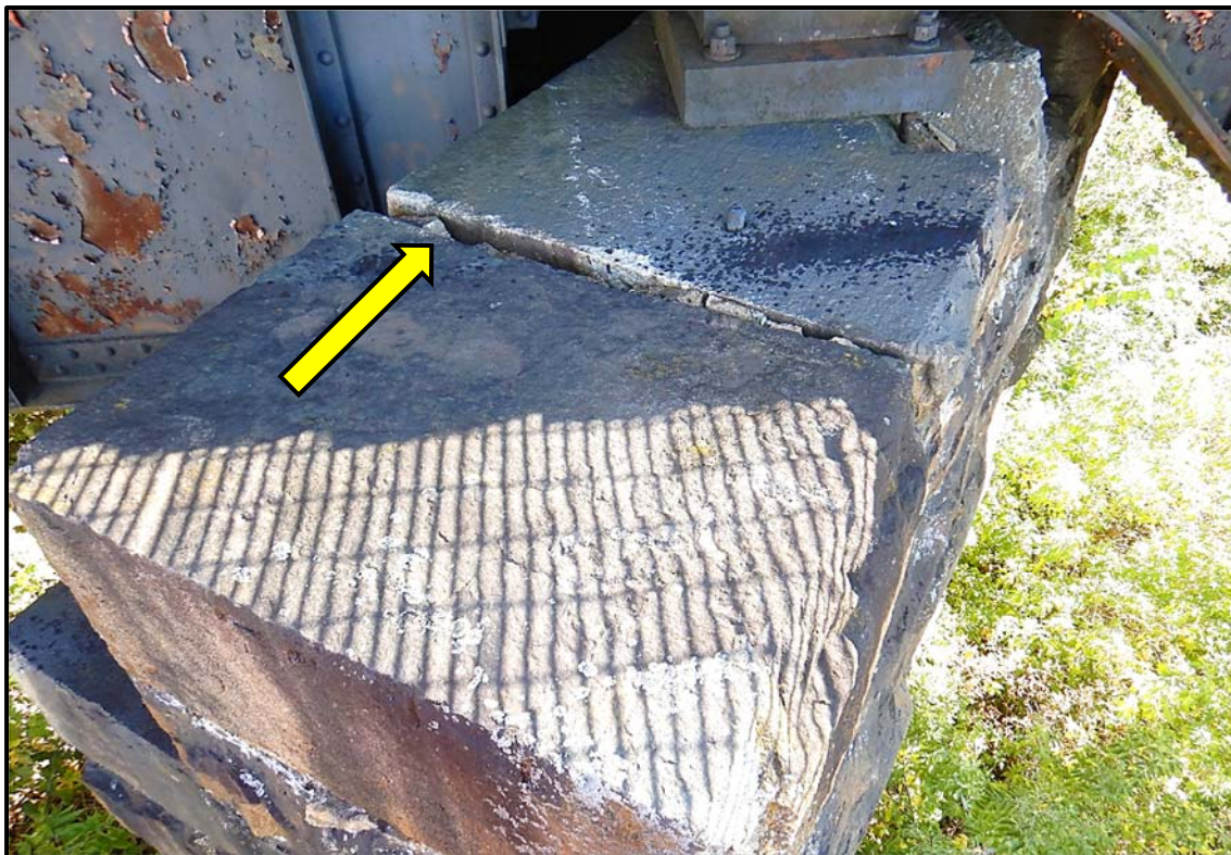
Blocks Shifting and Joint Opened on Top of Pier 4 on the West End
