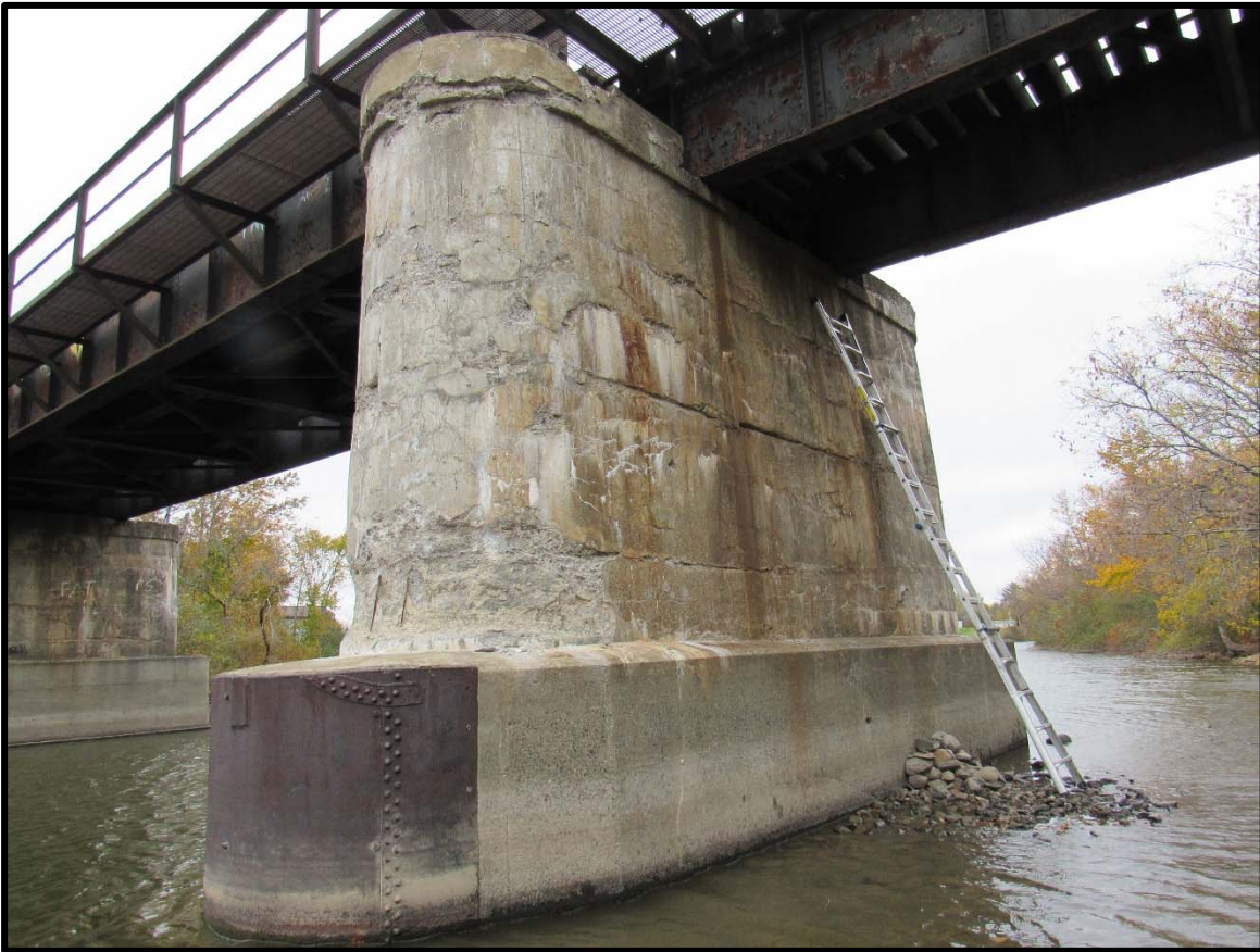
Heavy Spalling and Delaminations on Upstream End of the East (Track North) Pier
