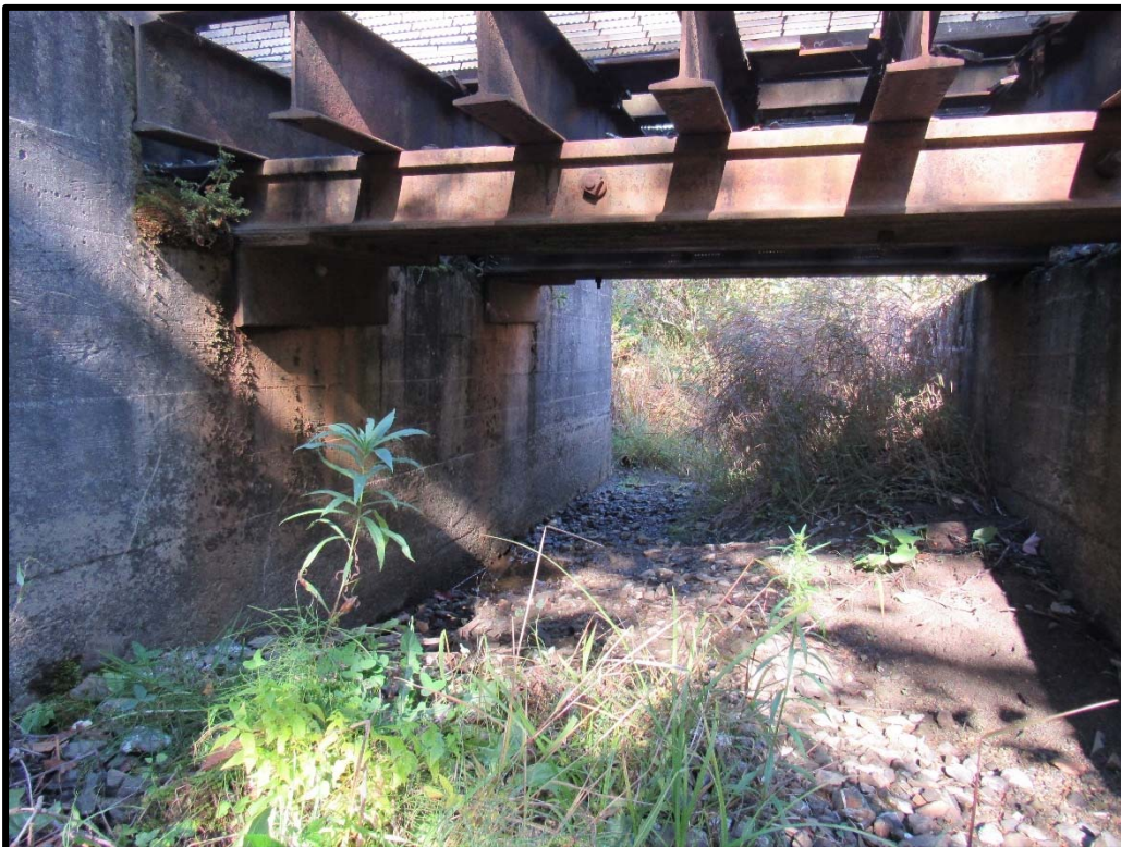
South Span Heavily Silted, Filled With Debris and Dry
