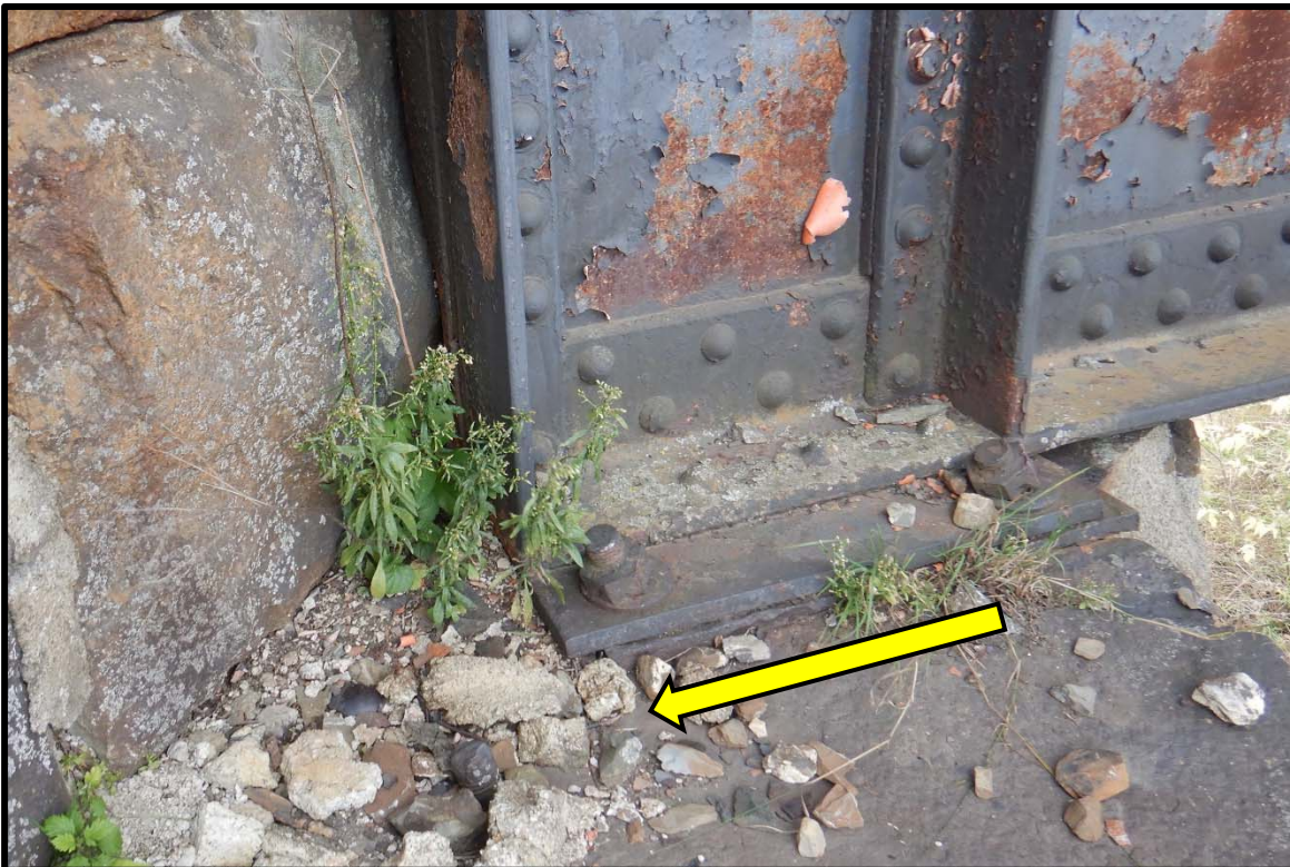
At Pier 1, Anchor Bolts Bent and Bearing Plates Overextended Away from the South Abutment
