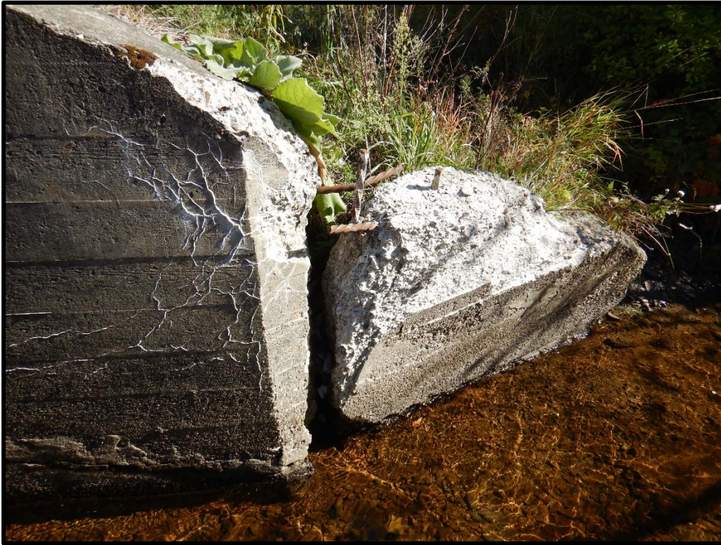
Northeast Wingwall Completely Detached From Breastwall and Tipping Forward
