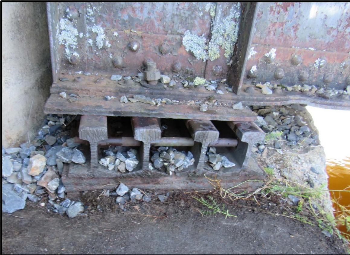
Girder Shifted Three Inches Laterally at the Northeast Bearing Due to Failed Anchor Bolts
