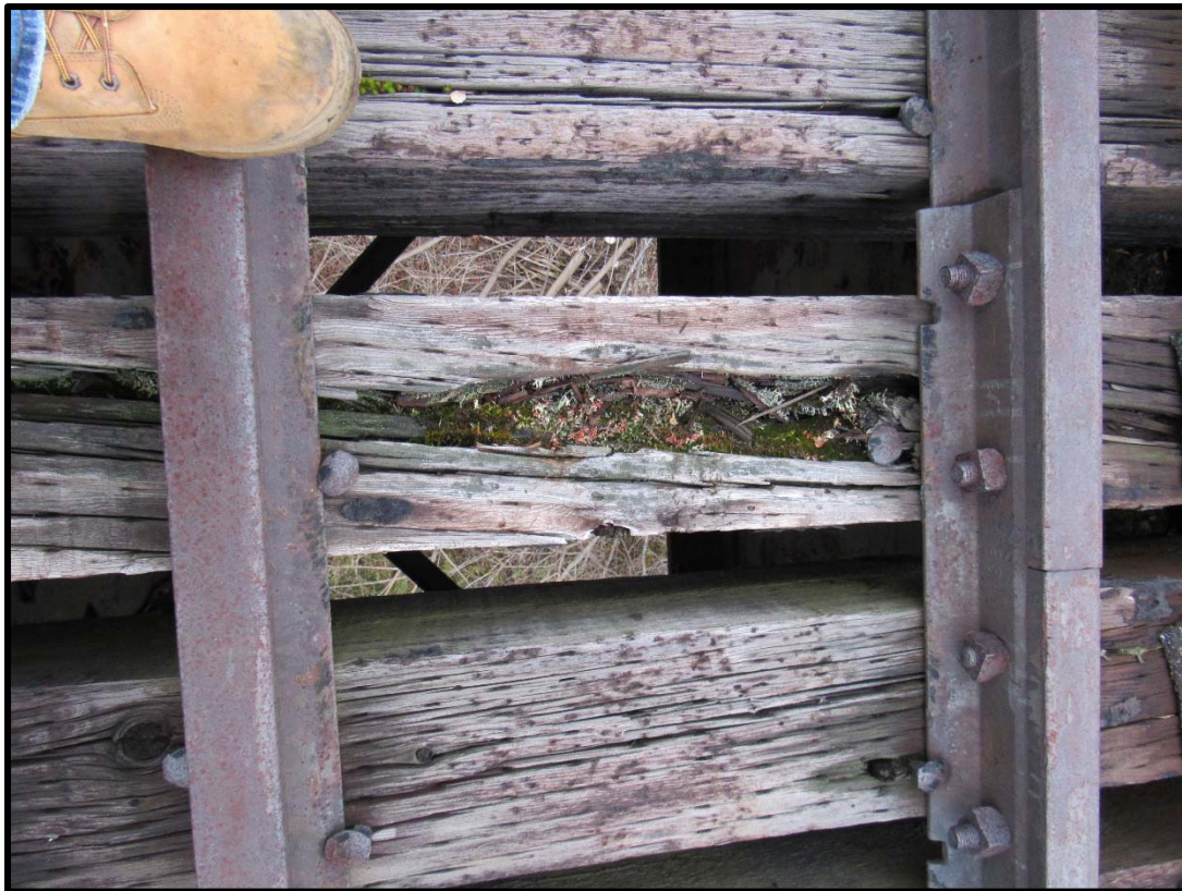
Bridge Timber in Serious Condition, Multiple Other Timbers in Similar Condition
