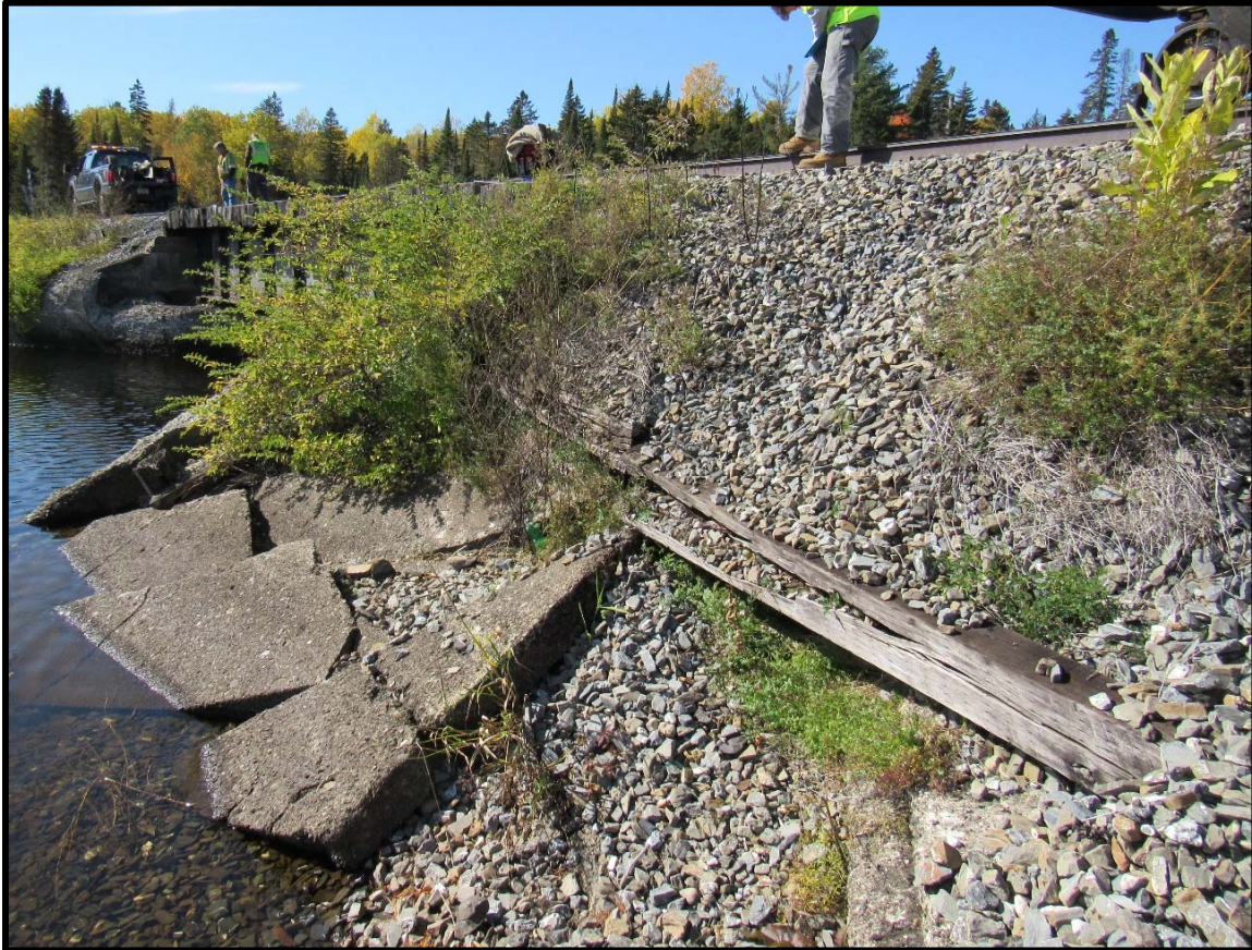
Failed Slope Protection Behind Southeast Wingwall
