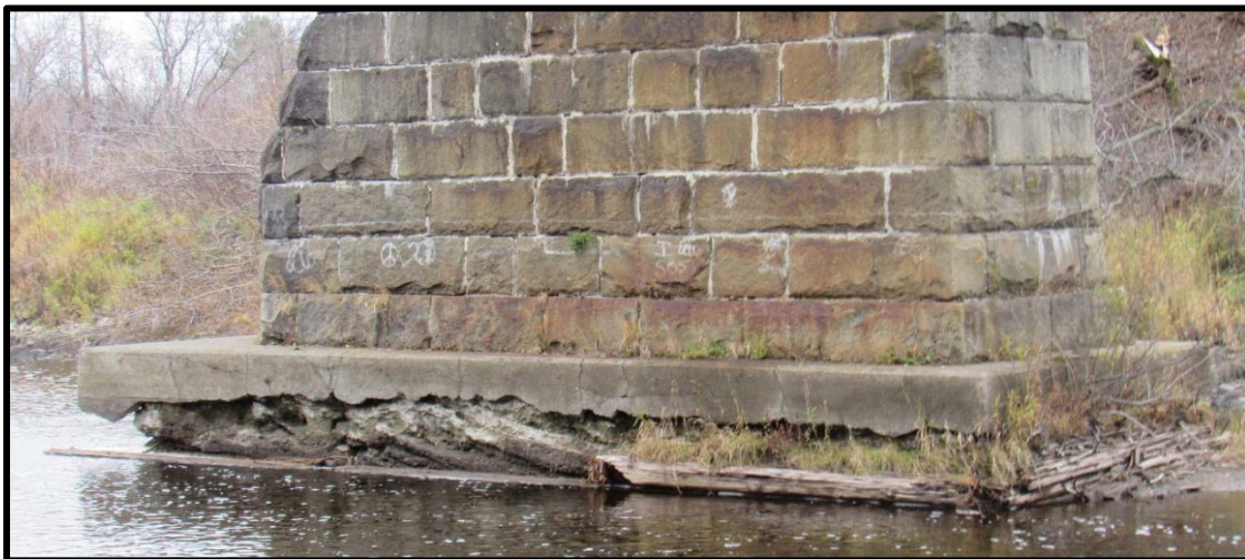
Heavy Deterioration and Undermining on South End of Pier 3 Footing Apron
