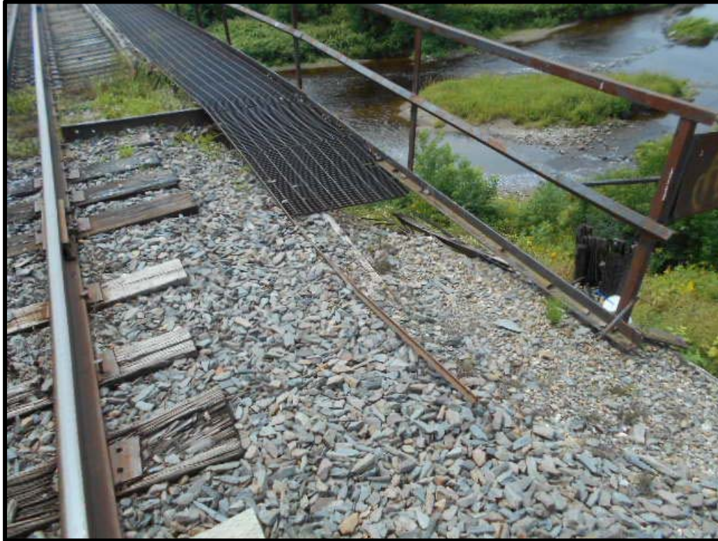
Damaged Walkway Section at North End of Bridge
