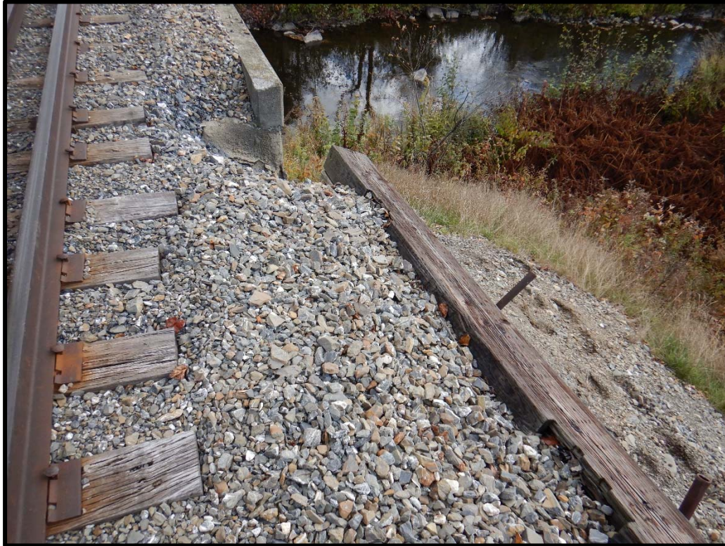
Failed Ballast Retainer Behind the West Abutment
