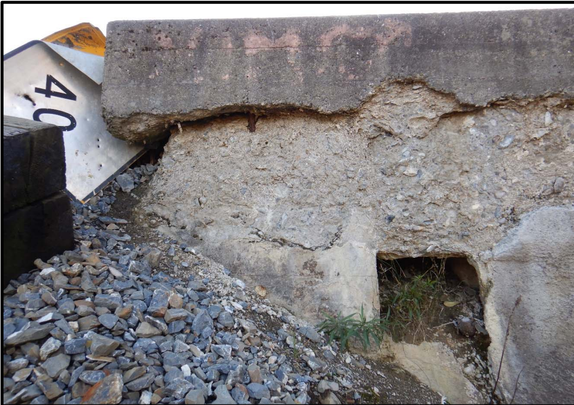
Deteriorated Concrete and Hole in the Northeast Wingwall
