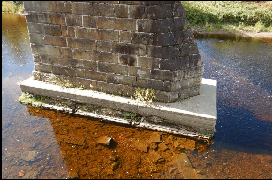
Heavy Deterioration and Undermining on South End of Pier 3 Footing Apron
