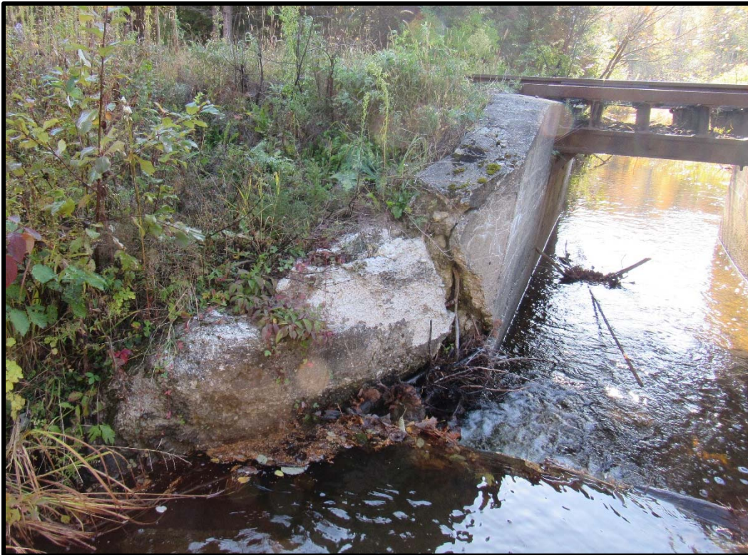
Northwest Wingwall Heavily Deteriorated and Cracked, North Abutment Tipping Forward
