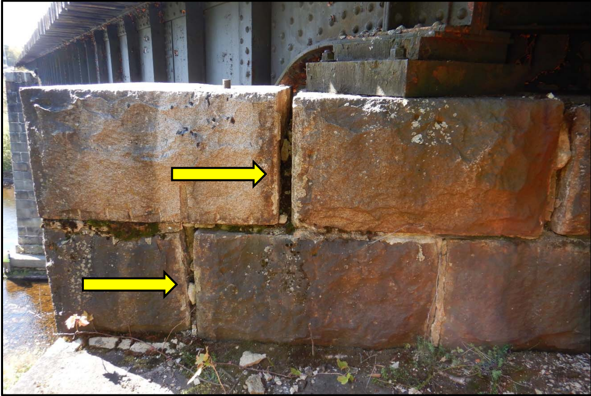
Blocks Shifting and Joints Open Up on the East Corner of the North Face of Pier 4
