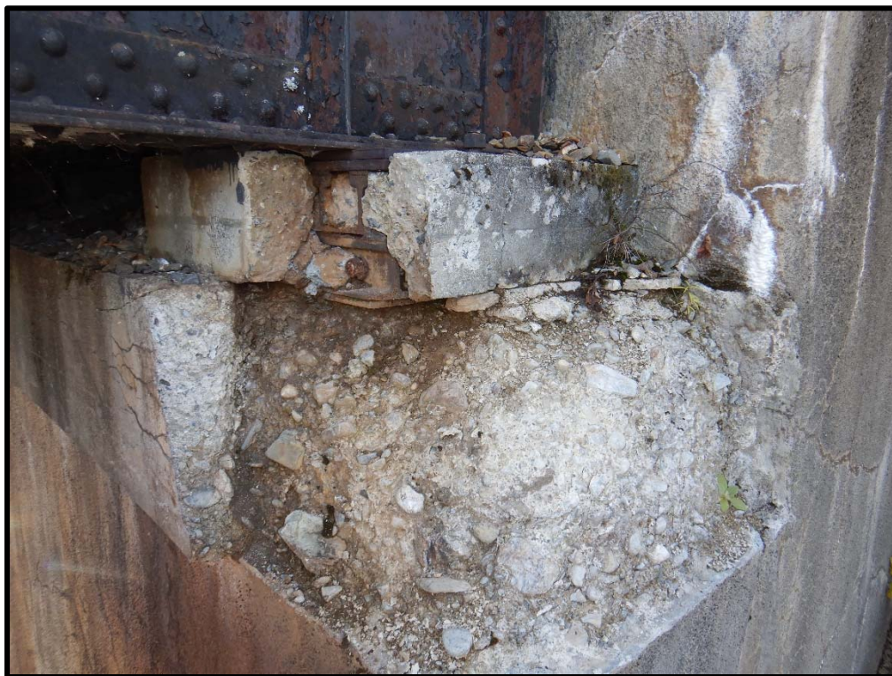
Coping Along Face of Bridge Seat Heavily Deteriorated at West Abutment
