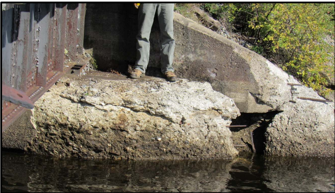
Heavy Deterioration and Large Hole at Southeast Corner of Bridge Seat and Wingwall
