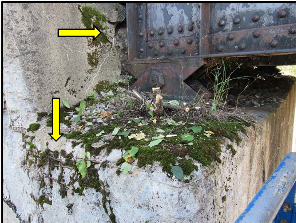
Deterioration in Bridge Seat and Backwall at Northwest Bearing
