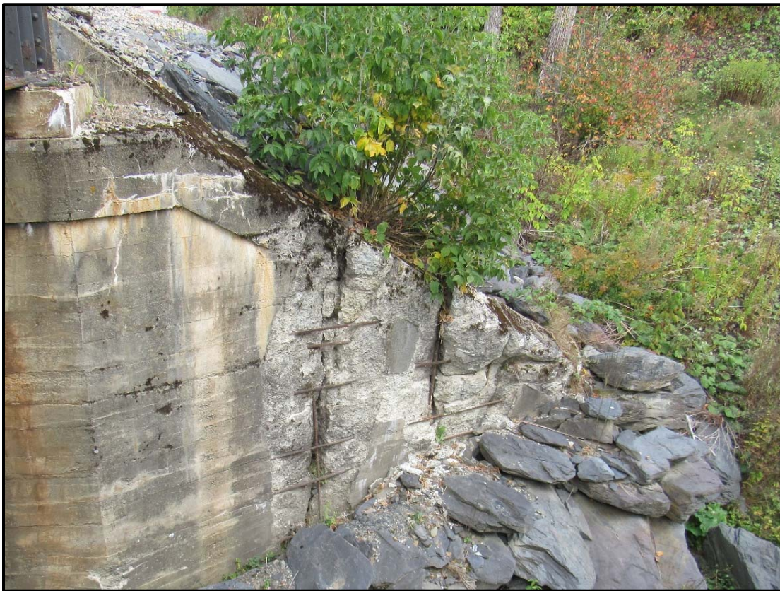
Heavy Deterioration and Cracking at the Northeast Wingwall
