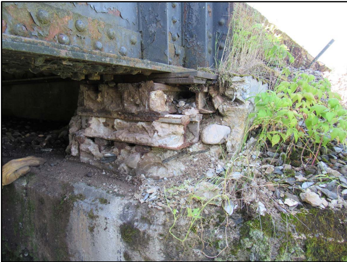
Deteriorated Concrete Around Grillage at Southwest Bearing
