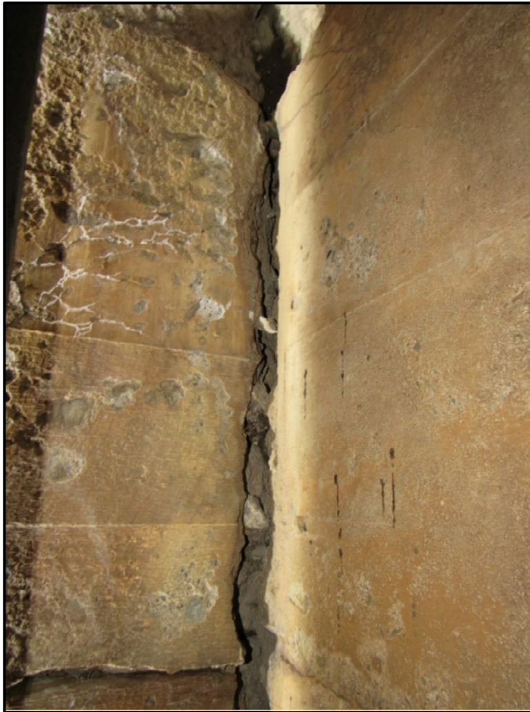
Crack in North Abutment at End of the East Girder, Up to 2" Wide
