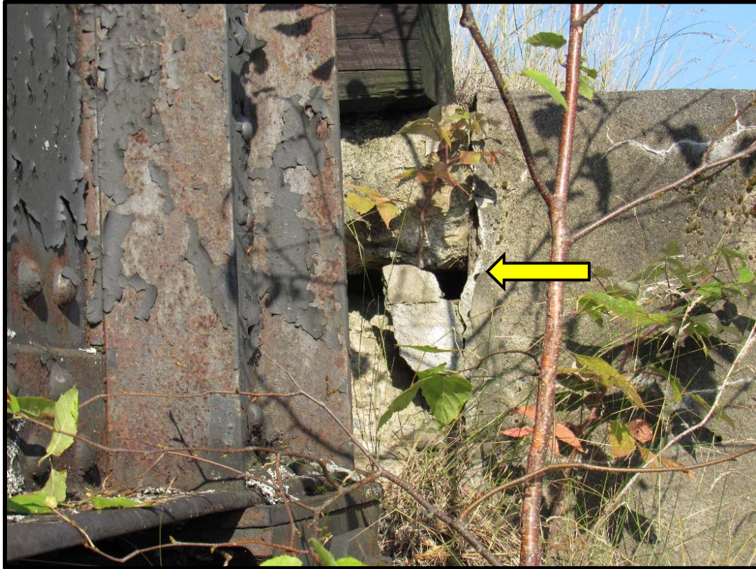
Deteriorated and Crumbling Concrete Backwall at Northeast Bearing
