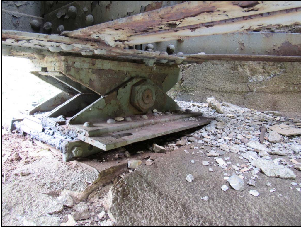
Failed Expansion Bearing at North Abutment
