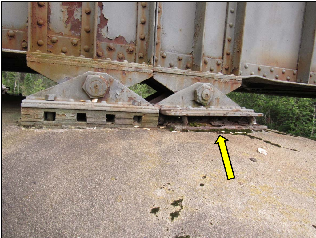
Failed Expansion Bearing on Southwest Side of Pier
