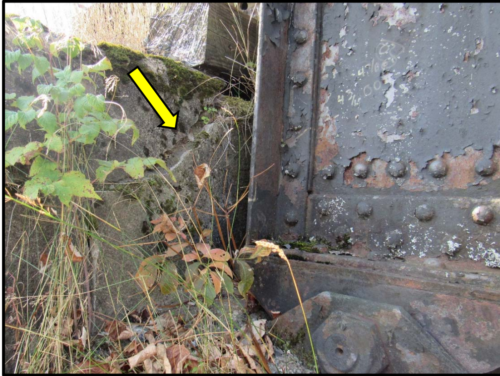
Crack in Backwall at Southeast Bearing
