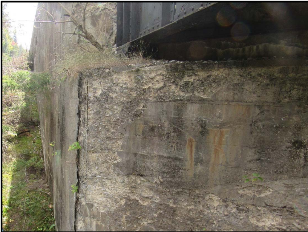
Heavy Deterioration in Bridge Seat at South Abutment
