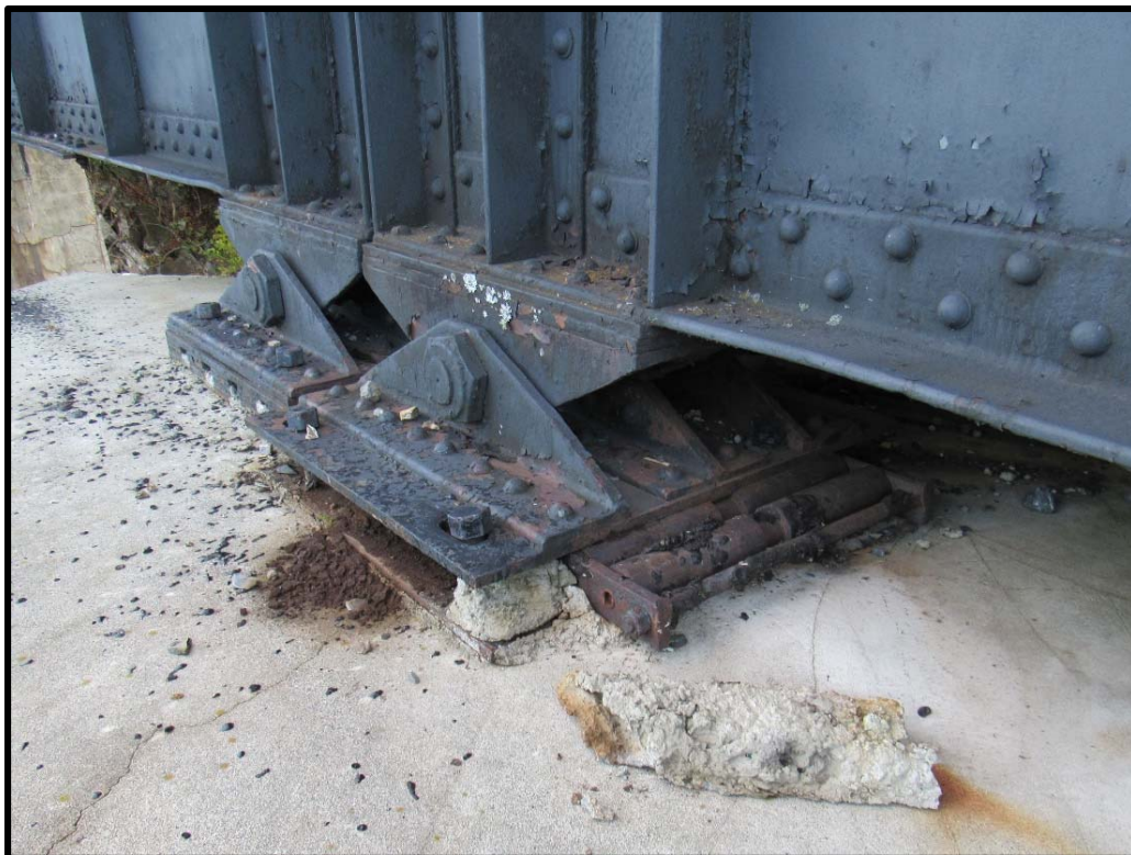
Failed Expansion Bearing at North Pier
