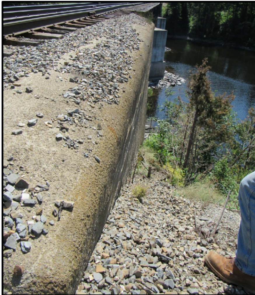
Northwest Wingwall Tilting Outward (Originally Battered Inward)
