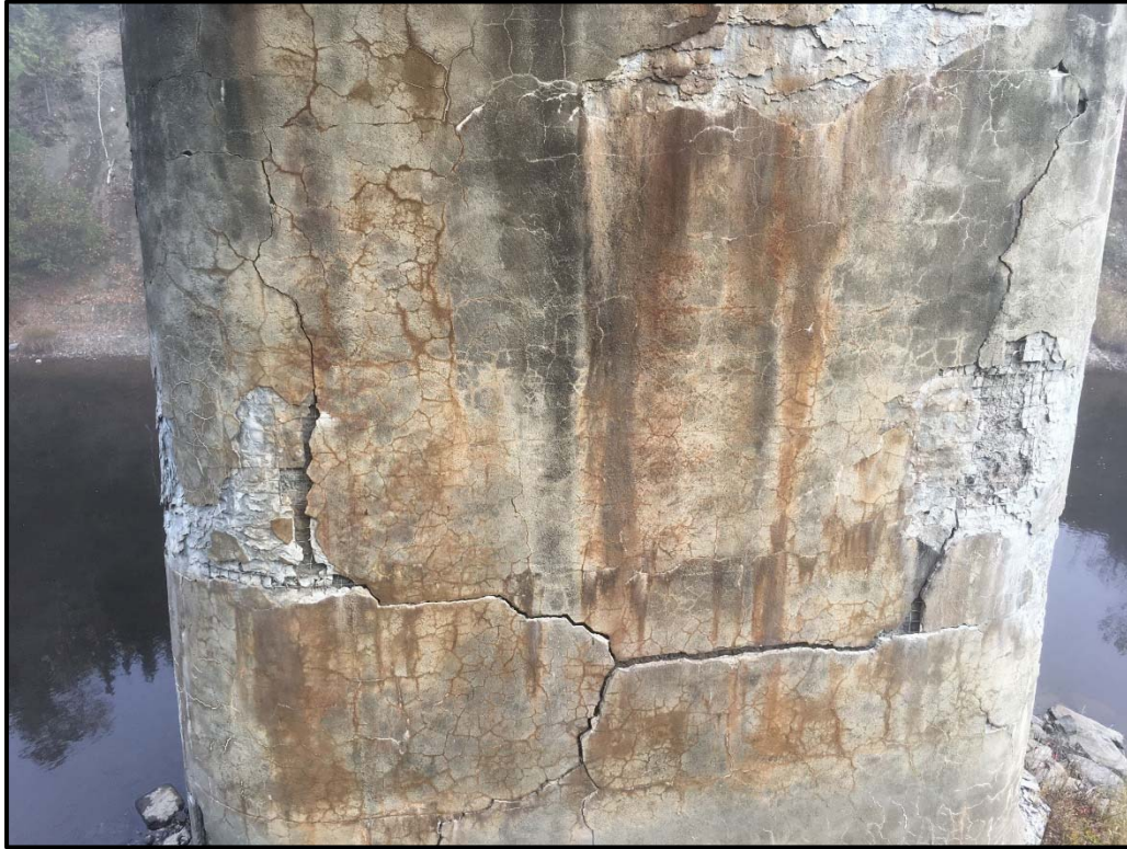
Delamination and Cracking on the South Face of Pier
