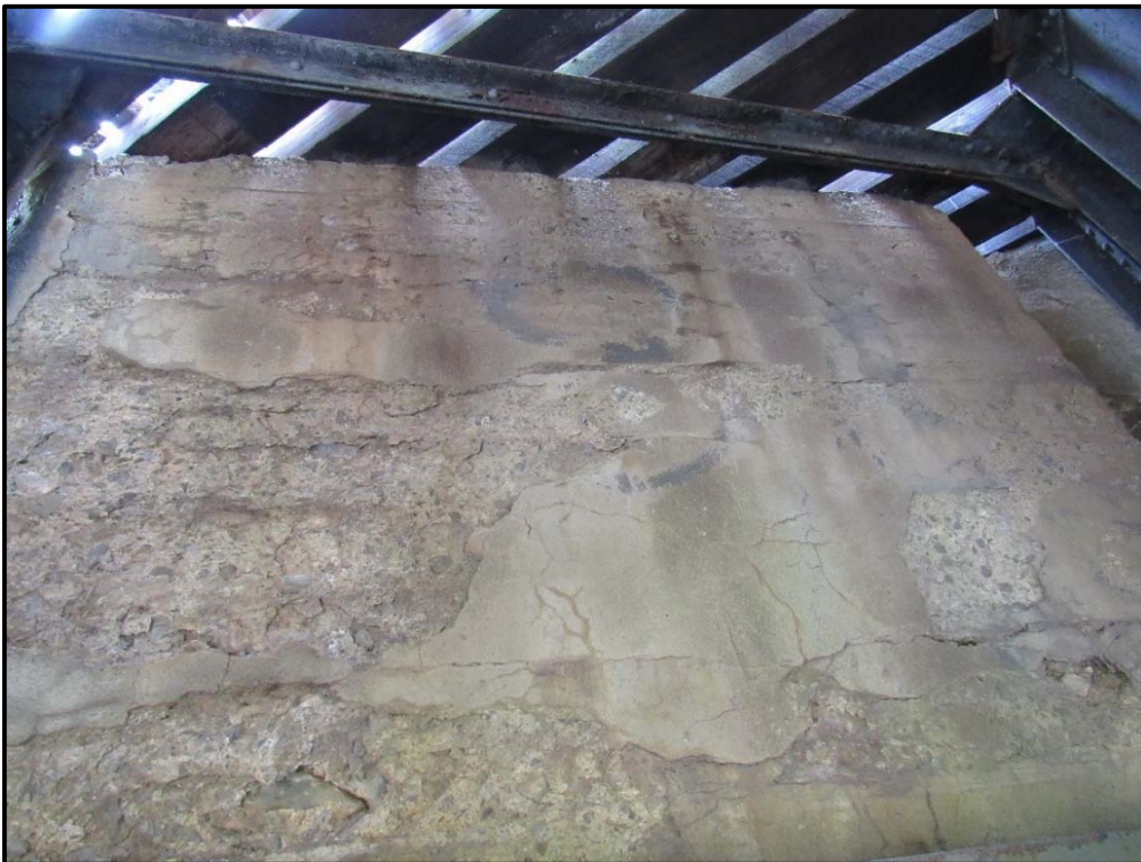
Spalled and Deteriorated Concrete in the Backwall of the South Abutment
