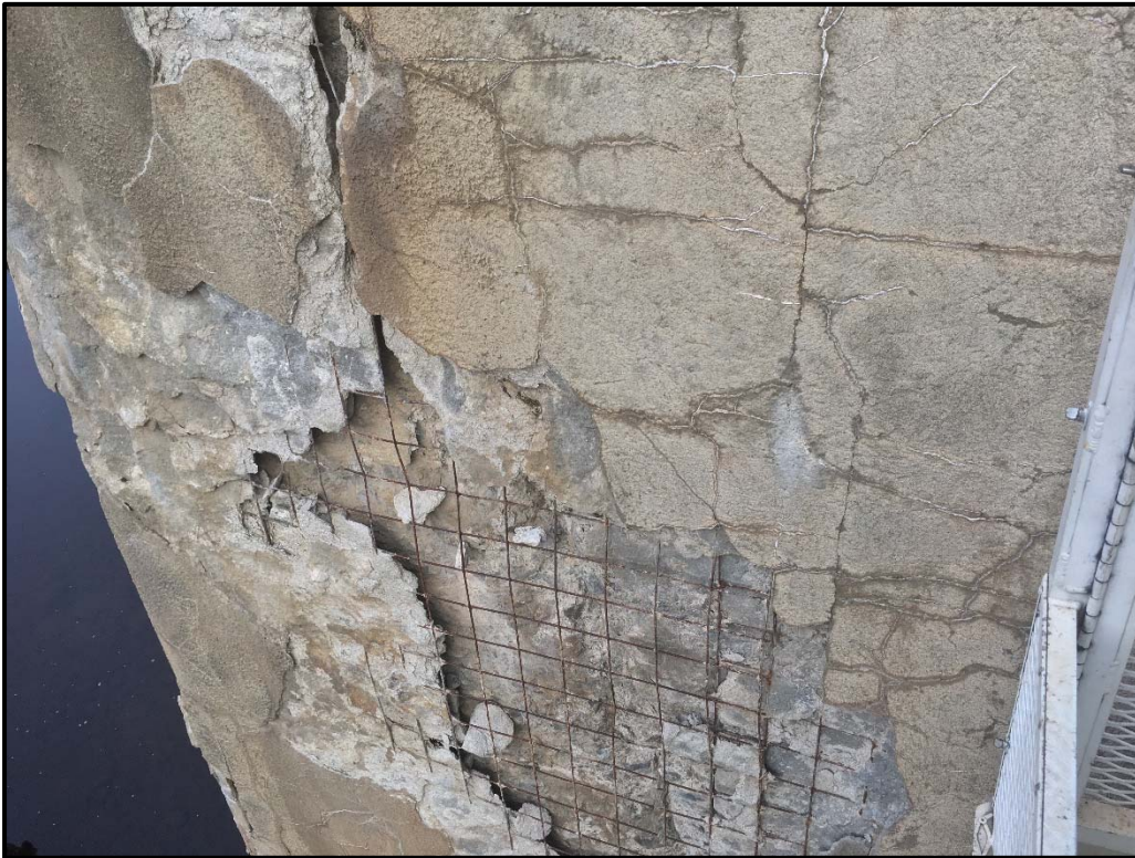
Heavy Delamination on the South East Corner of Pier
