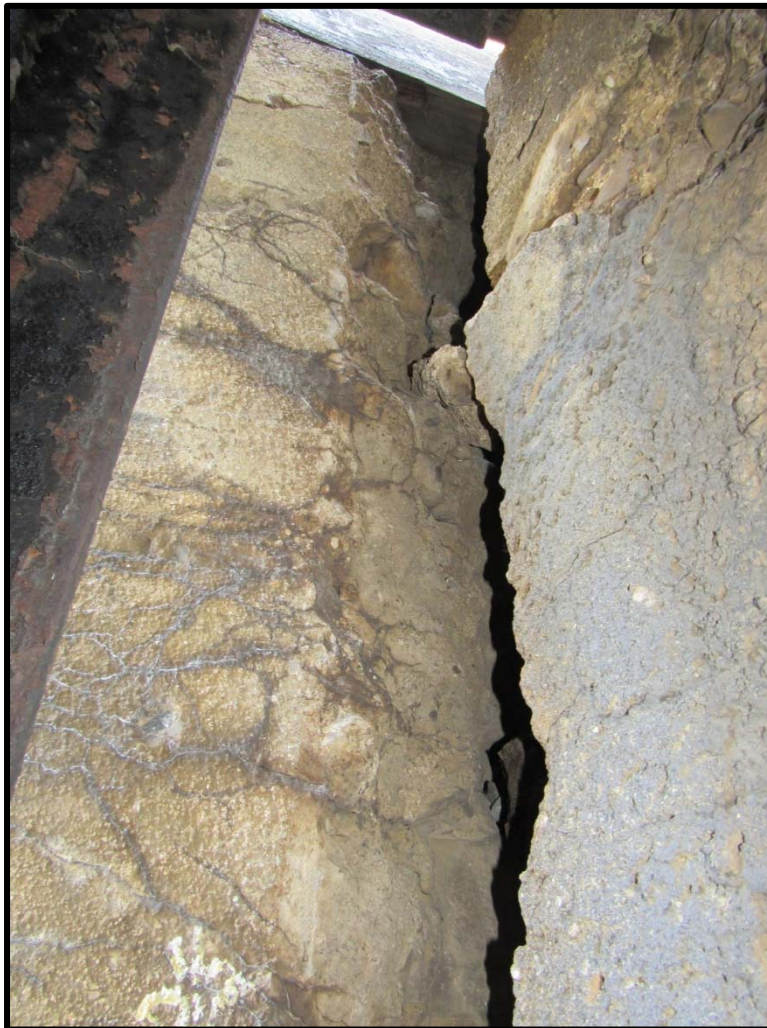
Crack in North Abutment at End of the West Girder, Up to 3" Wide
