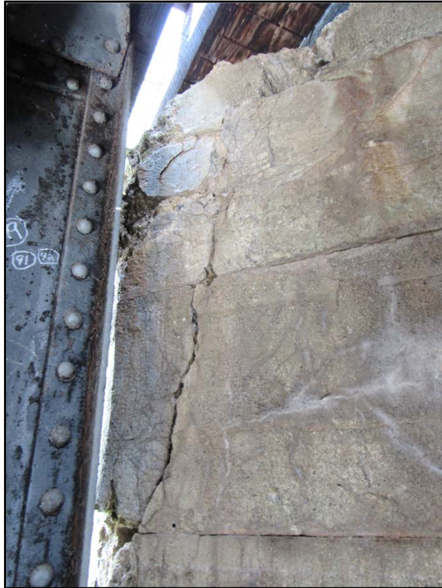
Diagonal Shear Crack in the Upper West Corner of the North Abutment Backwall Under Bridge Timber
