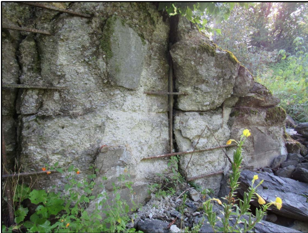
Heavy Deterioration and Cracks at the Northeast Wingwall
