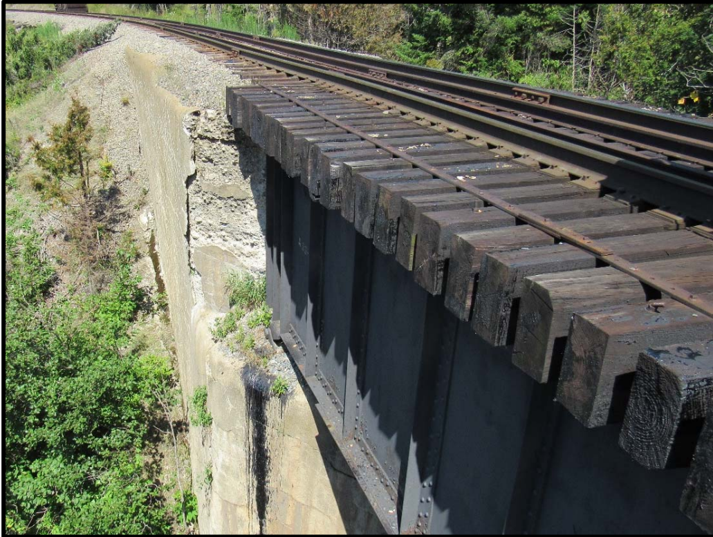
Heavy Deterioration at the Interface of Northwest Wingwall and Backwall
