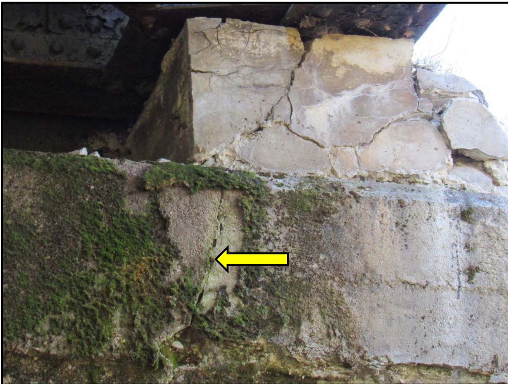
Cracking in Bridge Seat Directly Under Southwest Bearing
