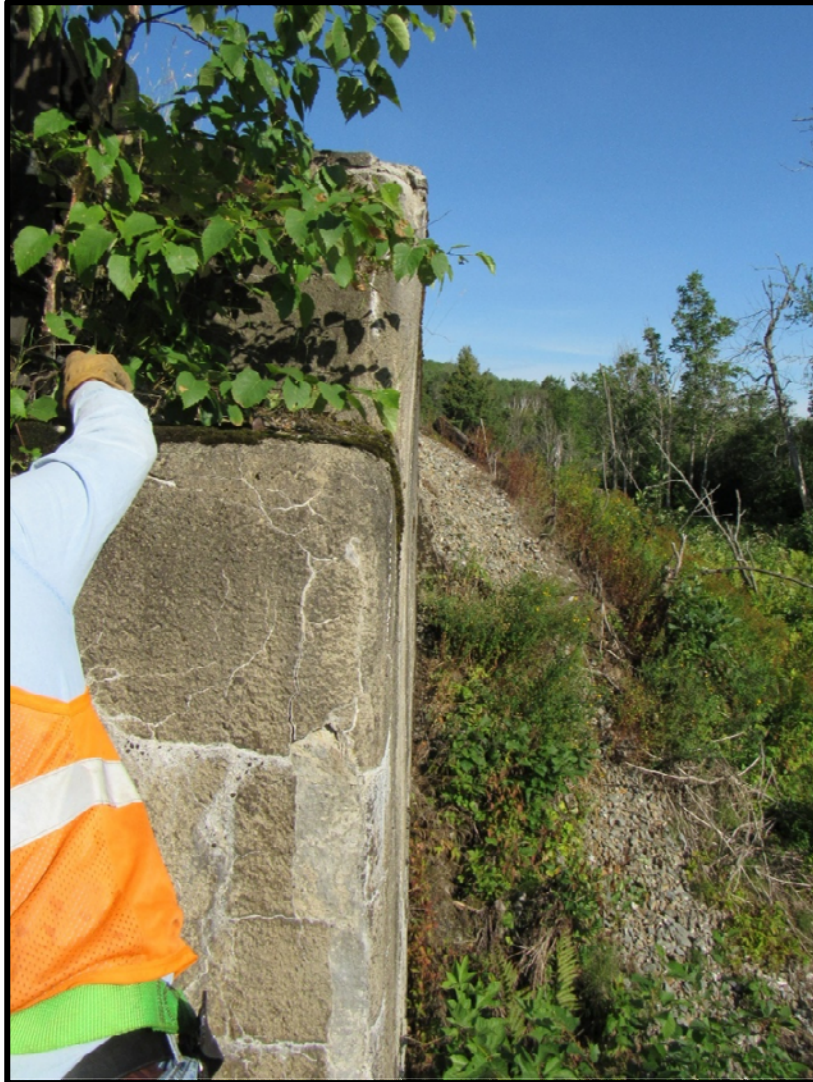
Northeast Wingwall Tilting Outward (Originally Battered)
