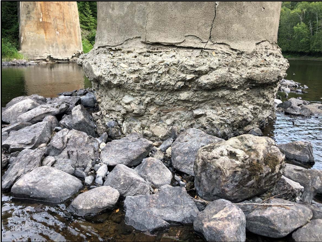
Deteriorated Concrete at Base of Pier
