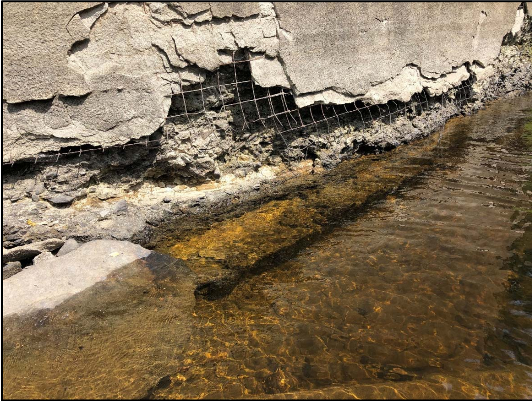
Deteriorated and Abraded Concrete at Base of North Abutment
