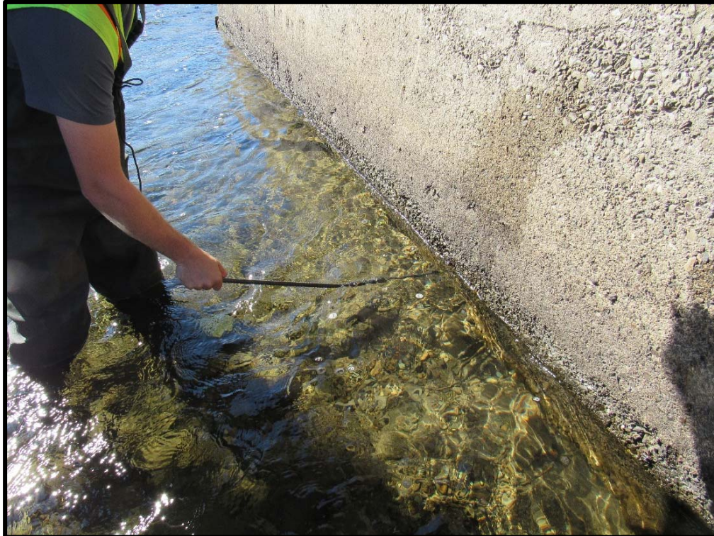
Gap Between the Bottom of the Concrete Encasement and the River Bed, at North Abutment
