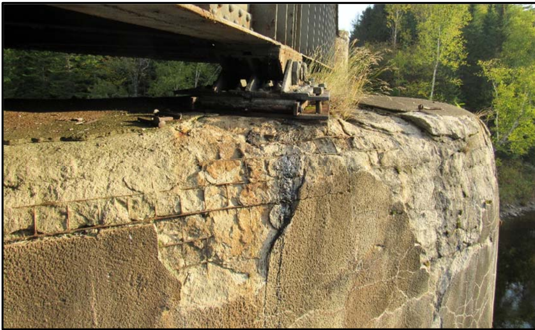
Heavily Deteriorated Concrete and Undermined Bearing at Top of Pier
