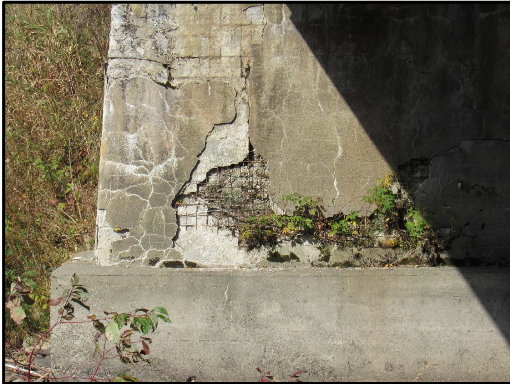
Heavy Deterioration in Shotcrete on North Abutment
