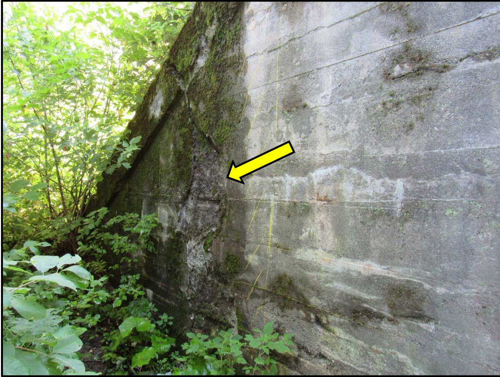
Spalled, Deteriorated, and Cracked Area at the Northwest Wingwall
