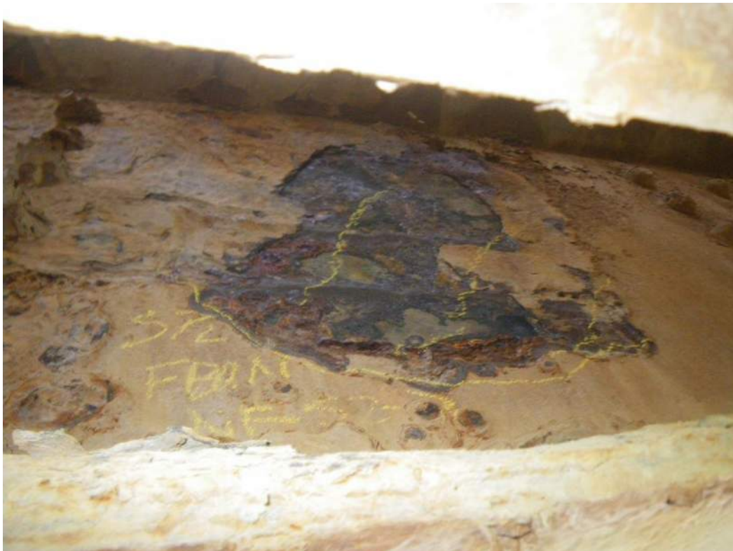
Photo 42: Floorbeam FB0N between Stringers S2 and S3, North Face, Span 2 - Web section loss. Note failed paint system.
