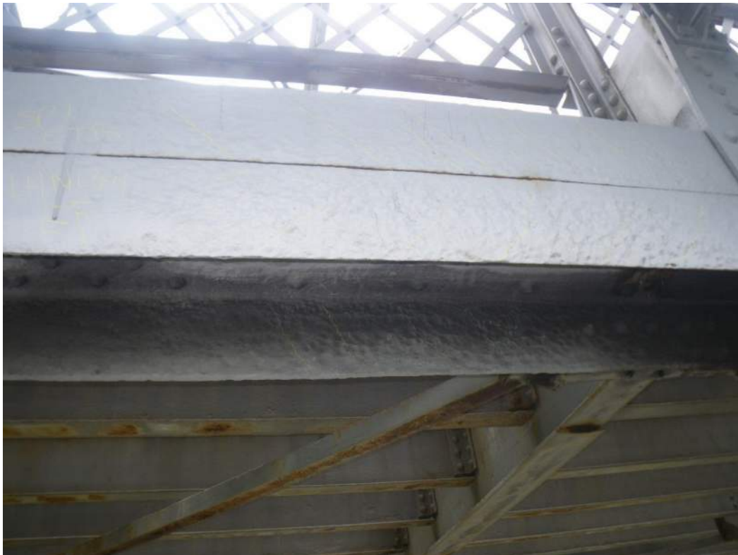
Photo 54: Lower Chord L3NL4N at 2'-0" from Panel Point L3N, East Face, East Truss, Span 1 - Section loss of all flange angles.
