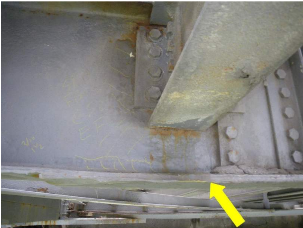
Photo 46: Floorbeam FB1S at Stringer S2, North Face, Span 4 - Web and bottom flange section loss adjacent to/below stringer connection. Note rust forming under paint system.
