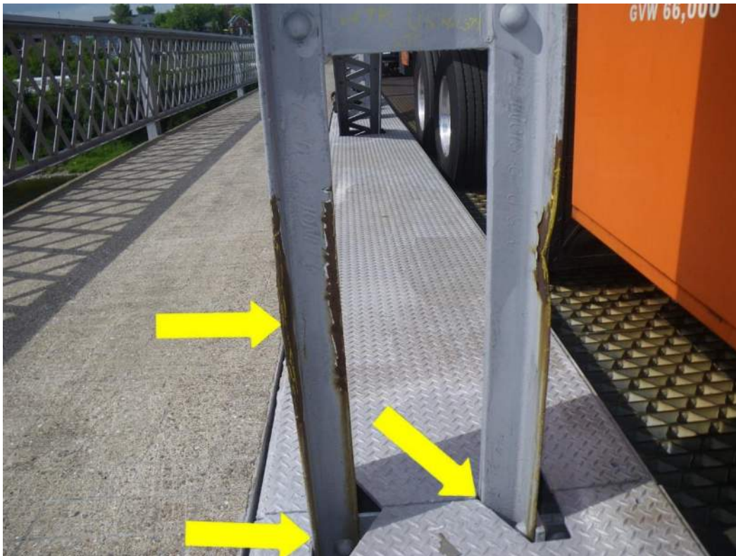
Photo 69: Vertical U5NL5N near Curb, South Face, West Truss, Span 3 - Bend and gouge of flange angles due to collision damage. Note flange angles in contact with curb.
