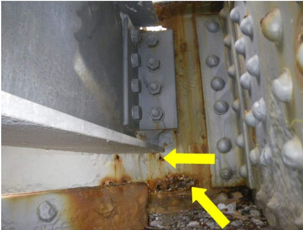
Photo 47: Floorbeam FB0S at Stringer S9, North Face, Span 4 - Web section loss below stringer connection including areas of 100% section loss. Note lower lateral bracing with rivet head loss.
