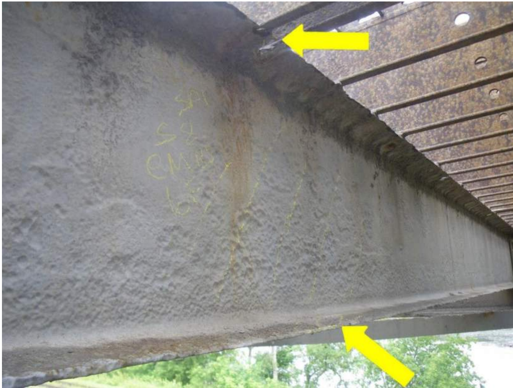
Photo 35: Stringer S8 at Midspan, between Floorbeams FB0N and FB1N, West Face, Span 1 - Section loss of flanges and web. Note top flange with 100% section loss of the outer edge including a vacant drilled hole.
