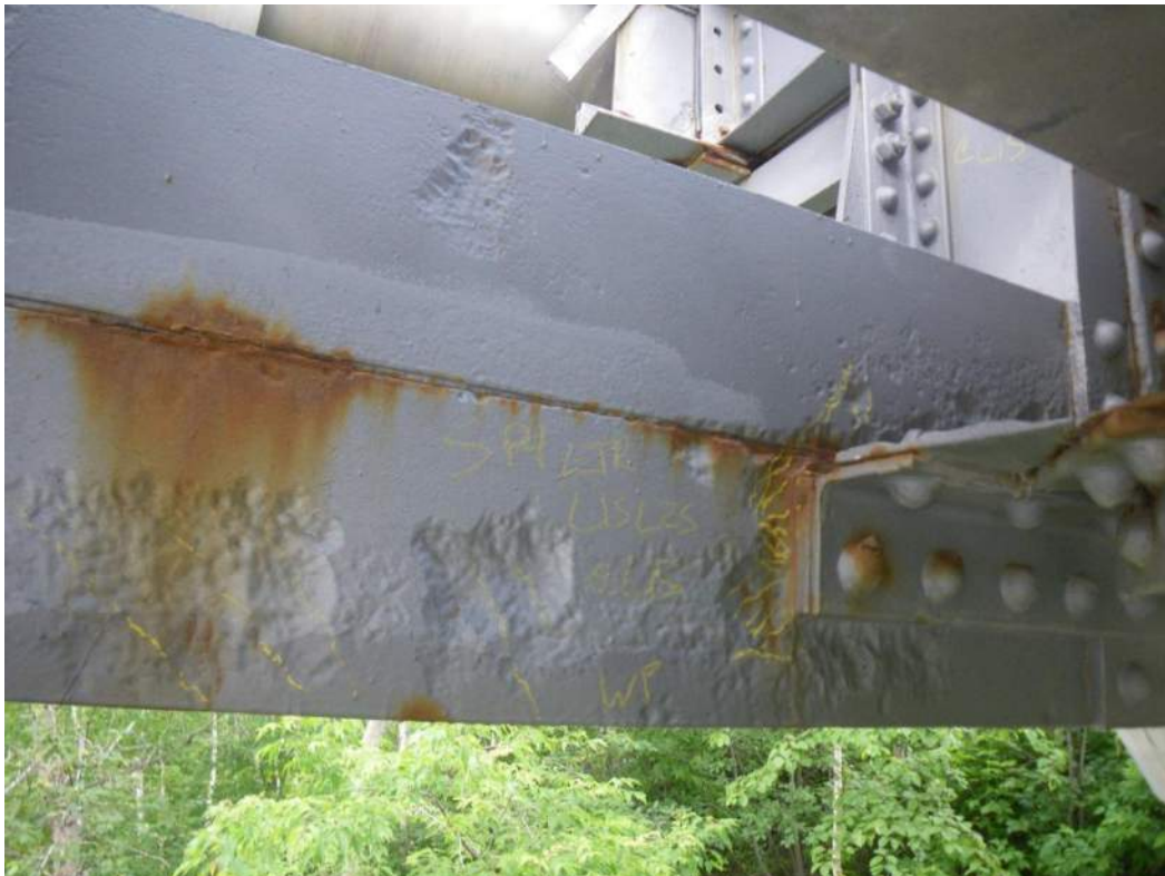
Photo 56: Lower Chord L2SL1S at Panel Point L1S, West Face, East Truss, Span 4 - Section loss of vertical legs. Note section loss of lower lateral bracing connection plate.
