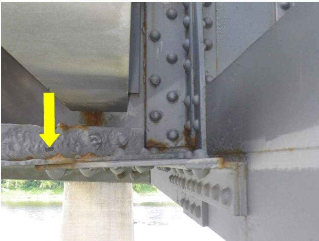
Photo 70: Lower Lateral Bracing Member at Panel Point L3S, East Truss, Span 1, Looking North - Section loss including area of 100% section loss. Note rivet head loss.
