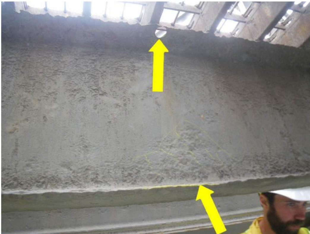
Photo 37: Stringer S6 at Midspan, between Floorbeams FB1N and FB2N, East Face, Span 1 - Section loss of flanges and web. Note top flange with 100% section loss of the outer edge including a vacant drilled hole.
