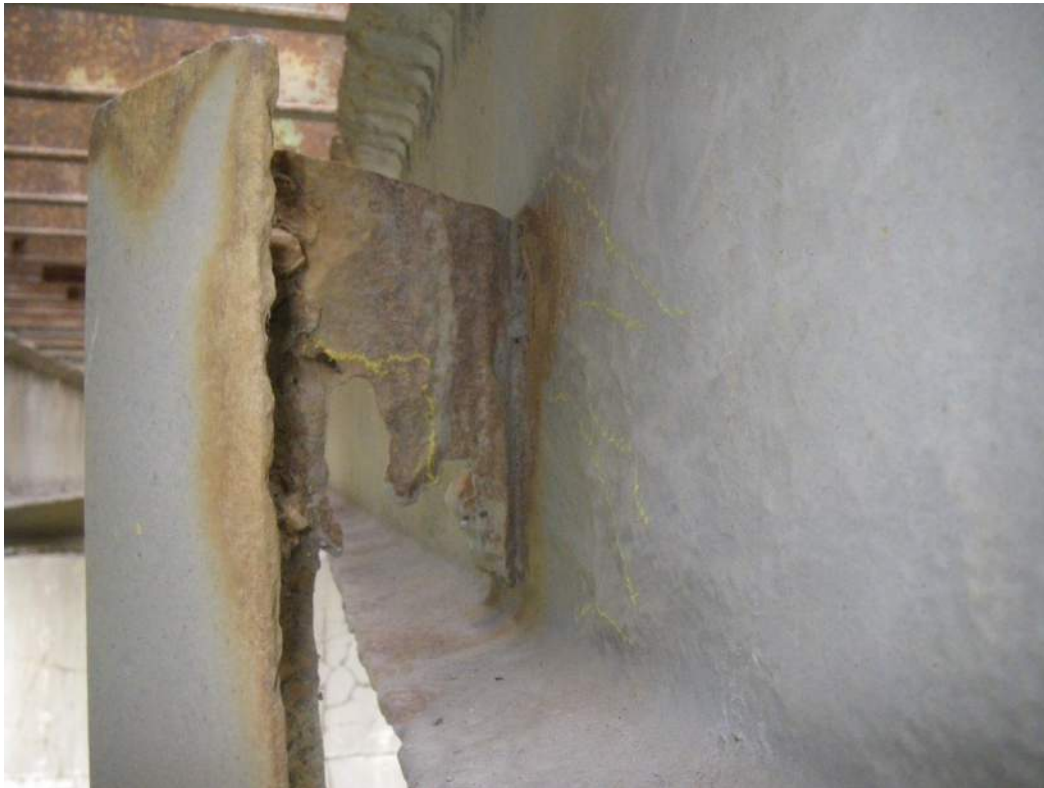
Photo 39: Stringer S5 at Midspan, between Floorbeams FB5N and FB6, West Face, Span 1 - Web section loss adjacent to lateral bracing connection plate. Note lower lateral bracing bent plate with area of 100% section loss.
