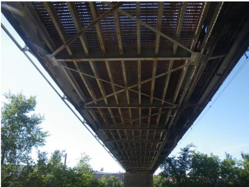
Photo 8: Underside of Span 1 near North Abutment, Looking South. Note areas of failed paint system on stringers and floorbeams.
