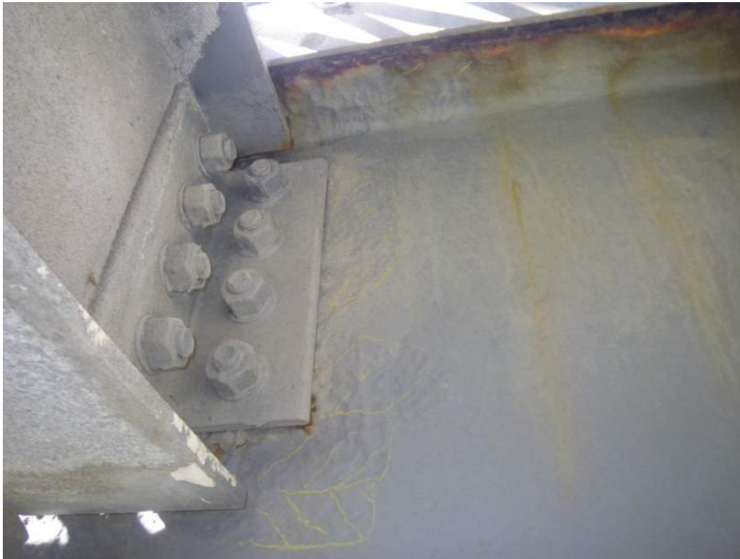
Photo 43: Floorbeam FB5S at Stringer S2, South Face, Span 4 - Web and top flange section loss adjacent to/above stringer connection.
