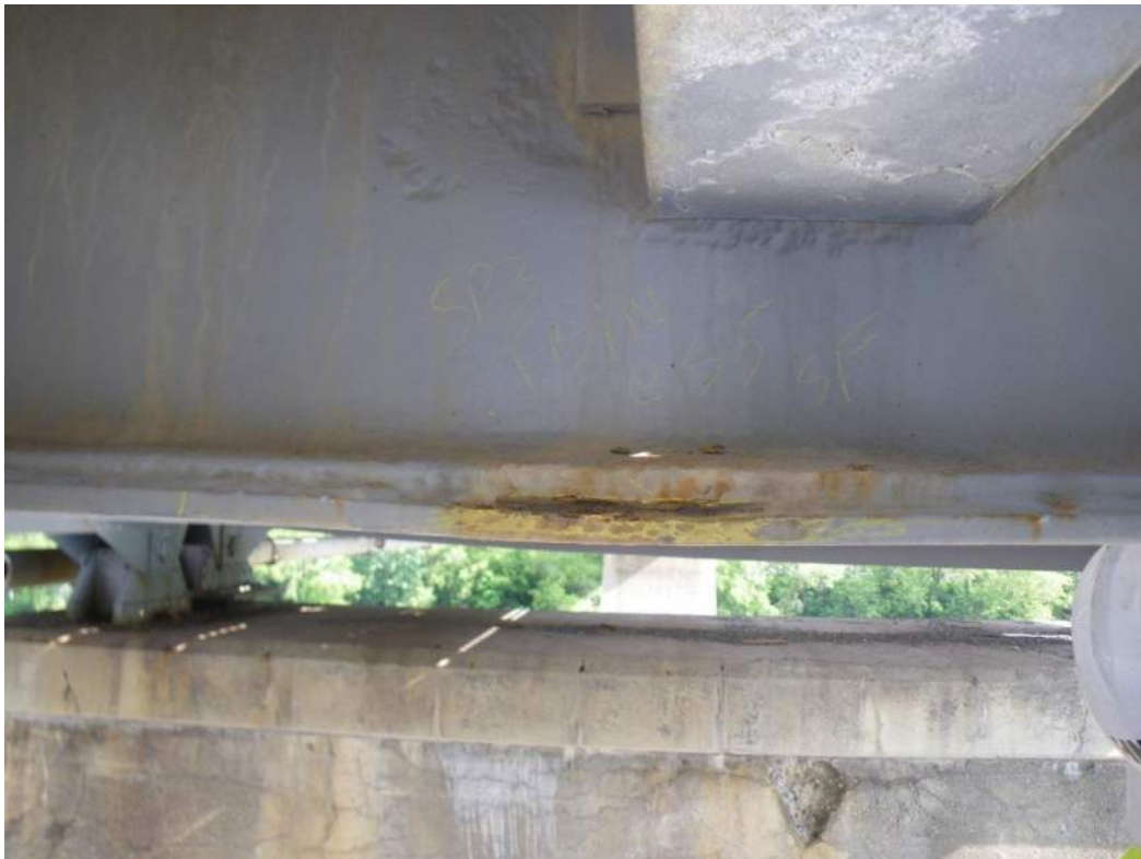
Photo 48: Floorbeam FB1N at Stringer S5, South Face, Span 3 - Bottom flange cover plate with bend. Note gap in weld between bottom flange and cover plate.
