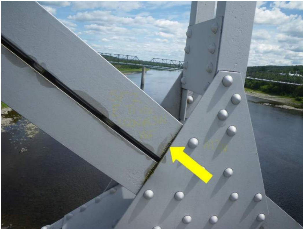
Photo 65: Diagonal U2NL4N at Panel Point M3N, West Face, East Truss, Span 2 - Section loss of both flange angles along gusset plate. Note impacted rust between gusset plate and flange angles.
