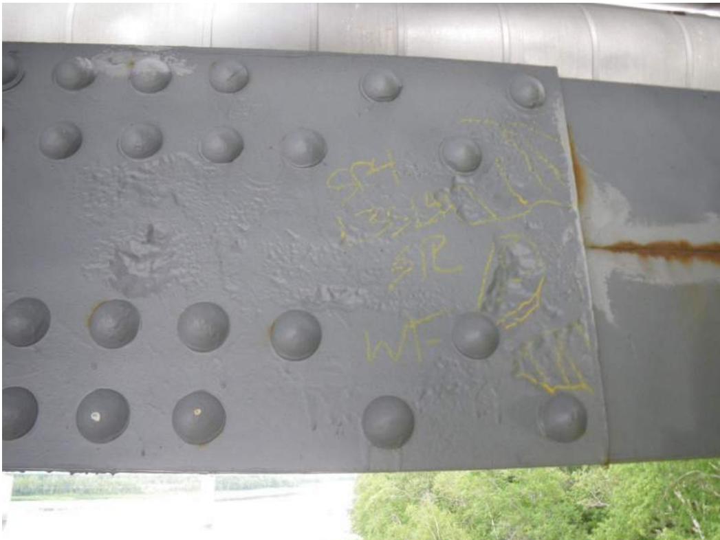
Photo 62: Lower Chord L4SL3S Splice, West Face, East Truss, Span 4 - Section loss of splice plate. Note lower chord with area of prime coat only and surface rust.
