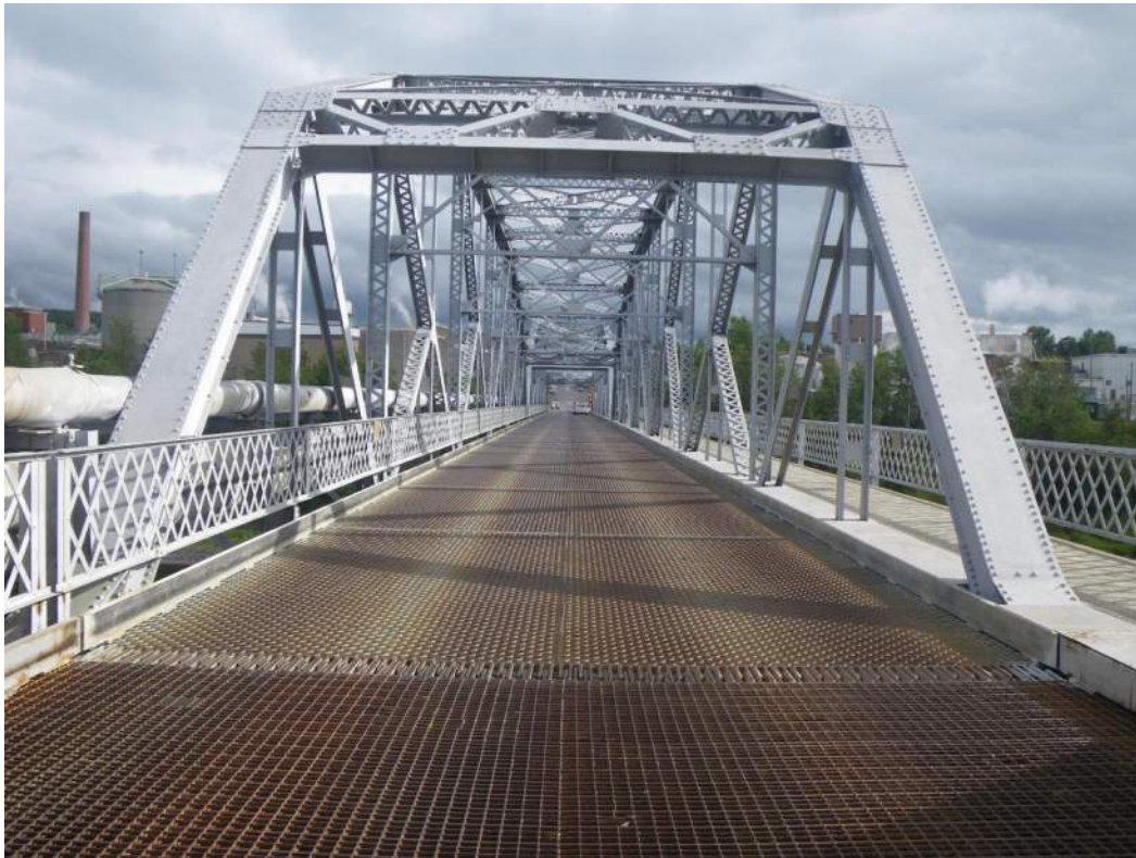
Photo 7: Typical Top of Deck at Pier 2, Looking South into Span 3. Note curbs with tire scrapes and failed paint system.
