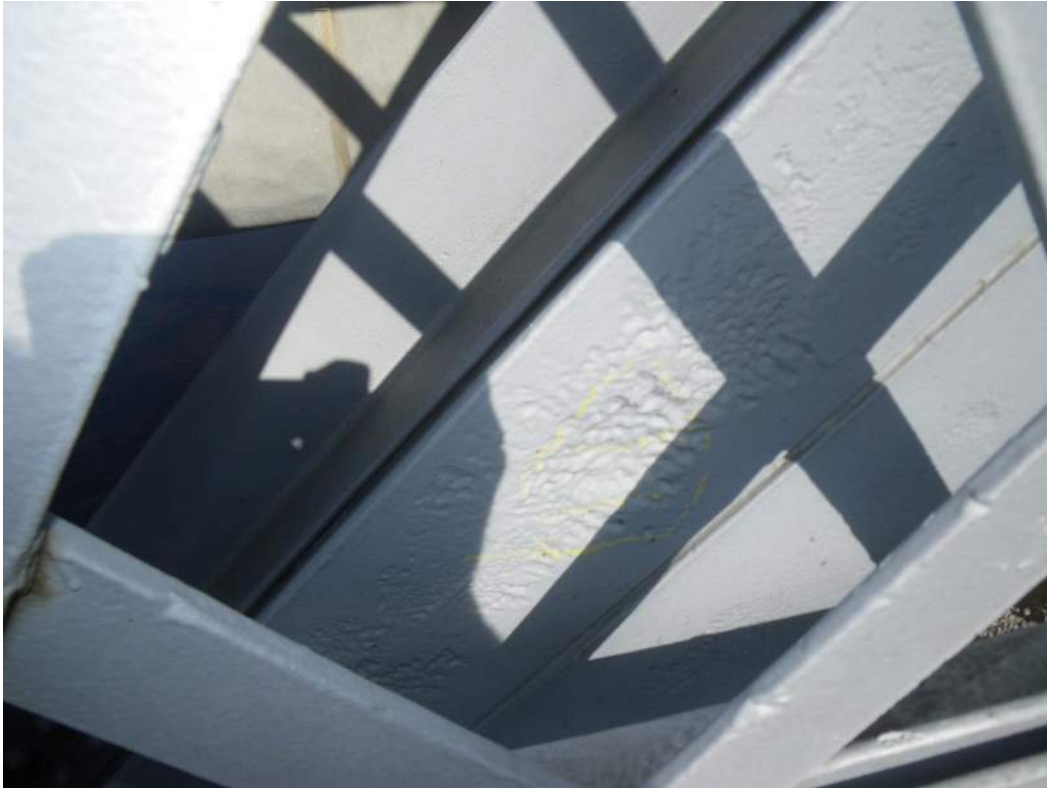
Photo 63: Diagonal L2SU1S near Deck, West Face, East Truss, Span 3 - Flange angle section loss.
