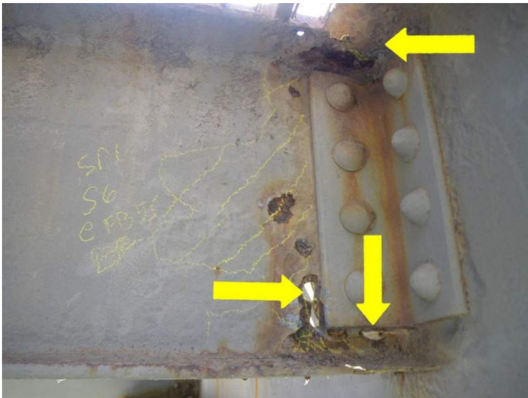
Photo 38: Stringer S6 at South Side of Floorbeam FB5S, East Face, Span 1 - Section loss of flanges and web including areas of 100% section loss. Note failed paint system.
