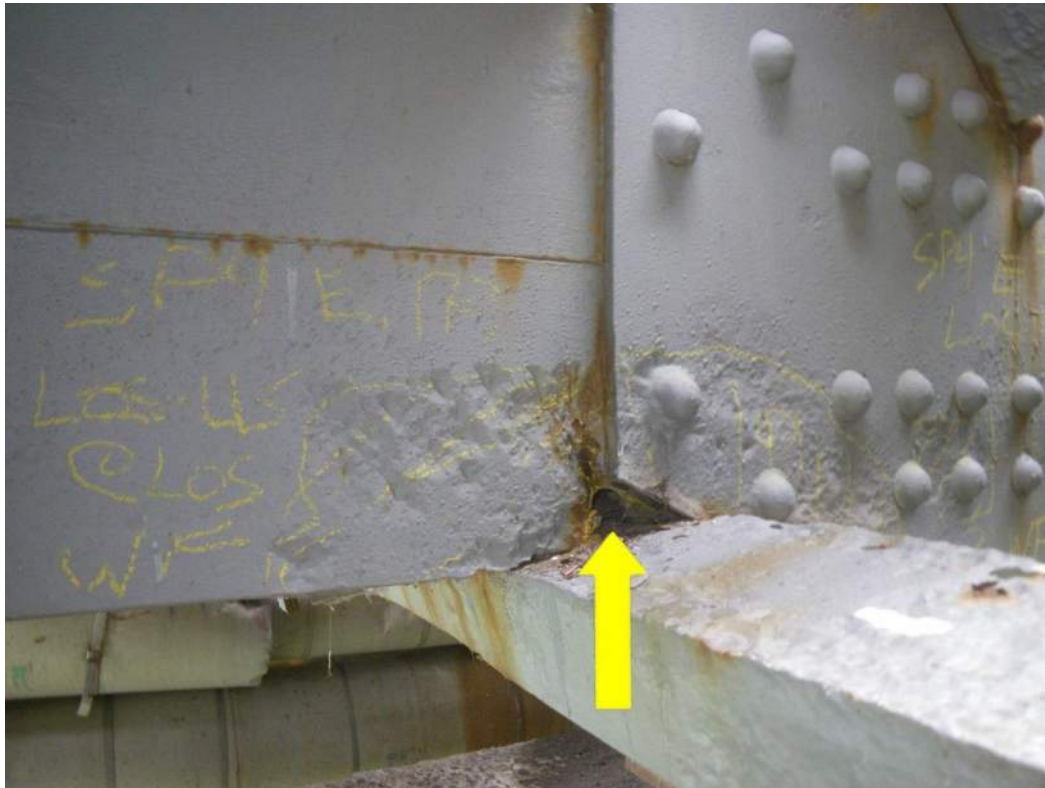
Photo 57: Lower Chord L1SL0S at Panel Point L0S, East Truss, Span 4 - Vertical leg section loss including area of 100% section loss. Note abandoned utility support angle in contact with lower chord and gusset plate section loss.
