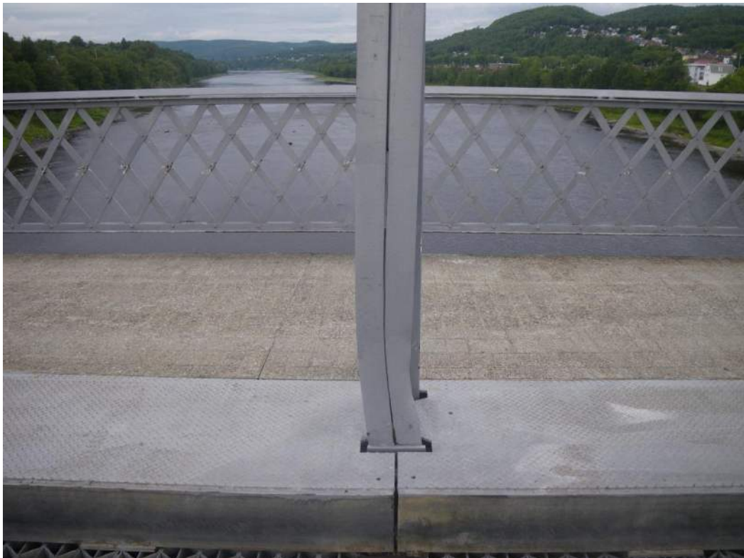
Photo 68: Vertical U3NL3N near Curb, East Face, West Truss, Span 3 - Flange angles with sweep, rotation and bend due to collision damage.
