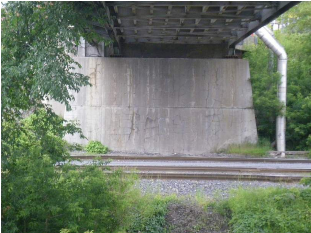
Photo 10: North Abutment, Looking North. Note breastwall with map cracking with moisture and scattered areas with efflorescence.
