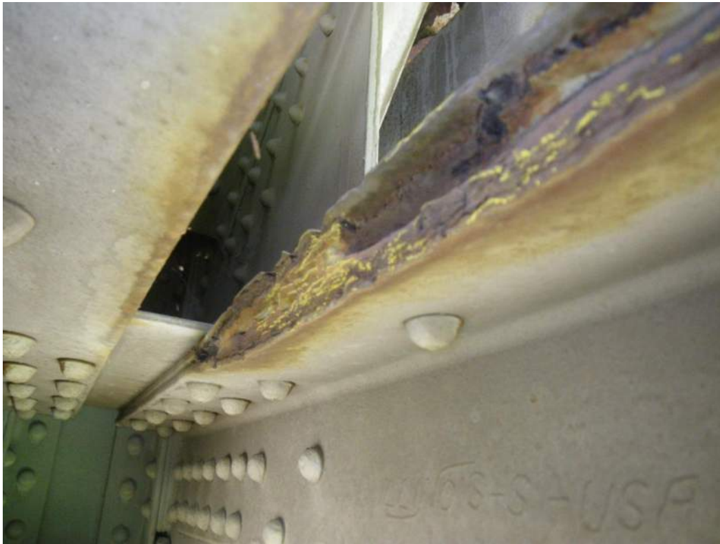
Photo 53: Lower Chord L1SL0S at Panel Point L0S, West Truss, Span 1, Looking South - Horizontal legs with section loss including 100% section loss of edge and impacted rust.
