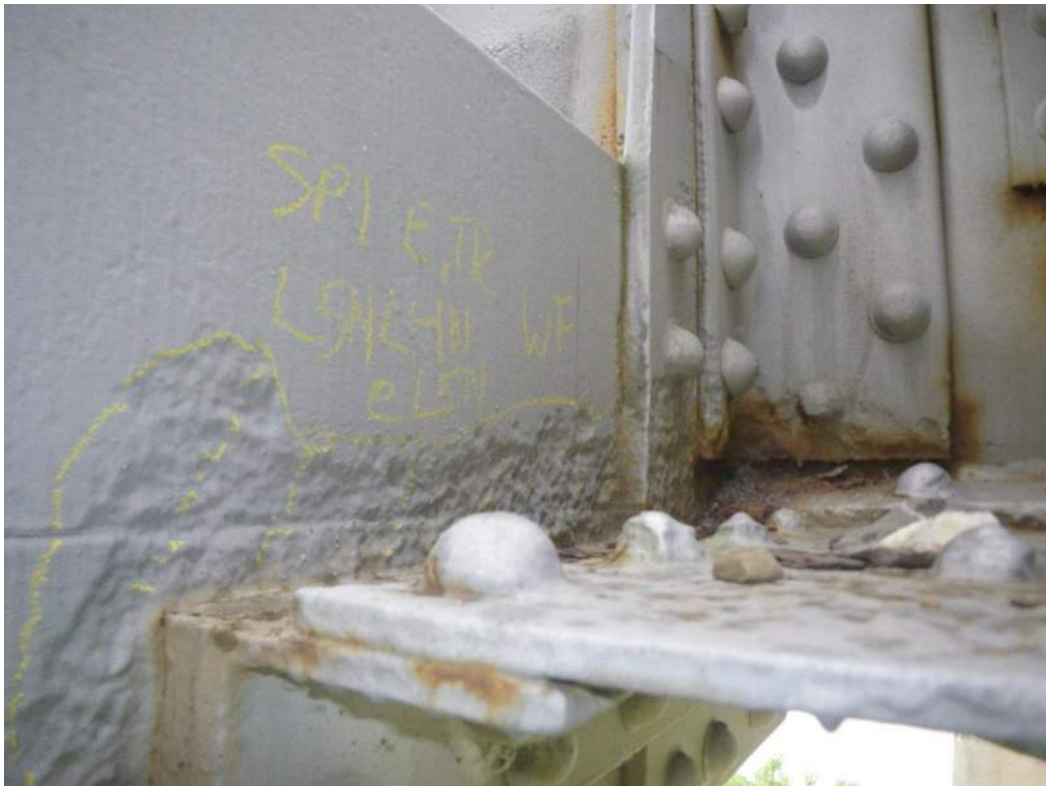
Photo 52: Lower Chord L4NL5N at Panel Point L5N, West Face, East Truss, Span 1 - Section loss of vertical legs along lower lateral bracing connection plate. Note section loss of gusset plate and floorbeam connection angle.
