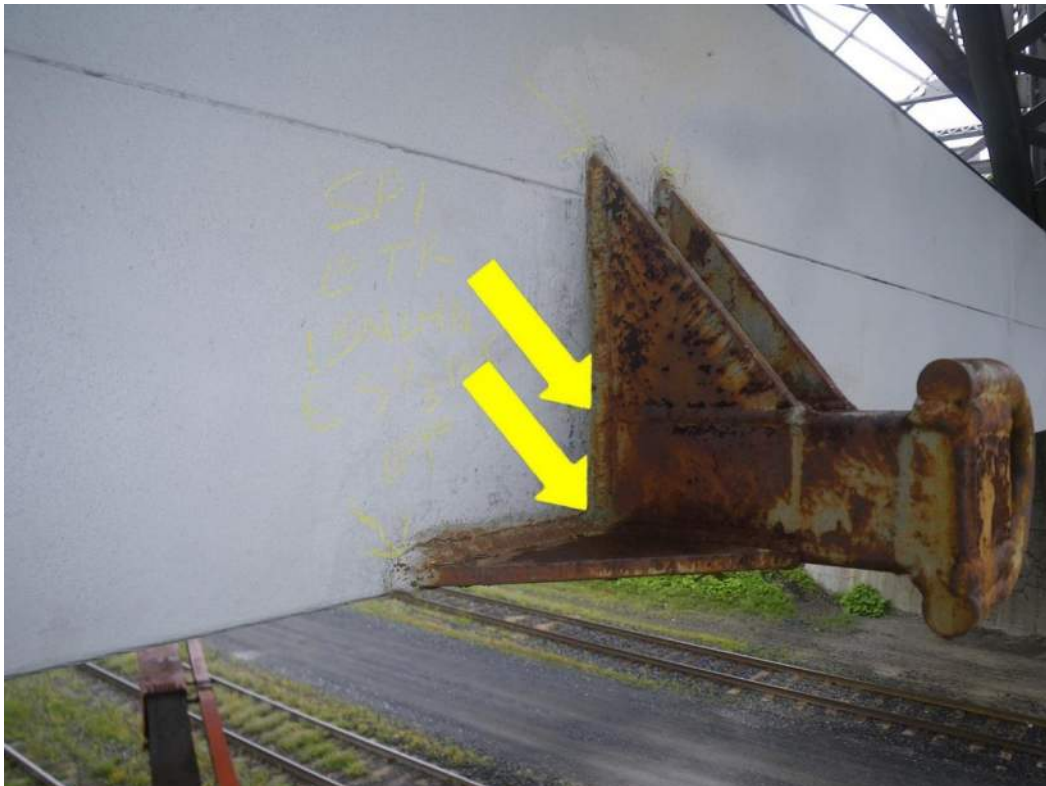
Photo 60: Lower Chord L4NL5N at South Third Point, East Face, East Truss, Span 1 - Intersecting welds of the abandoned anchor point on the flange angles.
