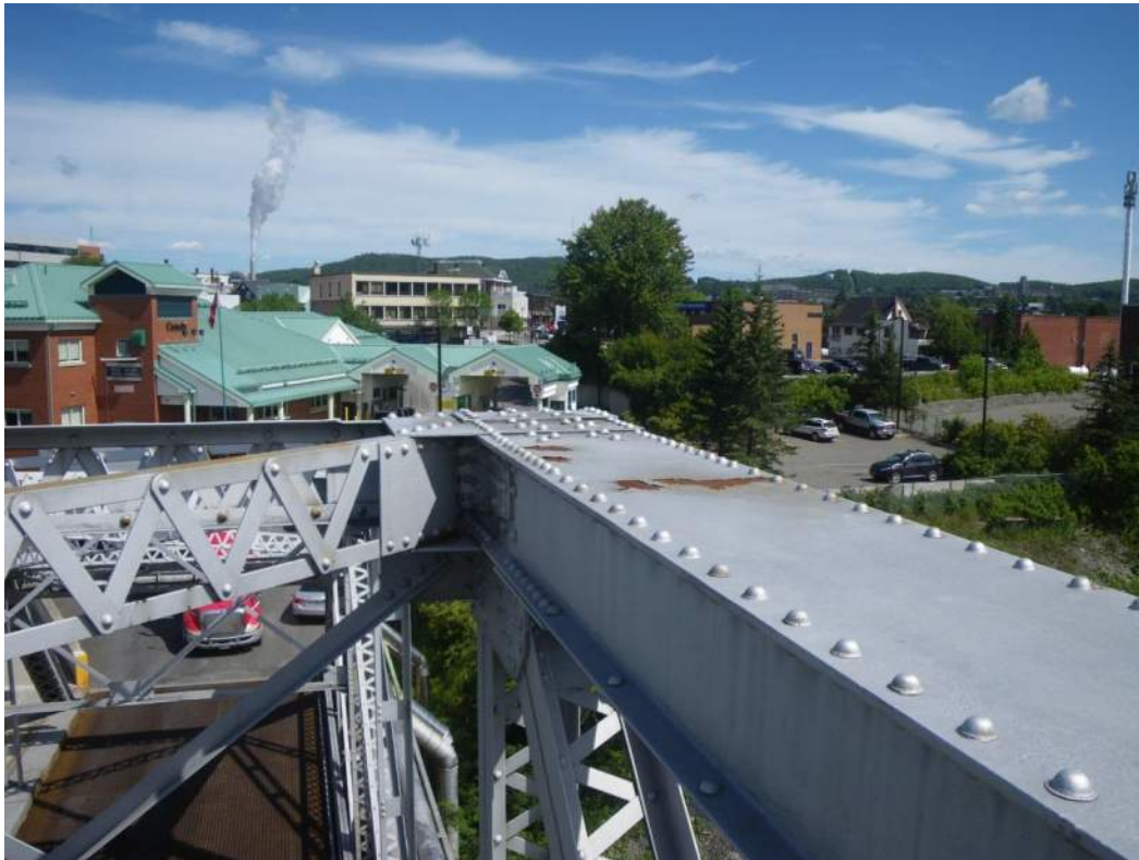
Photo 51: Upper Chord U5NU6 near Panel Point U5N, East Truss, Span 1, Looking North - Areas of surface rust and a failed paint system.
