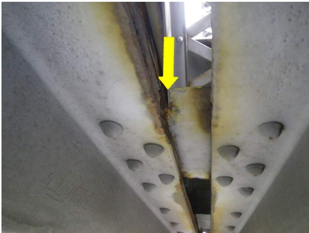
Photo 58: Lower Chord L2NL3N near Panel Point L2N, West Truss, Span 1, Looking North - Impacted rust between horizontal legs of flange angles. Note section loss of batten plate including area of 100% section loss.
