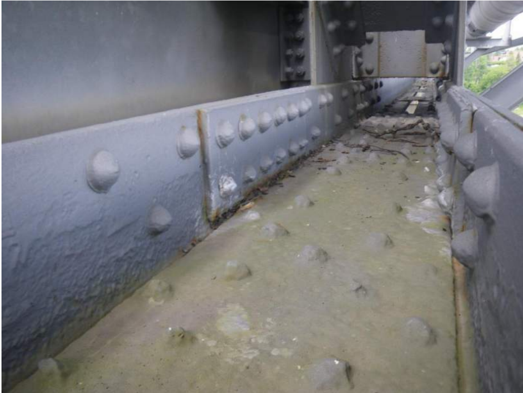
Photo 61: Lower Chord L6L5S Splice near Panel Point L6, East Truss, Span 4, Looking North - Section loss of splice plate. Note rivet head loss.
