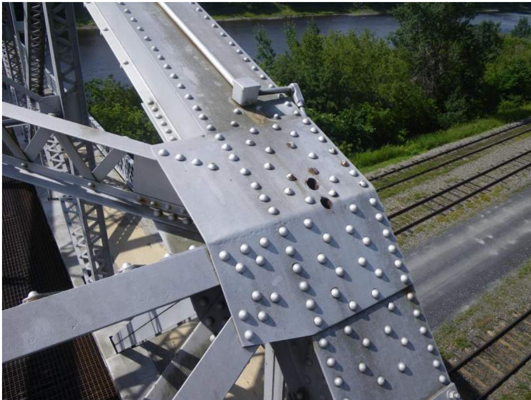
Photo 50: Upper Chord U1NU2N at Panel Point U1N, West Truss, Span 1, Looking Southwest - Vacant drilled holes in top plate and portal/upper lateral bracing connection plate.
