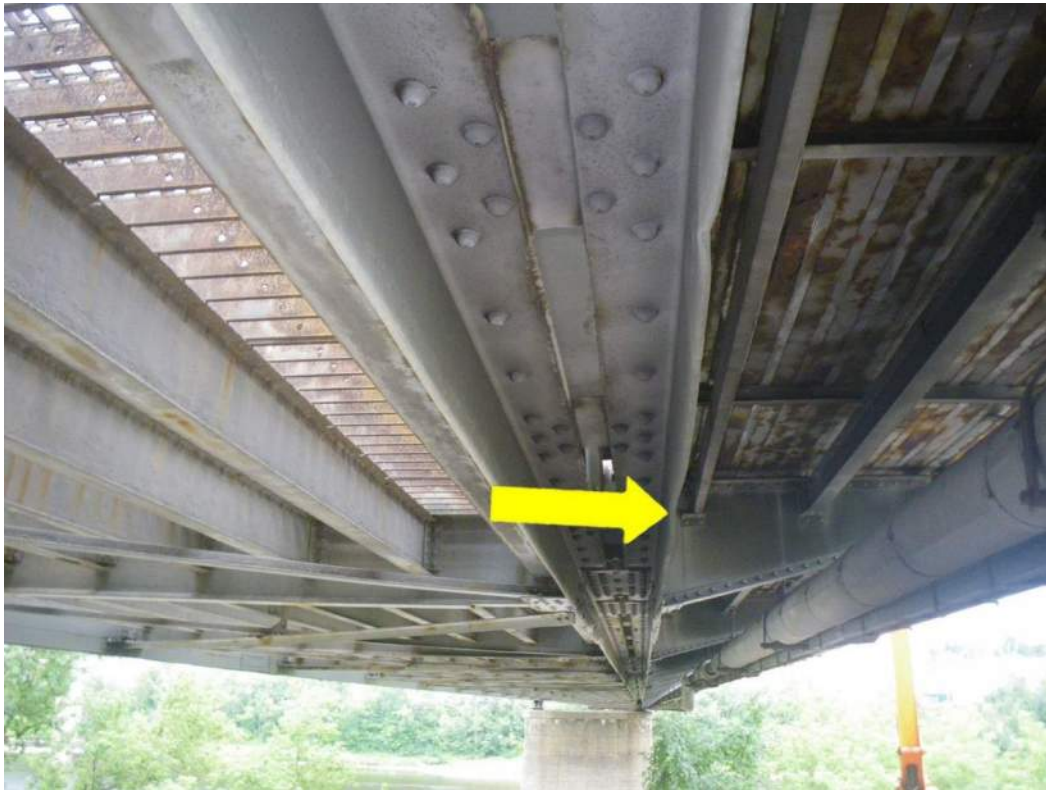
Photo 59: Lower Chord L1NL2N near Panel Point L1N, West Truss, Span 1, Looking South - Bends in the vertical leg of flange angle.
