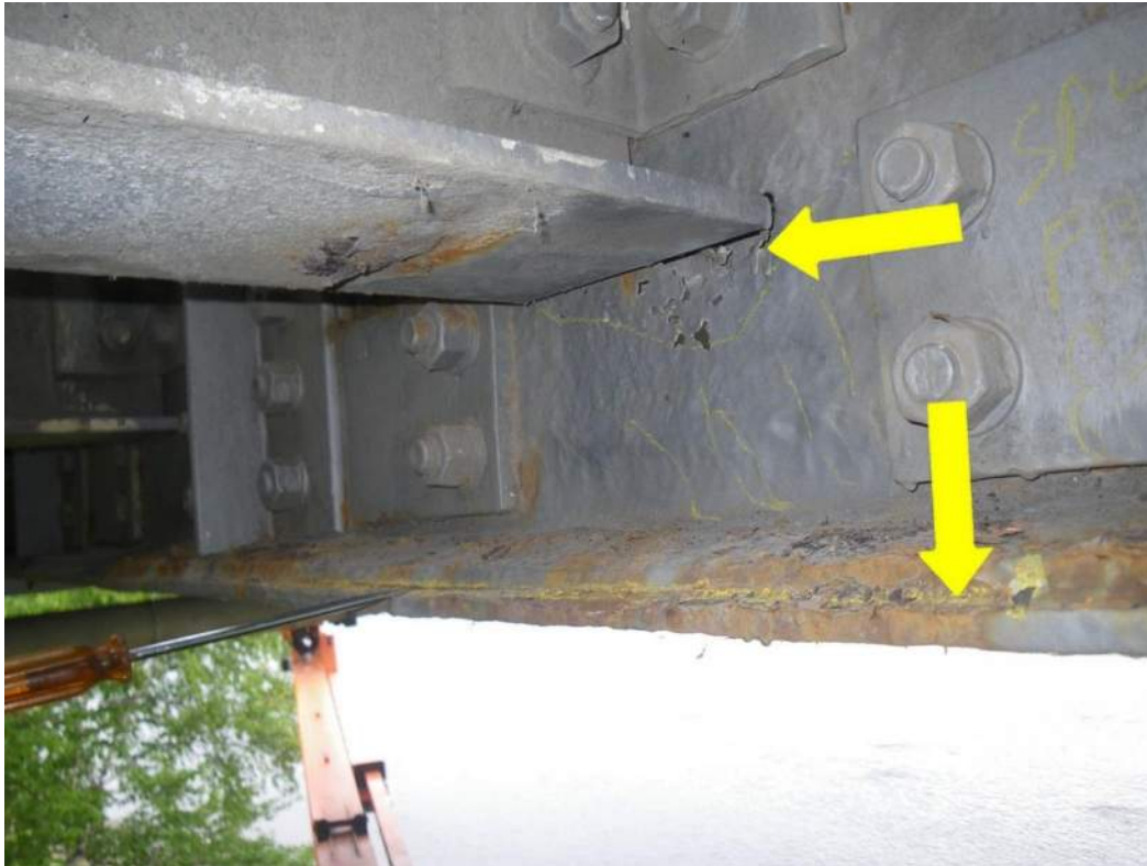
Photo 45: Floorbeam FB2S at Stringer S4, South Face, Span 4 - Web section loss below stringer connection including area of 100% section loss and bottom flange section loss. Note cracked weld between bottom flange and cover plate with gap.
