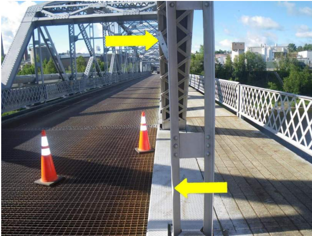
Photo 67: Vertical U1SL1S near Curb, North Face, West Truss, Span 2 - Bend of flange angle due to collision damage. Note abandoned sign support bar protruding outward from the vertical.
