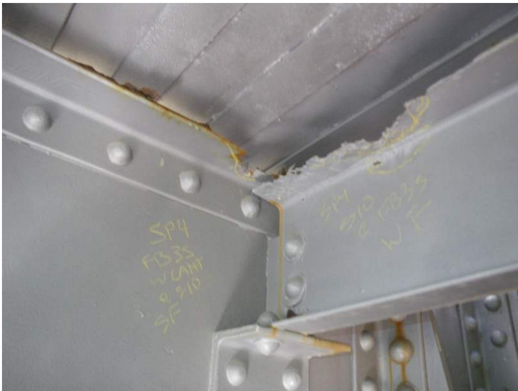
Photo 40: Stringer S10 at South Side of Floorbeam FB3N, West Face, Span 4 - Areas of 100% section loss in top flange and web. Note area of 100% section loss in floorbeam cantilever top flange.
