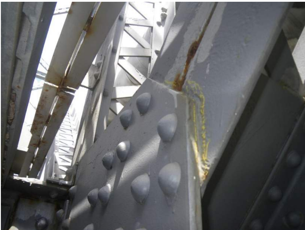
Photo 64: Diagonal L6U4S at Panel Point L6, West Face, East Truss, Span 4, Looking North - Section loss of both flange angles along gusset plate.
