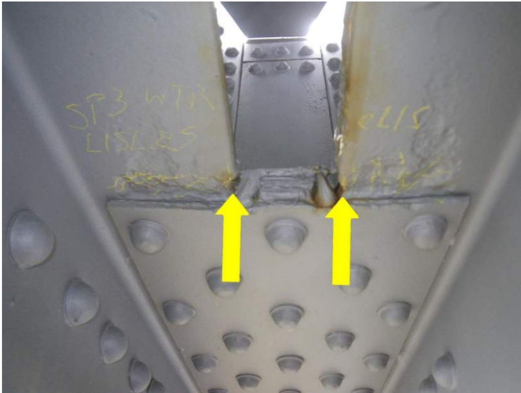
Photo 55: Lower Chord L2SL1S at Panel Point L1S, West Truss, Span 4, Looking South - Section loss of the horizontal legs along batten plate including 100% section loss of edge.
