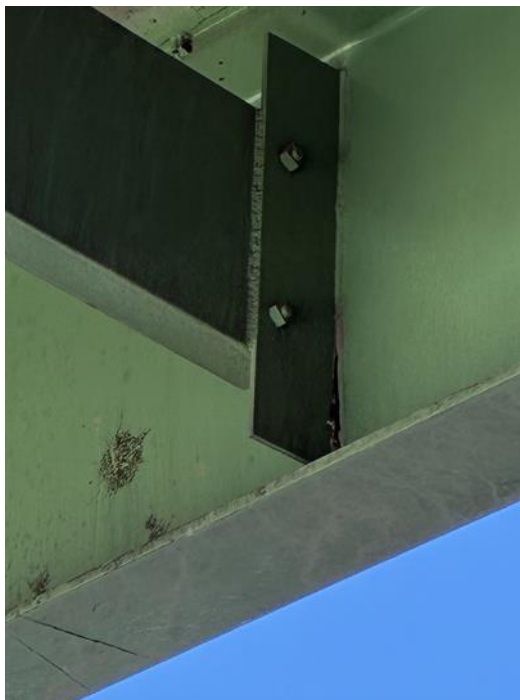
PHOTO 2 Condition Description Adjacent diaphragm. Tear in web connecting the web and connection plate.
