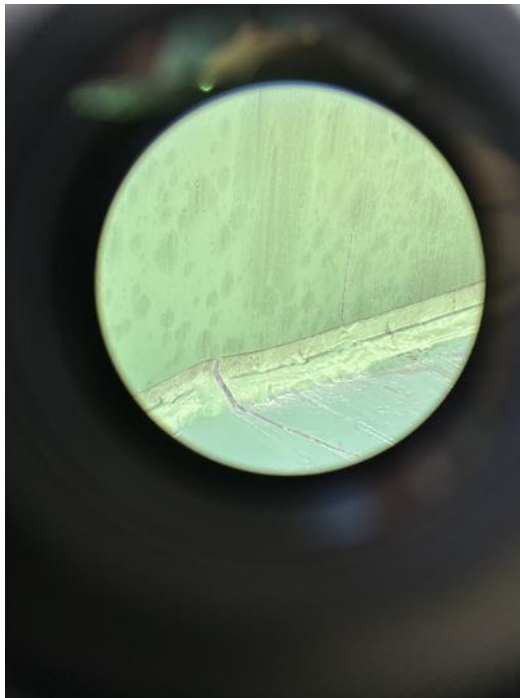
PHOTO 6 Condition Description Beam crack through spotting scope.
