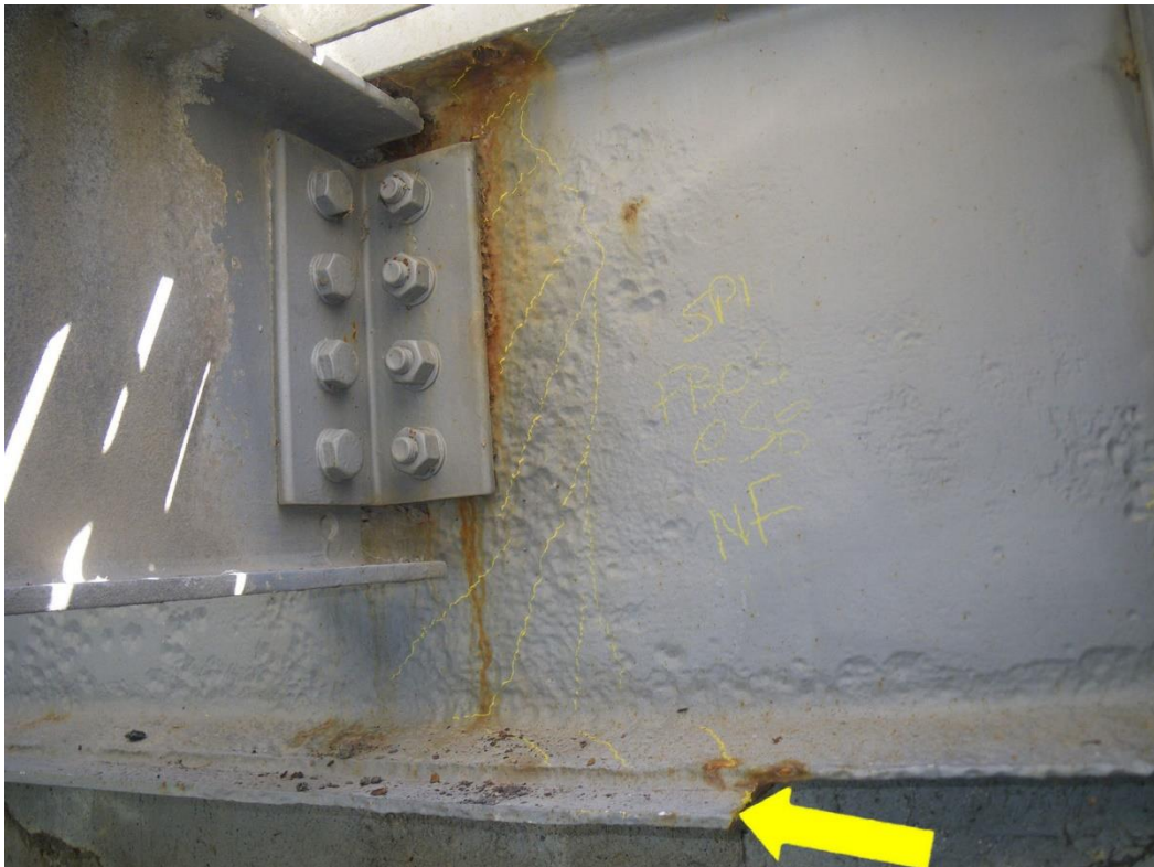
Photo 36: Floorbeam FB0S at Stringer S8, North Face, Span 4 - Web, bottom flange and cover plate section loss adjacent to/below stringer connection. Note misaligned bottom flange cover plate.
