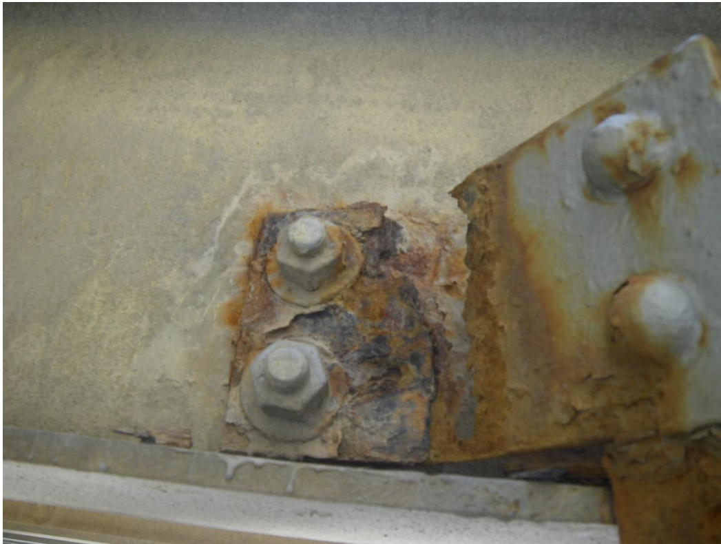
Photo 51: Lower Lateral Bracing Midspan Connection at Stringer S5, between Floorbeams FB5S and FB4S, Span 3, Looking East - Area of 100% section loss.
