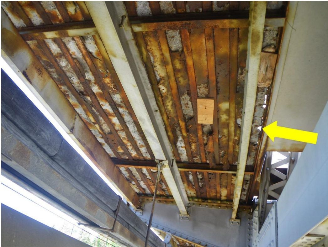
Photo 17: Stay-In-Place Forms between Floorbeams FB4S and FB3S, Span 1, Looking North - 100% section loss by full sidewalk width by full floorbeam bay length. Note sidewalk with failed paint system and rust of longitudinal bars, up to full depth spalls and previous repairs.
