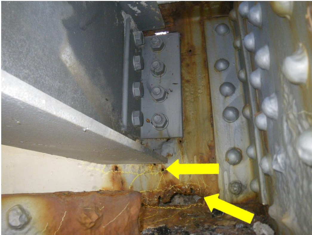
Photo 37: Floorbeam FB0S at Stringer S9, North Face, Span 4 - Web section loss below stringer connection including areas of 100% section loss. Note floorbeam connection, lower lateral bracing and lower chord gusset plate with rivet head loss.
