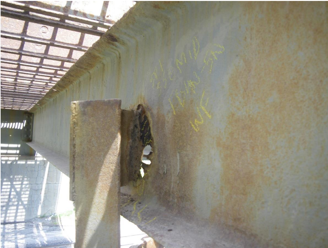
Photo 27: Stringer S5 at Midspan, between Floorbeams FB4N and FB5N, West Face, Span 1, Looking North - Web section loss adjacent to lateral bracing connection plate including area of 100% section loss.
