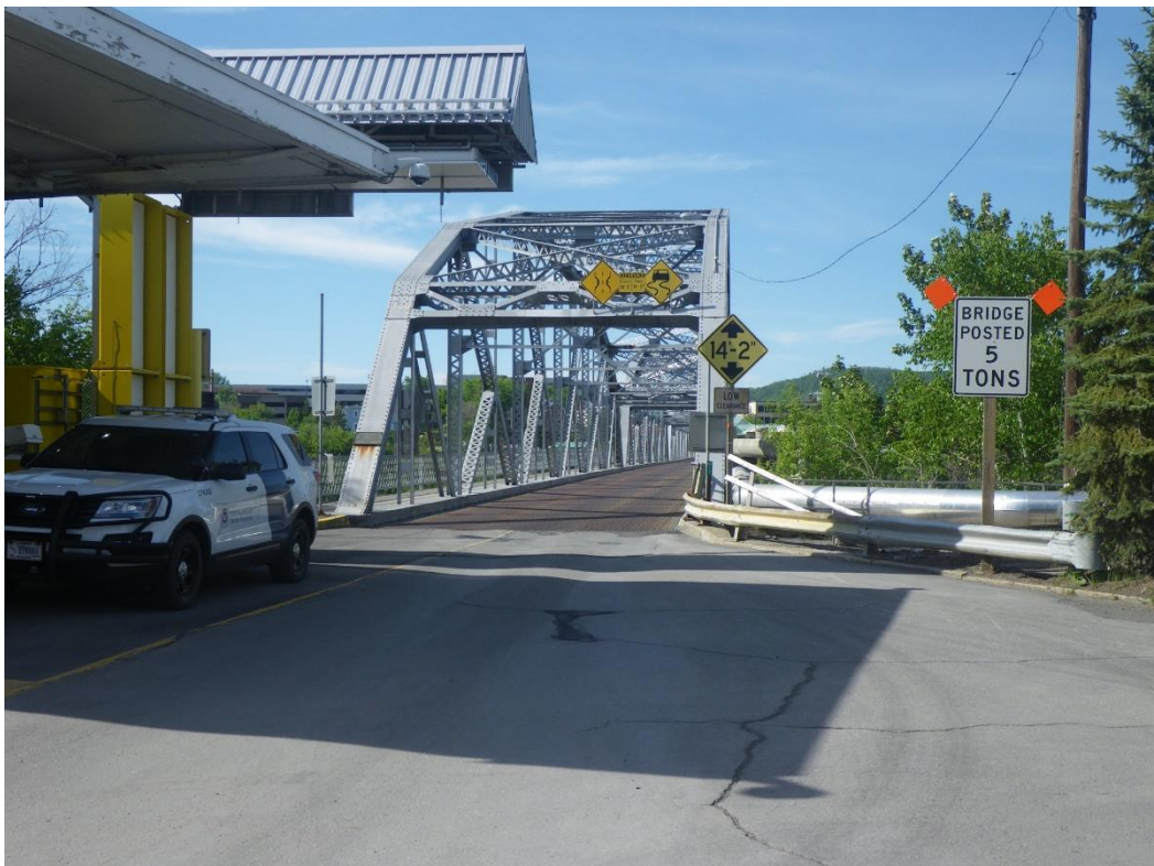
Photo 4: South Approach, Looking North. Note "At-Bridge" bridge load posting and vertical clearance signs.
