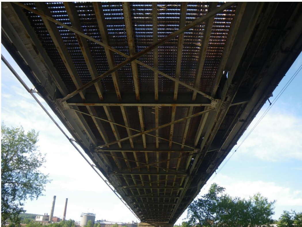
Photo 6: Underside of Span 1 near North Abutment, Looking South. Note conduits/abandoned pipe along west truss and areas of a failed paint system on the stringers and floorbeams.
