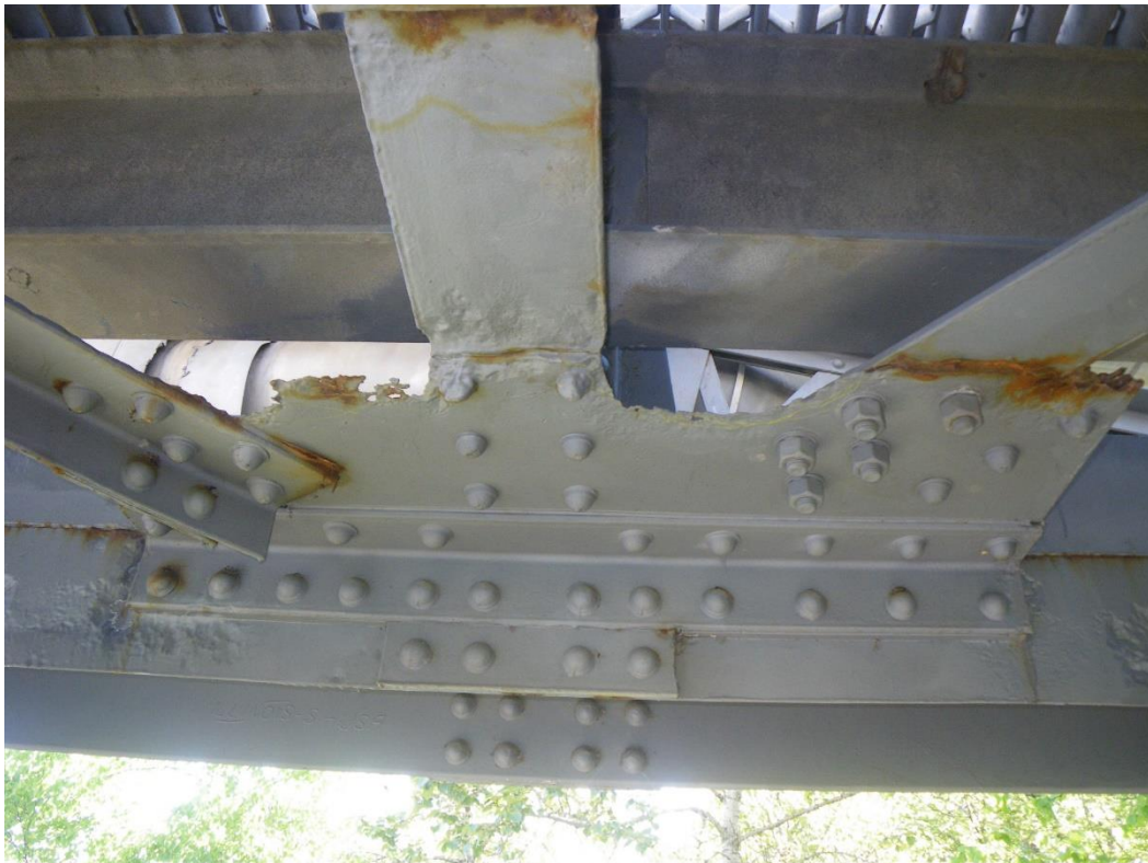
Photo 50: Lower Lateral Bracing Connection Plate at Panel Point L1S, East Truss, Span 4, Looking East - Areas of 100% section loss.
