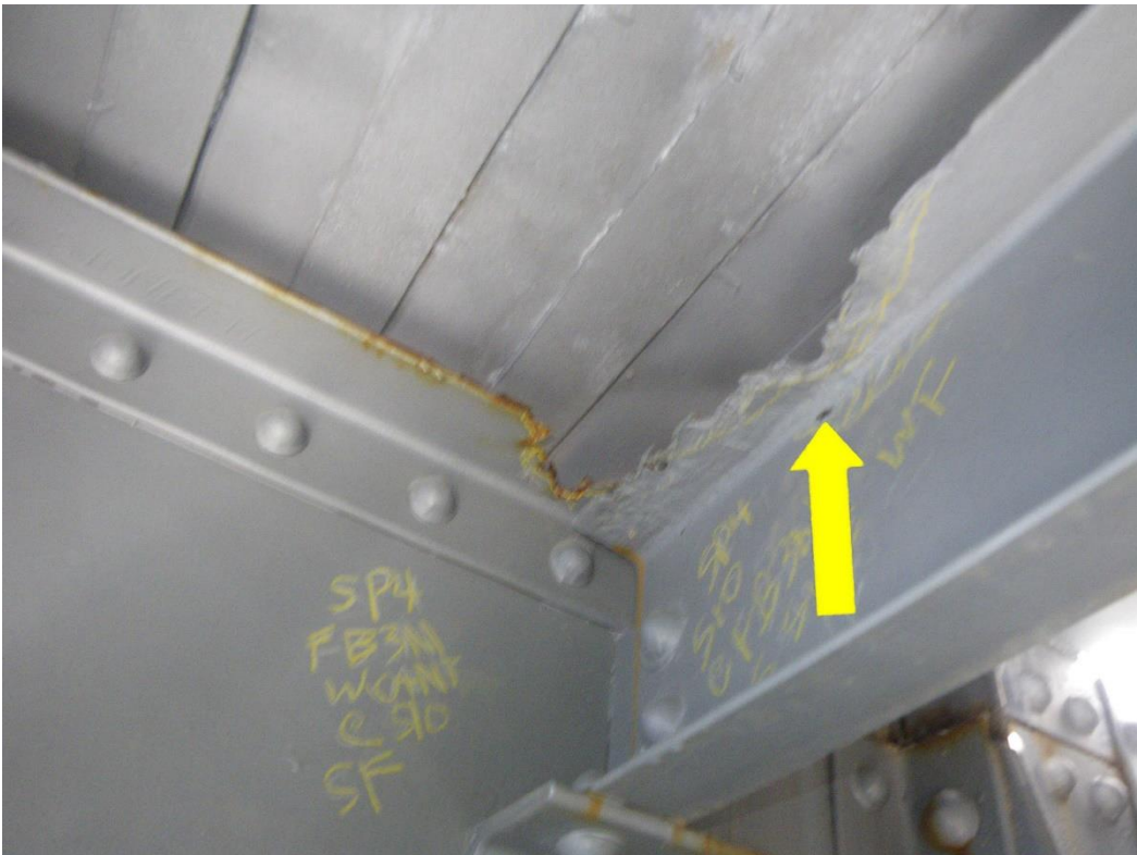
Photo 28: Stringer S10 at South Side of Floorbeam FB3N, West Face, Span 4, Looking Northeast - Areas of 100% section loss in top flange and web. Note area of 100% section loss in floorbeam cantilever top flange.
