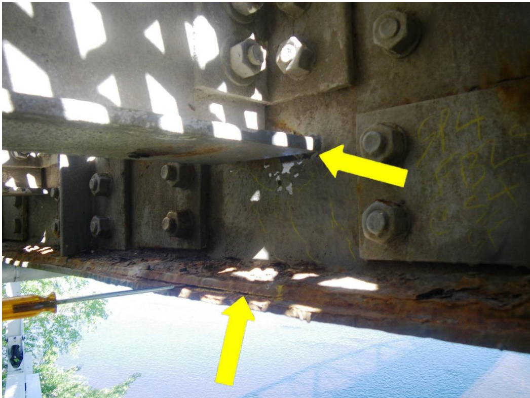
Photo 34: Floorbeam FB2S at Stringer S4, South Face, Span 4 - Web section loss below stringer connection including area of 100% section loss and bottom flange section loss. Note repair plates not covering 100% section loss and cracked/separated weld between bottom flange and cover plate.
