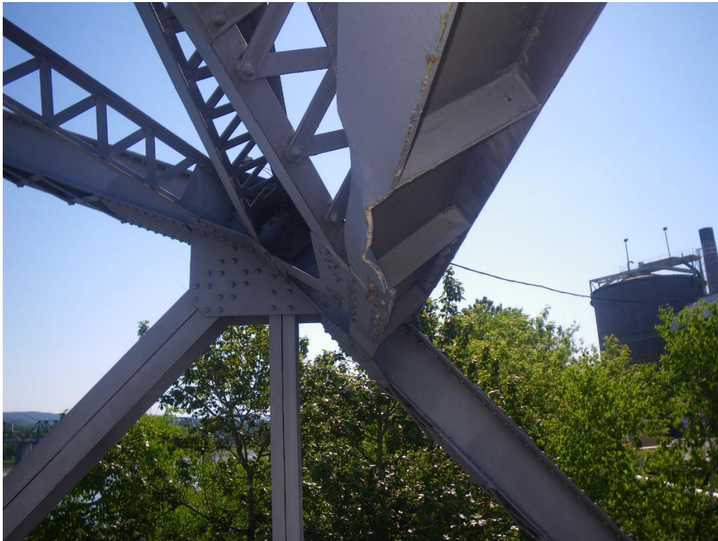
Photo 49: Portal Bracing Lower Transverse Brace above NB Lane, South Portal, Span 4, Looking East - Bottom flange with rotation/twisting, sweep and bend due to collision damage. Note cut out portion with above repair plate.
