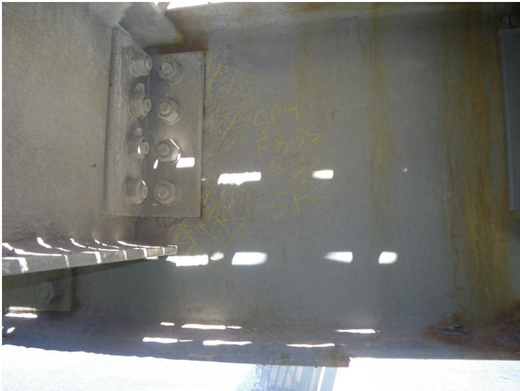
Photo 32: Floorbeam FB5S at Stringer S2, South Face, Span 4 - Web section loss adjacent to/above stringer connection and flange section loss.
