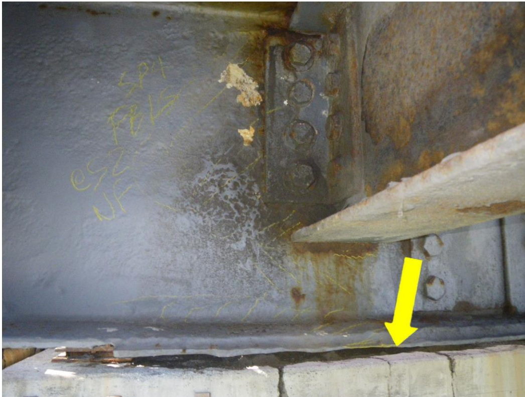
Photo 35: Floorbeam FB1S at Stringer S2, North Face, Span 4 - Web and bottom flange section loss adjacent to/below stringer connection. Note rust forming under paint system.
