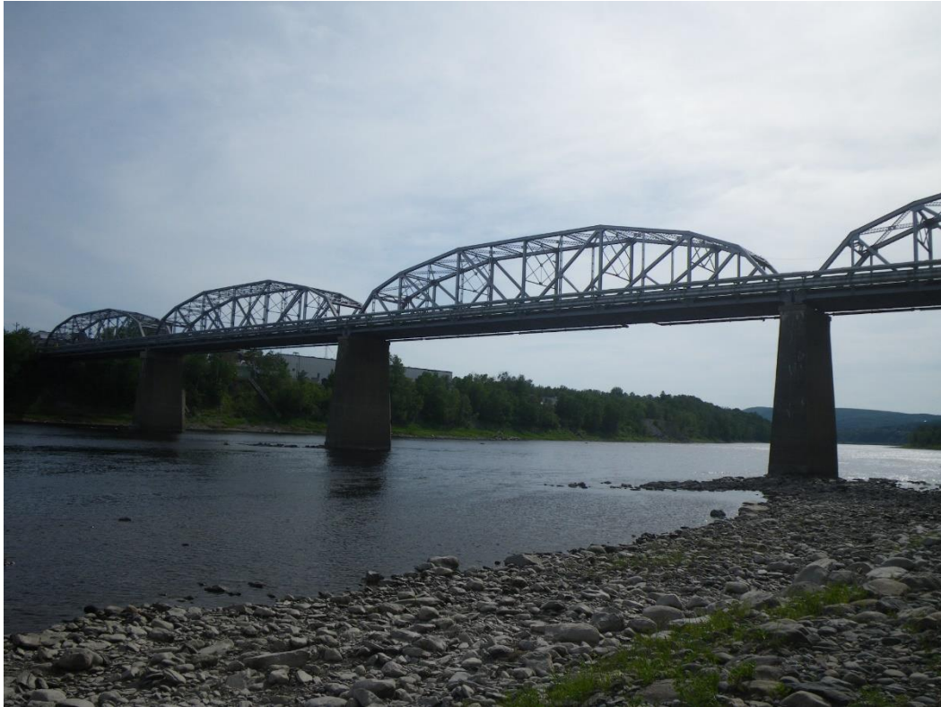
Photo 1: East Elevation, Looking Southwest. Note paper process pipes for the Twin Rivers Paper Company along east truss.
