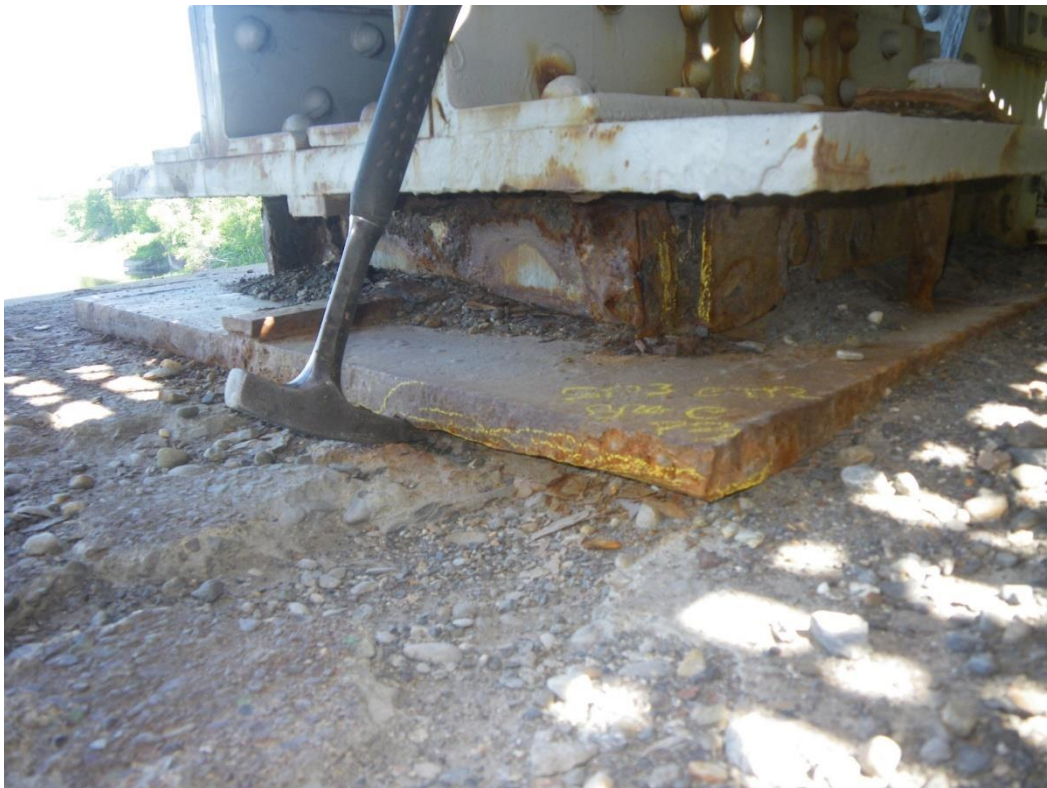
Photo 56: East Truss Bearing at Pier 3, North Face, Span 3, Looking Southeast - Undermining of masonry plate due to pier cap spall.
