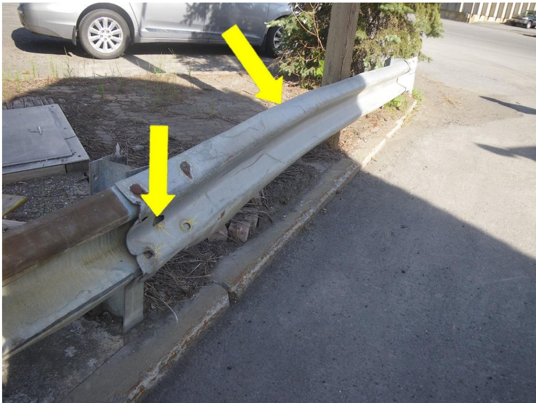
Photo 60: SE Approach Guardrail at Third Rail Post from South Abutment, Looking SE - Splice with 2 of 4 bolts in place, loose horizontal bolt connecting guardrail to rail post and bend of rail section due to collision damage.
