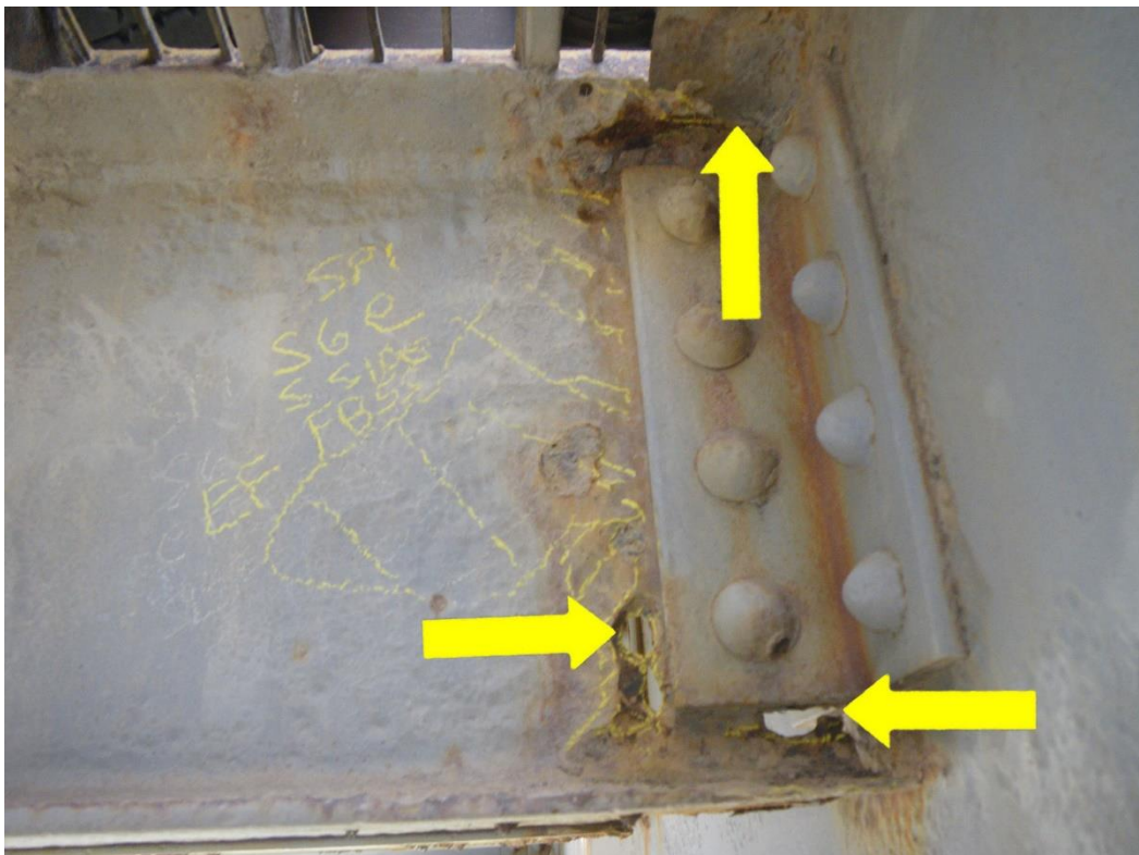
Photo 24: Stringer S6 at South Side of Floorbeam FB5S, East Face, Span 1 - Section loss of flanges and web including areas of 100% section loss. Note corrosion crack in web and failed paint system.
