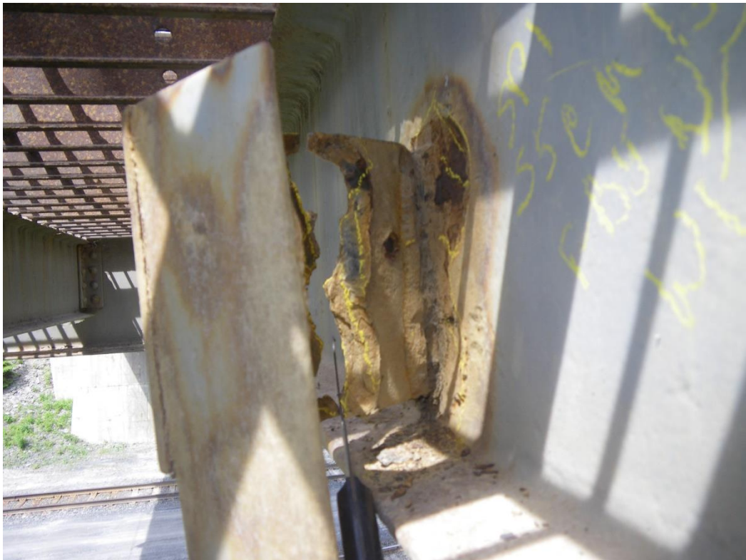
Photo 26: Stringer S5 at Midspan, btwn Floorbeams FB5N & FB6, West Face, Span 1, Looking North - Web section loss adj. to lateral bracing conn. plate. Note lower lateral bracing bent plate w/ 100% section loss by full height.
