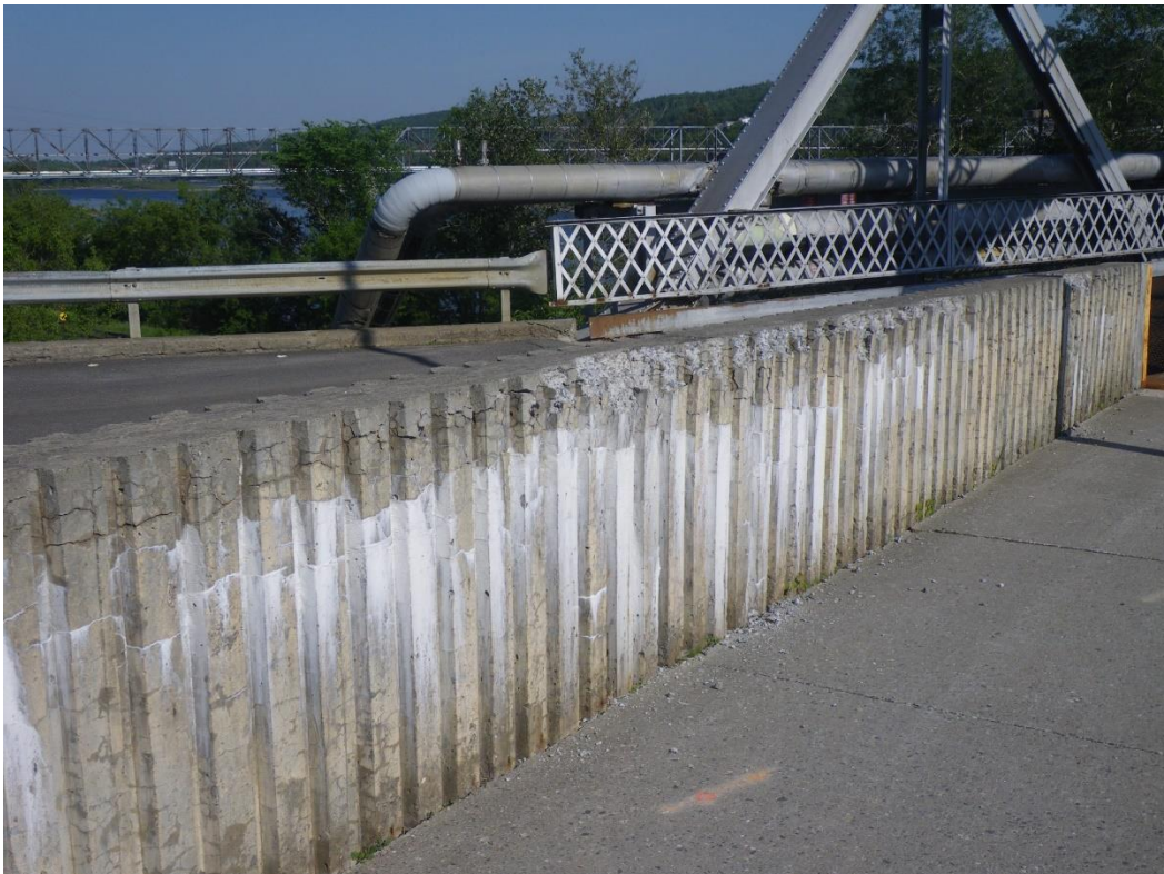
Photo 62: Northwest Traffic Barrier near North End, West Face, Looking Southeast - Extensive map cracking with moisture and efflorescence, delamination and spalls.
