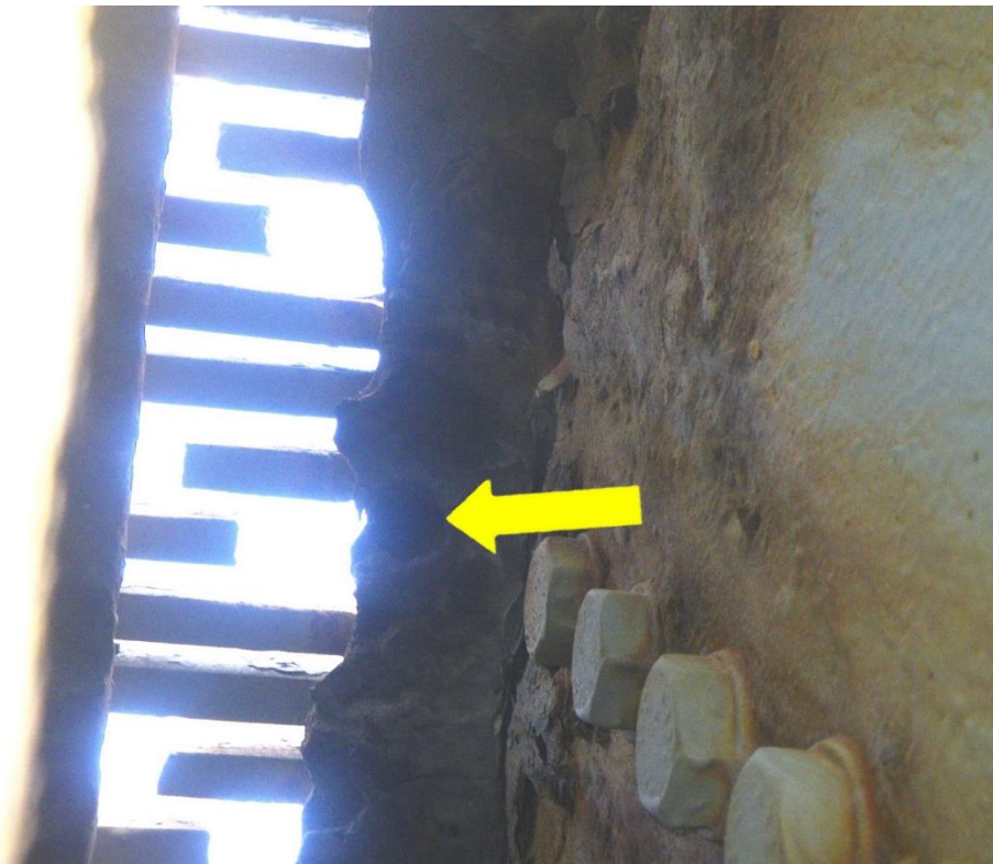
Photo 38: Floorbeam FB0S between Stringers S1 and S3, North Face, Span 2, Looking East - Top flange section loss including area of 100% section loss encompassing a vacant drilled hole. Note failed paint system.
