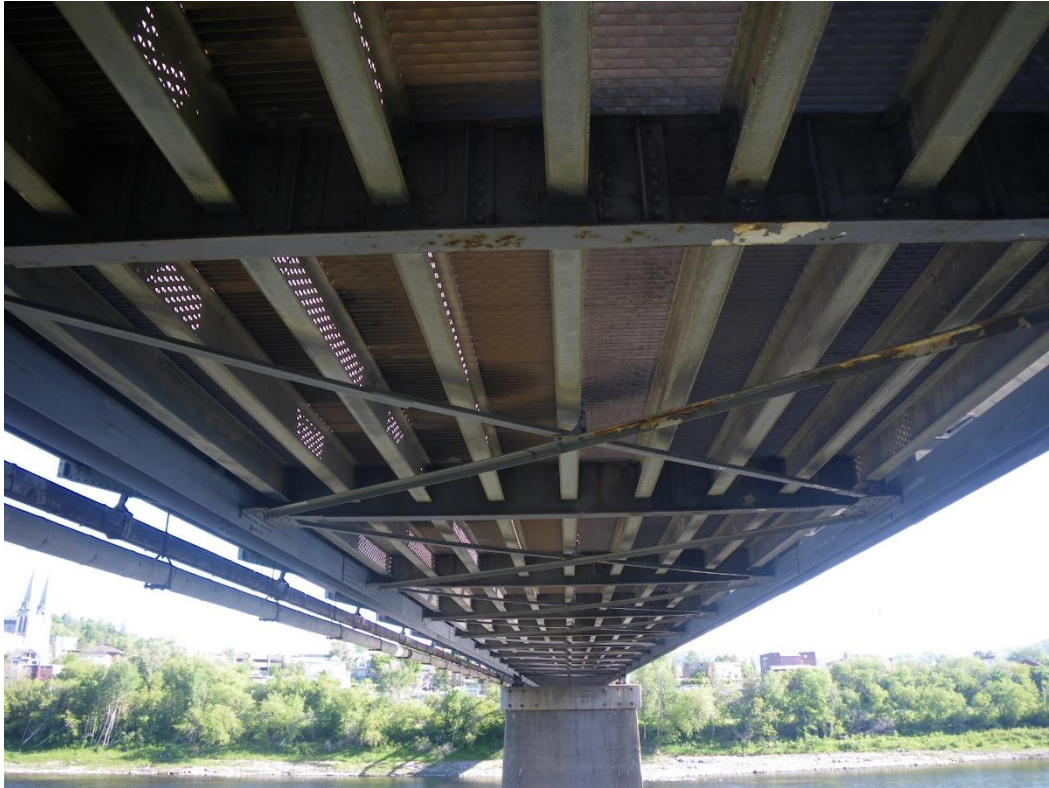
Photo 7: Underside of Span 4 near South Abutment, Looking North. Note areas of a failed paint system on the floorbeams.
