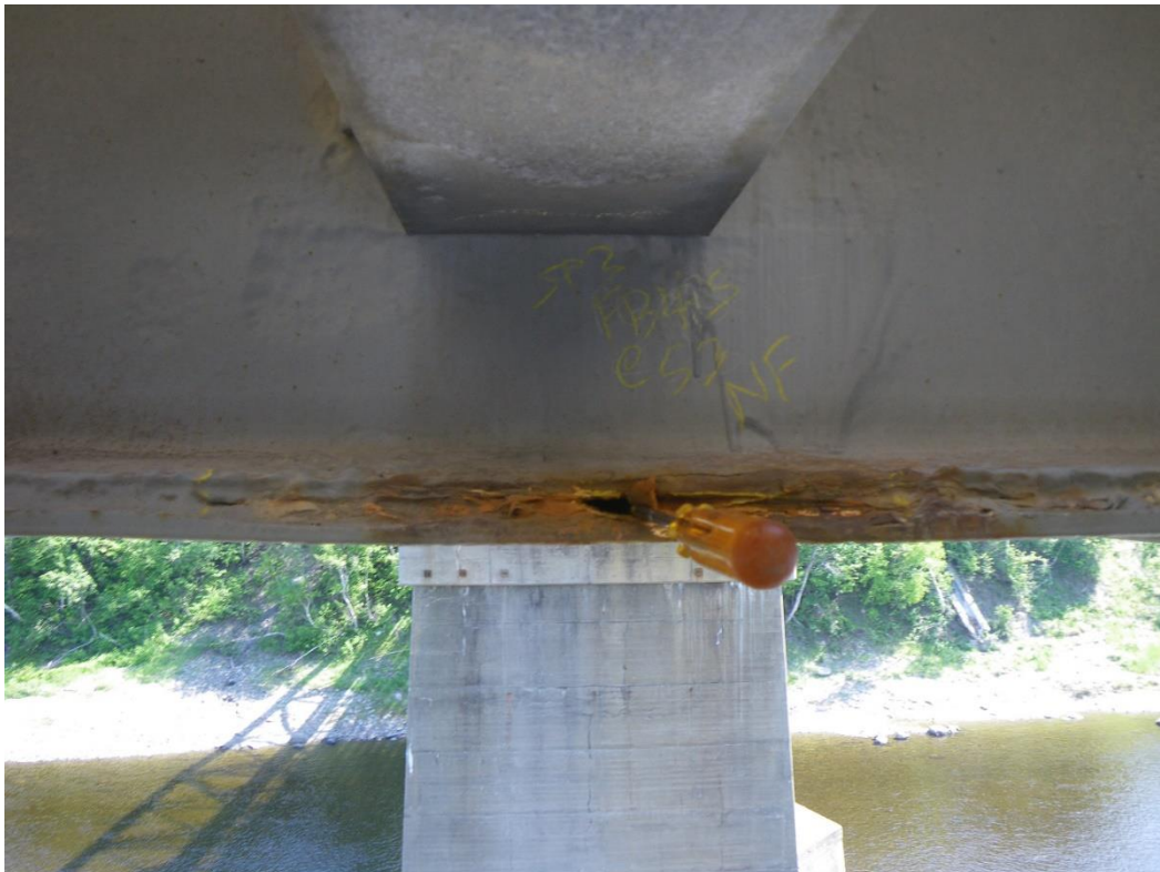
Photo 42: Floorbeam FB4S at Stringer S3, North Face, Span 3 - Bottom flange cover plate weld with crack/separation and gap.
