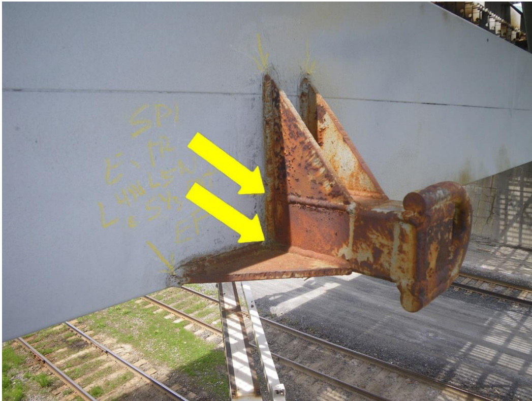
Photo 57: Lower Chord L4NL5N at South Third Point, East Face, East Truss, Span 1, Looking Northwest - Intersecting welds of the abandoned anchor point on the flange angles.
