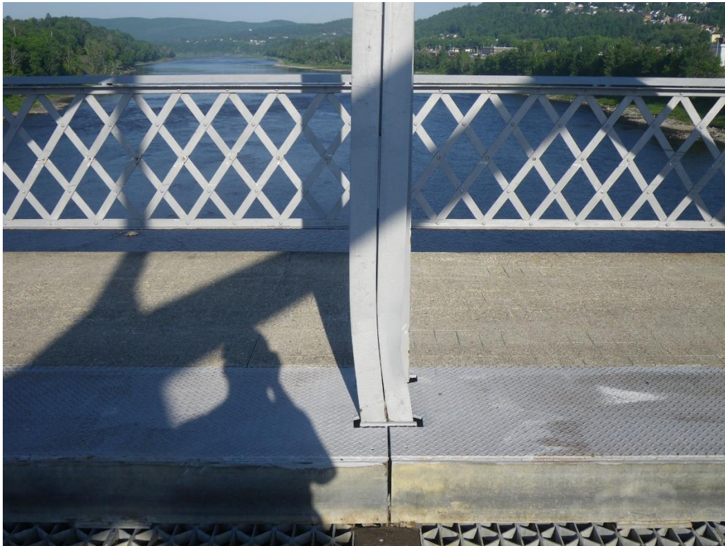
Photo 43: Vertical U3NL3N near Curb, East Face, West Truss, Span 3 - Flange angles with sweep, rotation and bend due to collision damage.
