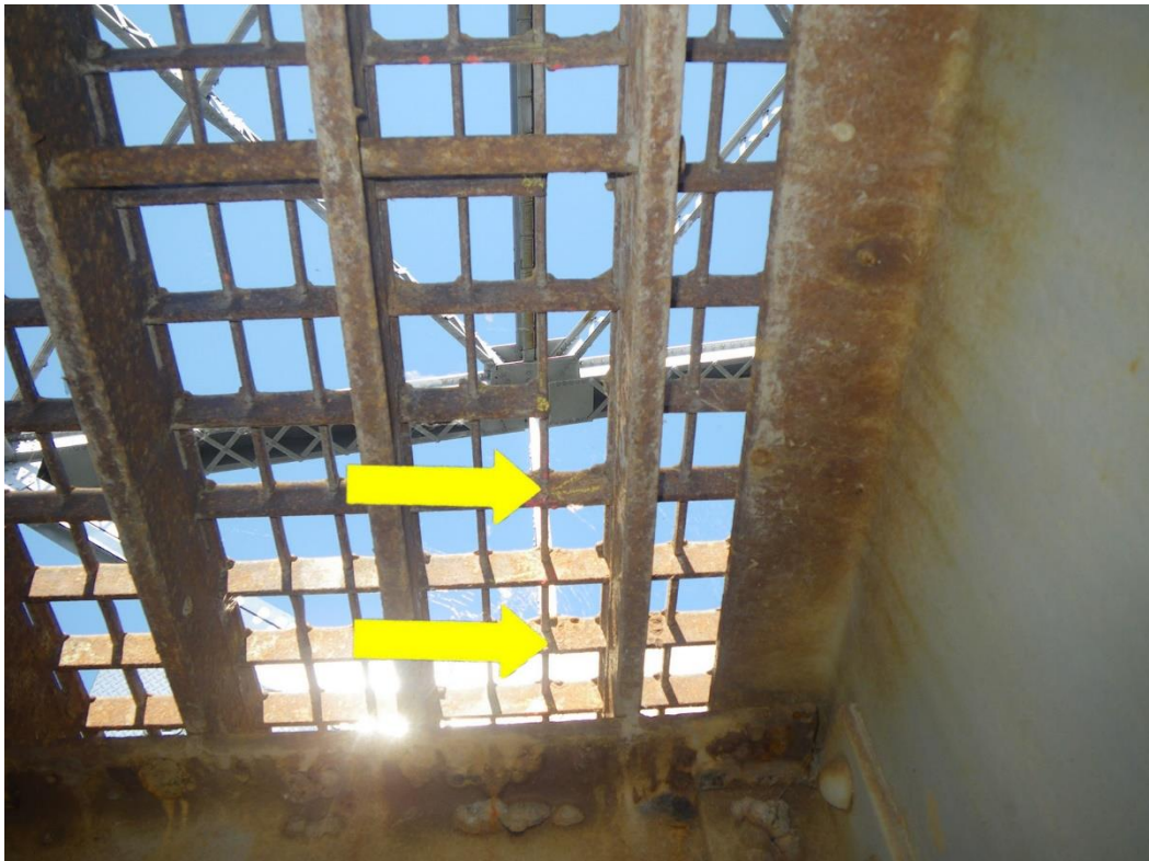
Photo 14: Deck between Stringers S2 and S3, at South Side of Floorbeam FB3S, Span 1, Looking West - Transverse distribution bars with full height cracks or missing sections.
