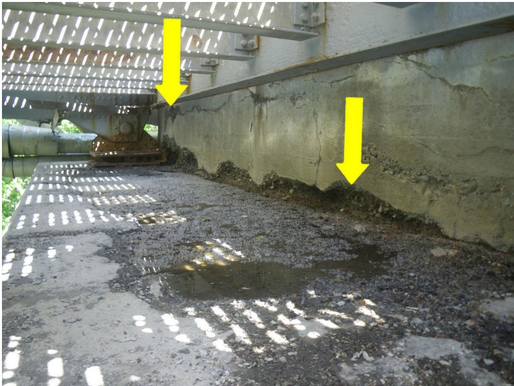
Photo 58: South Abutment Backwall between East and West Trusses, Looking East - Spalling and map cracking with moisture.
