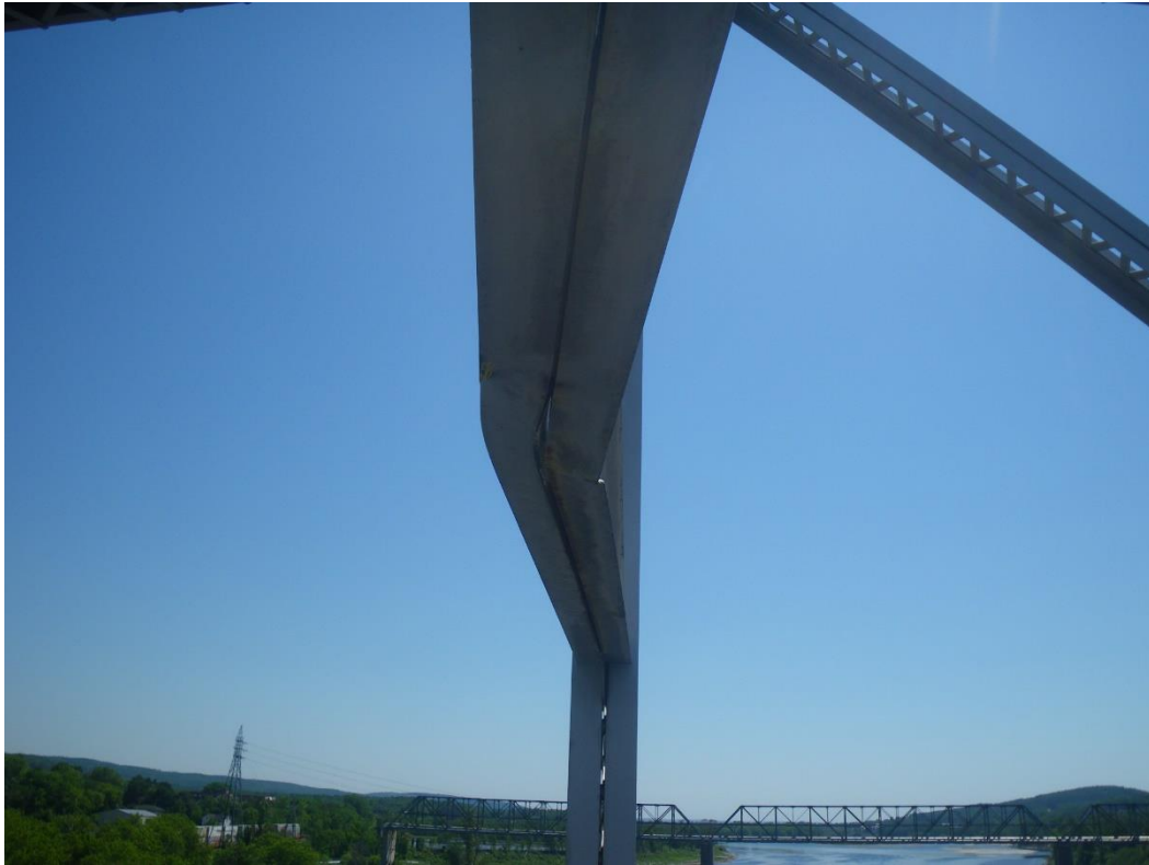
Photo 45: Sway Bracing Lower Horizontal Strut above Northbound Lane, Panel Point 4N, Span 2, Looking East - Flange angles with sweep and bend in outstanding leg due to collision damage.
