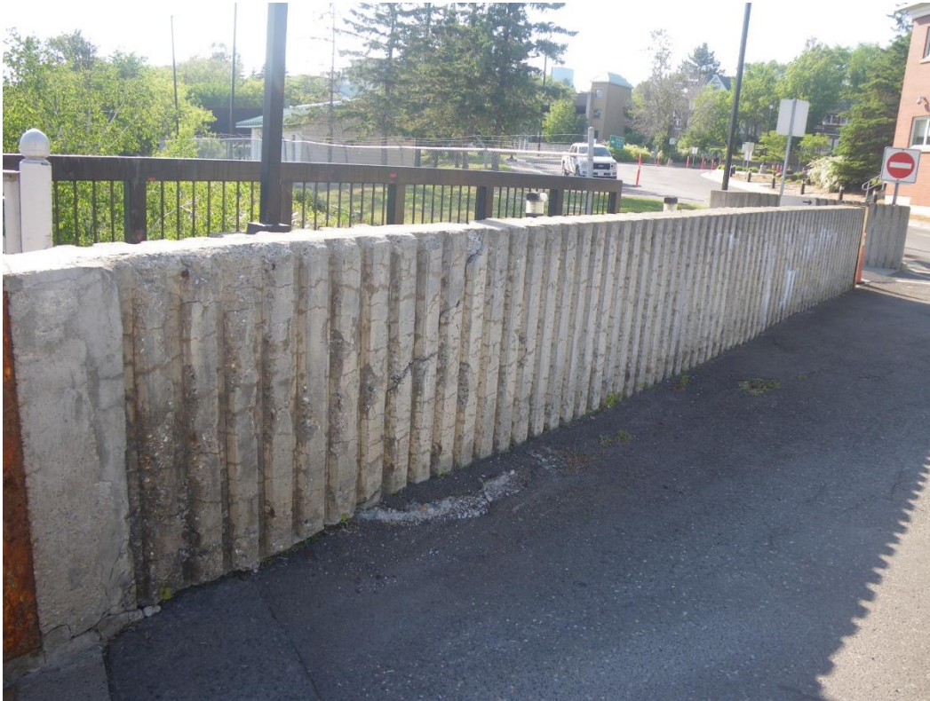
Photo 61: Northwest Traffic Barrier near North End, East Face, Looking Northwest - Extensive map cracking with moisture and efflorescence, diagonal crack, delamination and spalls.
