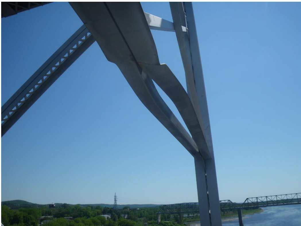
Photo 46: Sway Bracing Lower Horizontal Strut above Northbound Lane, Panel Point 4S, Span 2, Looking East - Flange angles with sweep, twisting, separation between back to back vertical legs and upward bend in outstanding leg due to collision damage.
