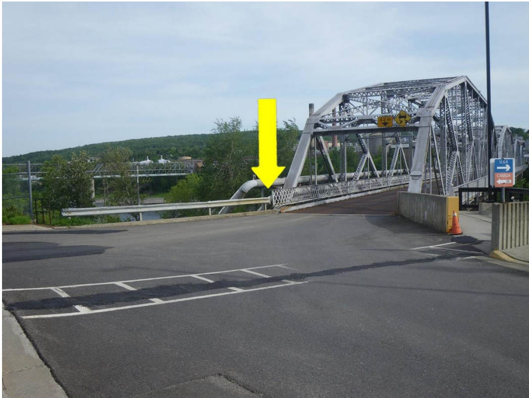
Photo 3: North Approach, Looking Southeast. Note "At-Bridge" vertical clearance sign, no "At Bridge" bridge load posting sign and no connection of east bridge railing to approach guardrail.
