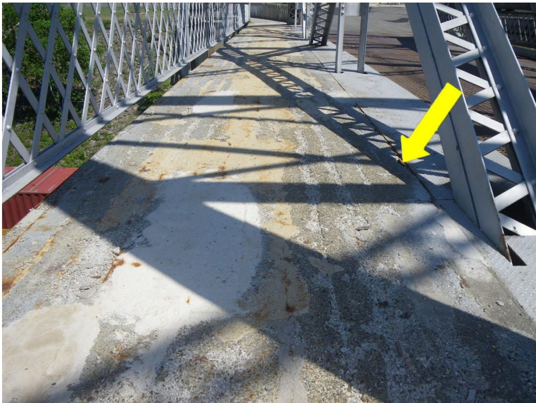
Photo 18: Top of Sidewalk between Panel Points L3N and L4N, Span 1, Looking North - Thin concrete patch layer not covering full width of sidewalk, exposed distribution bars with rust, scaling, full depth spalling along curb and previous repairs.
