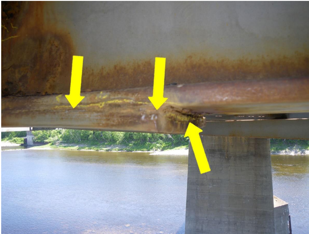
Photo 41: Floorbeam FB5S between Stringers S8 and S9, North Face, Span 2 - Impacted rust between the bottom flange and cover plate. Note weld between bottom flange and cover plate extends to cover plate edge and is cracked.
