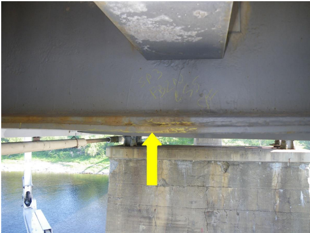
Photo 40: Floorbeam FB1N at Stringer S5, South Face, Span 3 - Bottom flange cover plate with bend. Note gap in weld between bottom flange and cover plate.
