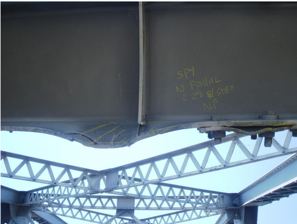
Photo 48: Portal Bracing Lower Transverse Brace above SB Lane, North Face, North Portal, Span 1 - Bottom flange with bend and gouge, bent and detached web stiffener and bent connection plate due to collision damage.
