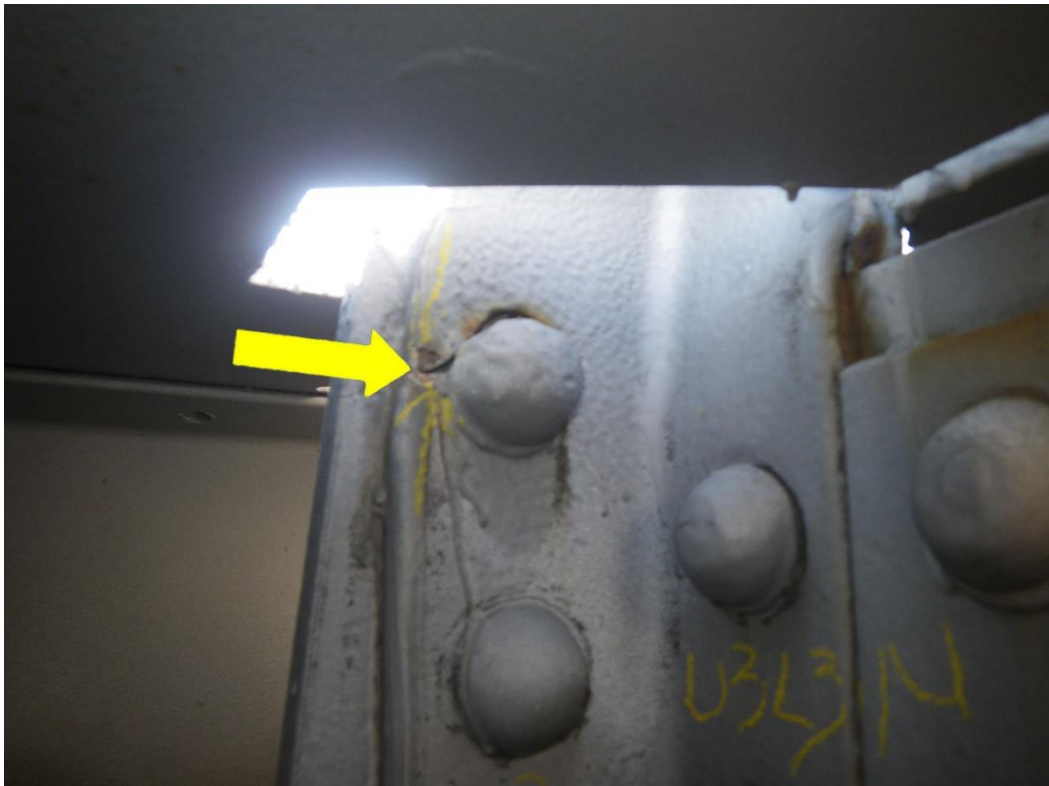
Photo 44: Vertical U3NL3N at Panel Point L3N, West Face, West Truss, Span 3 - Crack in outstanding leg of flange angle due to collision damage above the curb and section loss along the edge of the drilled hole.
