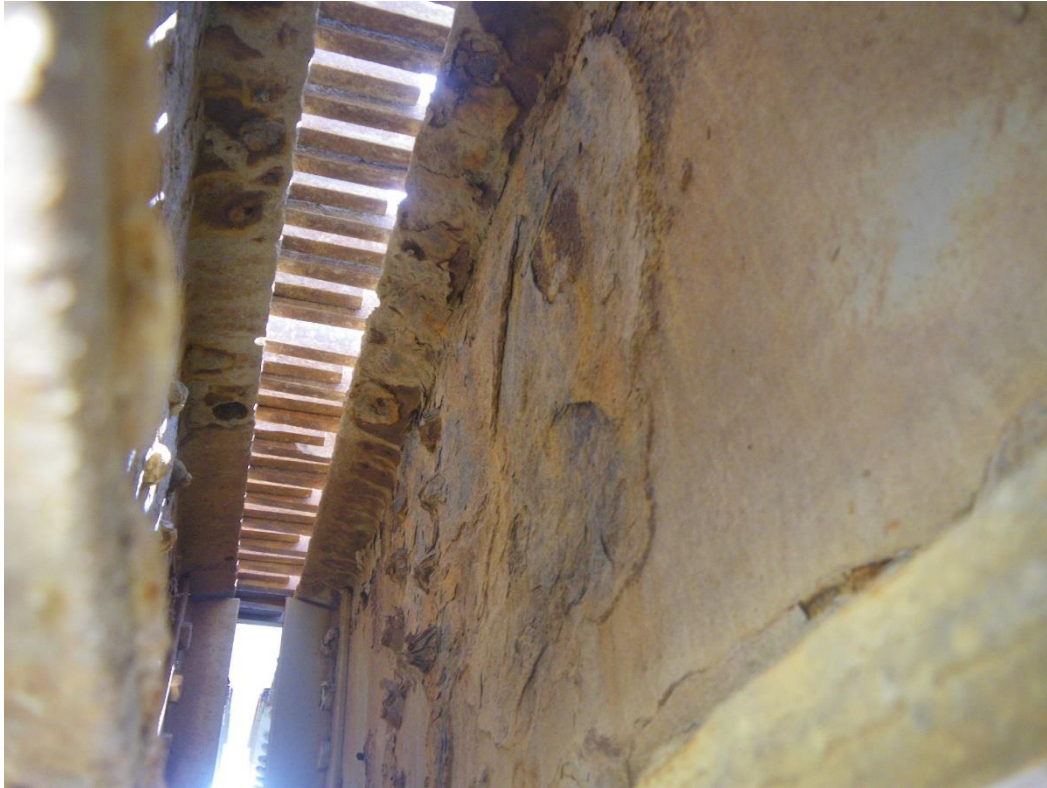
Photo 31: Floorbeam FB0N between Stringers S2 and S3, South Face, Span 2, Looking West - Web section loss. Note failed paint system.
