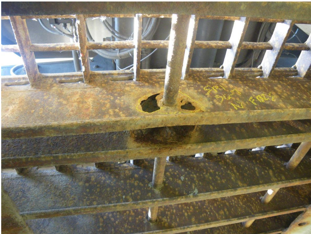
Photo 16: Deck between Stringers S6 and S7, at 3'-6" North of Floorbeam FB2S, Span 1, Looking South - Transverse bearing bar with area of 100% section loss around the longitudinal circular diaphragm bar.
