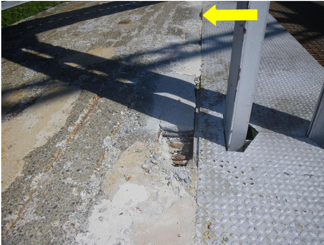
Photo 19: Top of Sidewalk at Panel Point L3S, Span 1, Looking North - Exposed top of distribution bars with surface rust, scaling, full depth spall and previous repairs.
