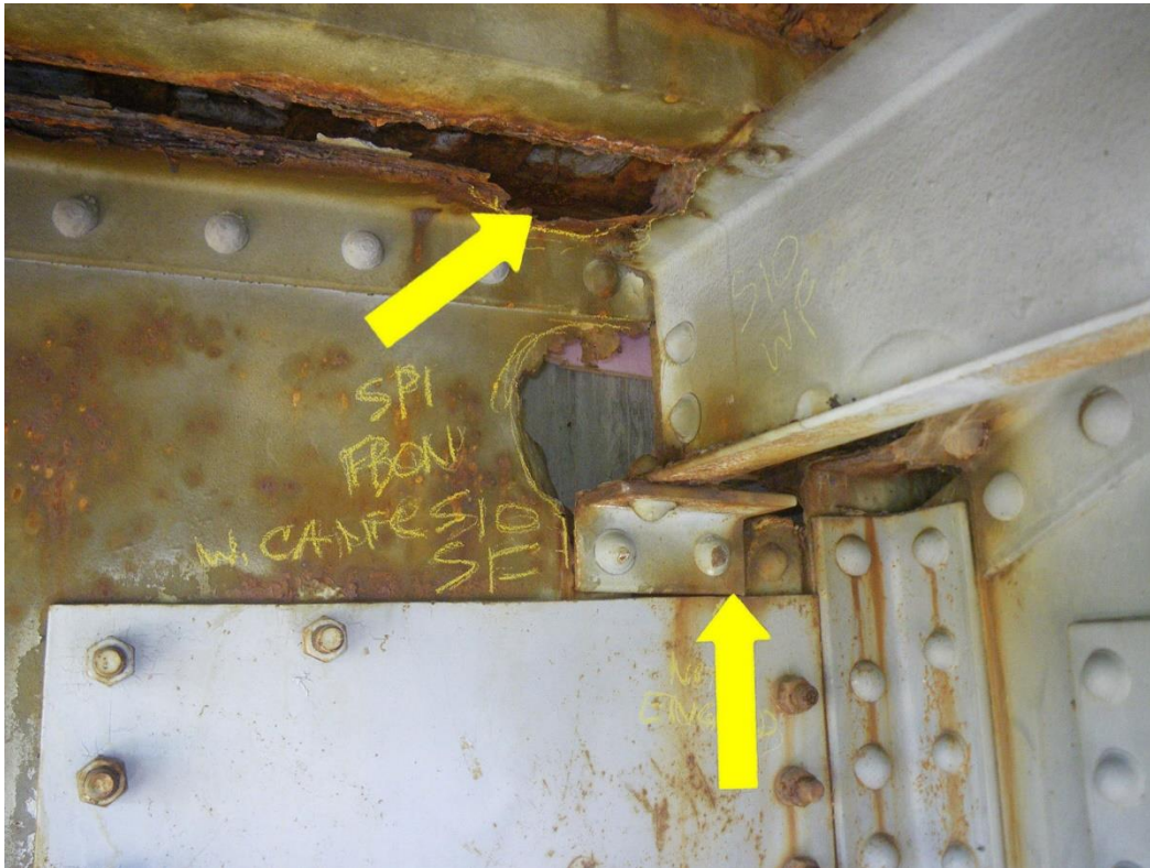
Photo 29: Stringer S10 at Floorbeam FB0N Cantilever, South Face, Span 1 - Not connected to floorbeam web due to 100% section loss of floorbeam web. Note rotated stringer seat angle and 100% section loss of the floorbeam cantilever top flange.
