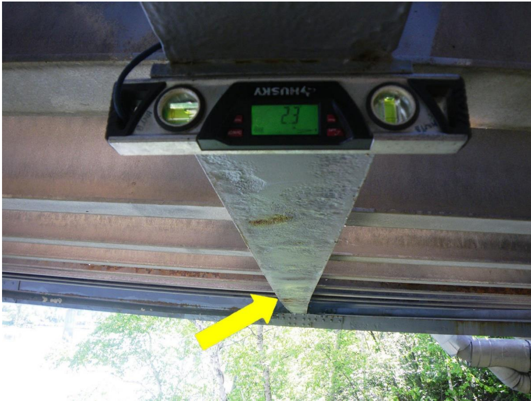
Photo 39: Floorbeam FB1S between Stringers S8 and S9, Span 4, Looking East - Bottom flange cover plate section loss and rotation. Note floorbeam sweep.
