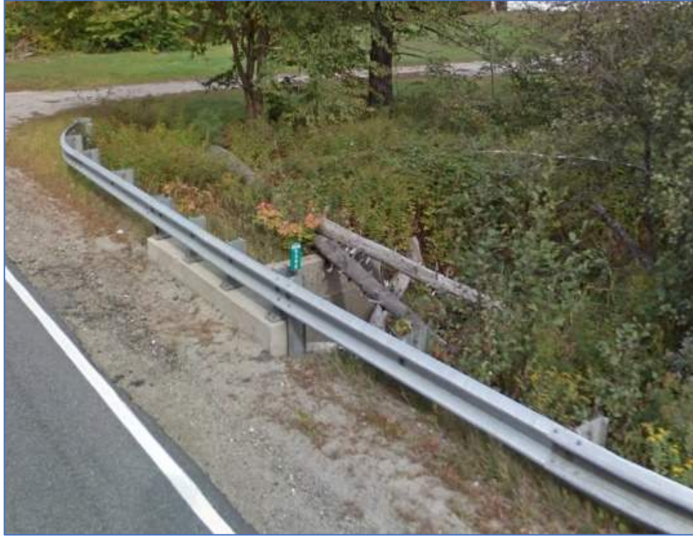
Figure 6 - Fallen Trees on Top of Inlet Wingwall (Google Streetview image captured Sept 2016)
