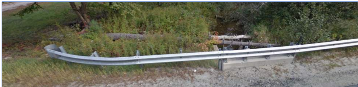
Figure 5 - Fallen Trees on Top of Inlet Wingwall (Google Streetview image captured Sept 2016)
