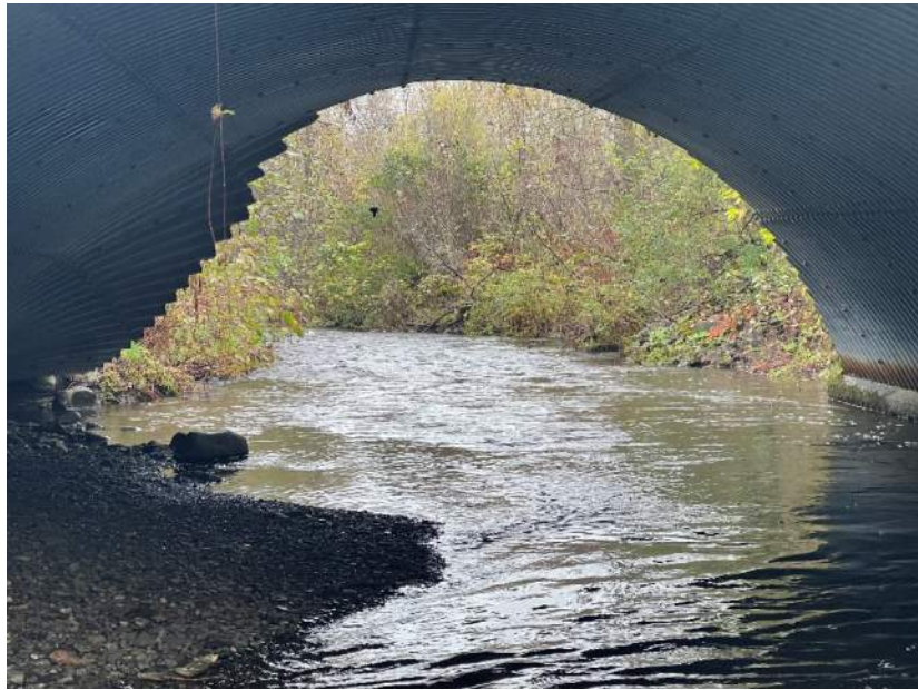
Photo 7: Looking downstream through Bridge 5309 at sediment buildup.
