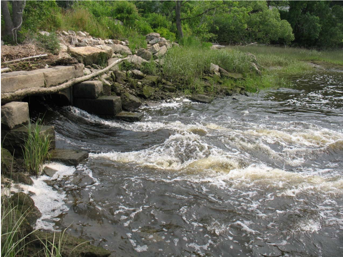
Figure 2 Culvert underneath George Wright Road. Photo taken downstream of Back River Marsh.
