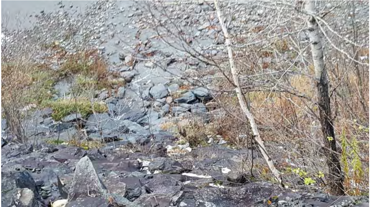
Figure 9. Example of steep bank and riprap protection on U.S. side of St. John River, upstream of International Bridge
