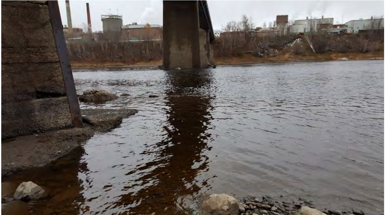
Figure 11. Piers of International Bridge, note triangular nose and apparent ice damage.
