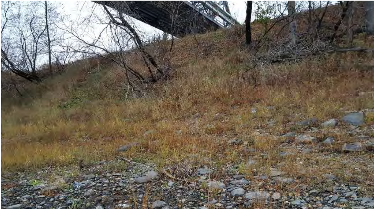
Figure 10. Steep bank below Abutment on Canadian side of International Bridge.
