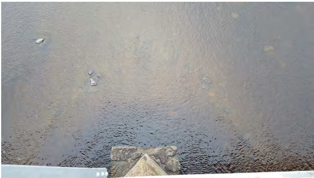
Figure 33. Note scour hole at nose of pier of existing bridge
