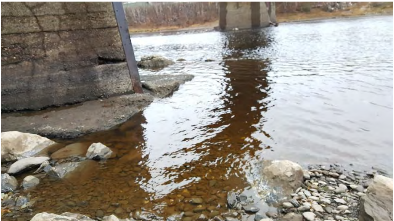
Figure 35. Pier shows evidence of scour at base as well as pointed nose shape with ice/debris protection
