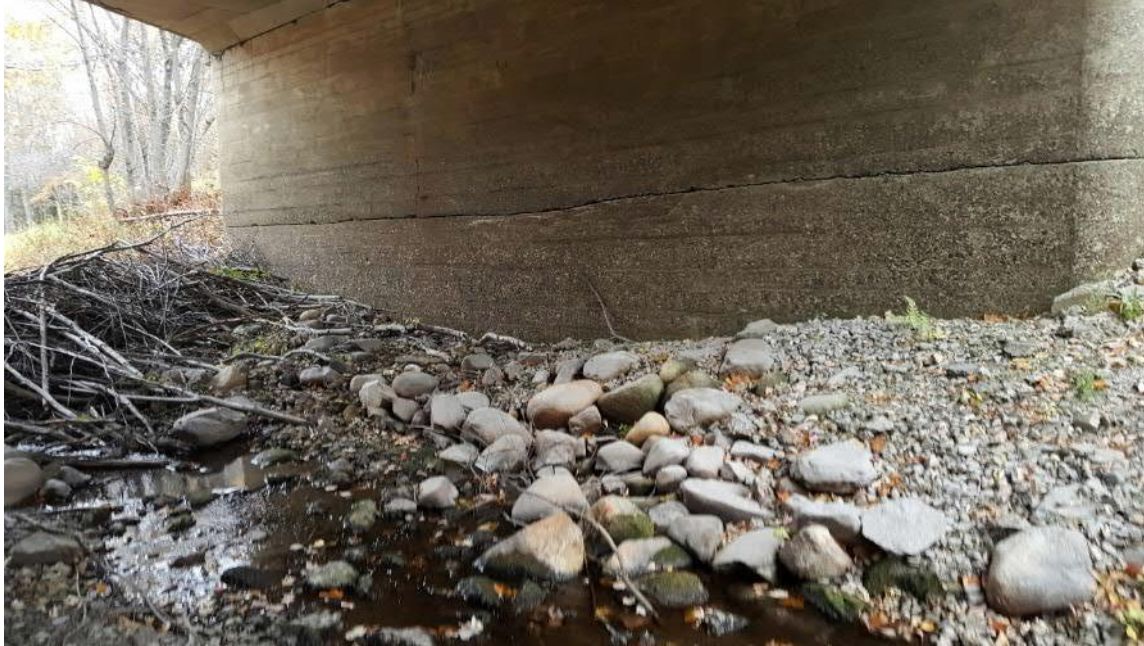
Figure 21. Center channel. Note scour hole along center of pier.
