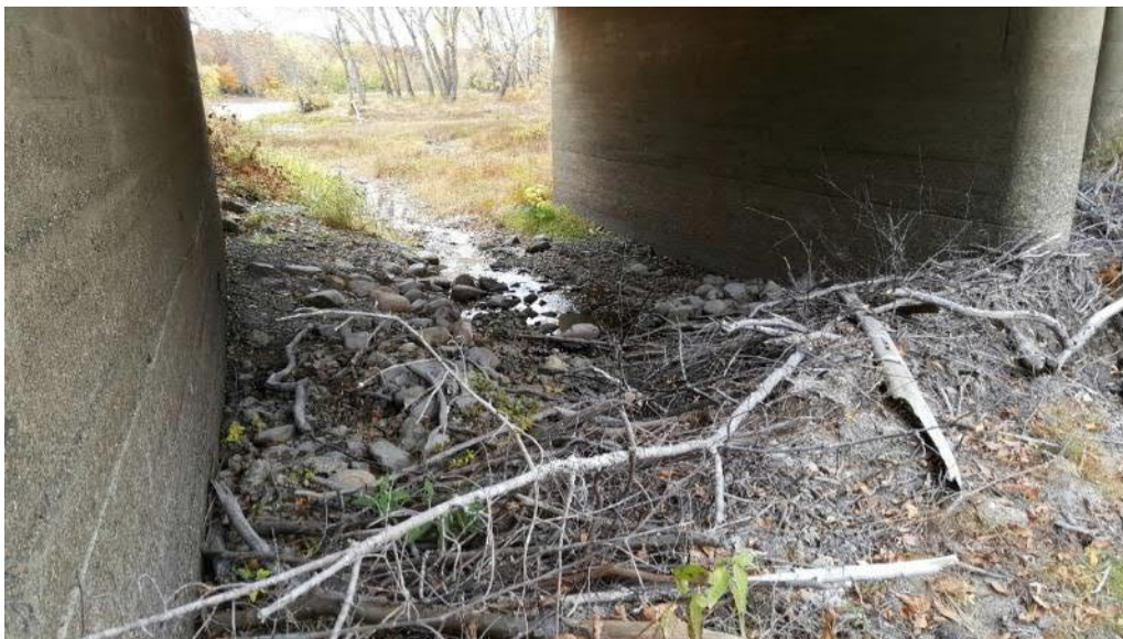
Figure 20. Center channel of existing bridge looking downstream from beaver dam. Note large stones in channel and erosion near piers.
