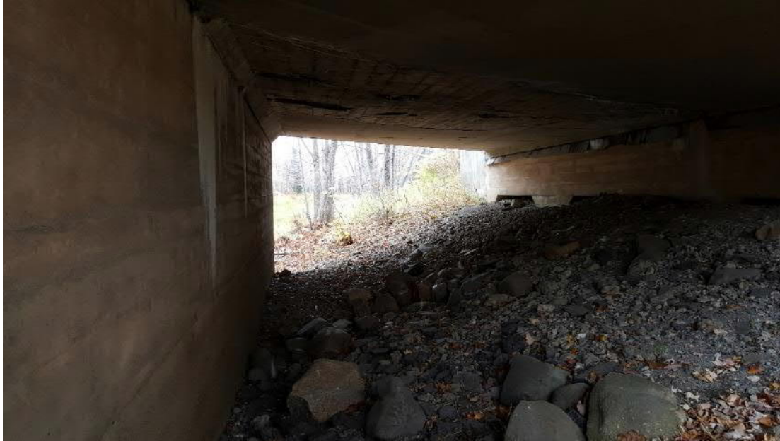
Figure 19. South channel of bridge (looking upstream). Note large rocks and erosion near pier.
