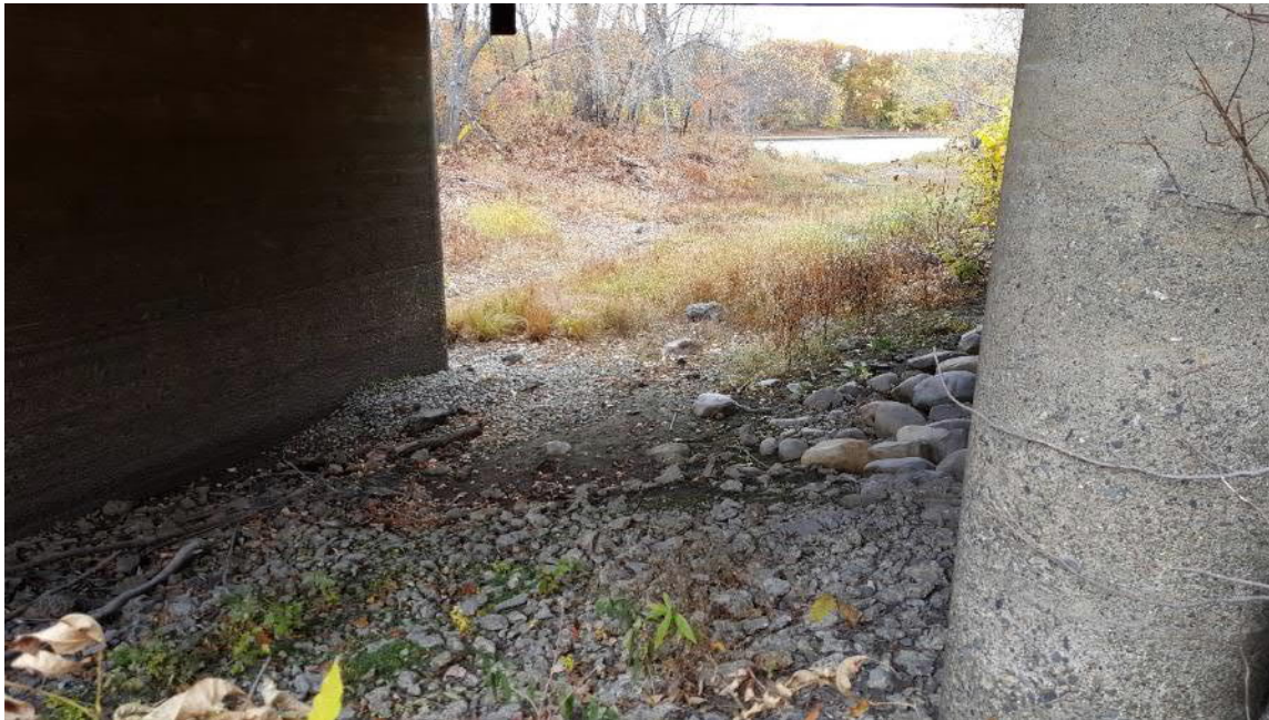
Figure 22. Center channel. Note large stones and scour along pier.
