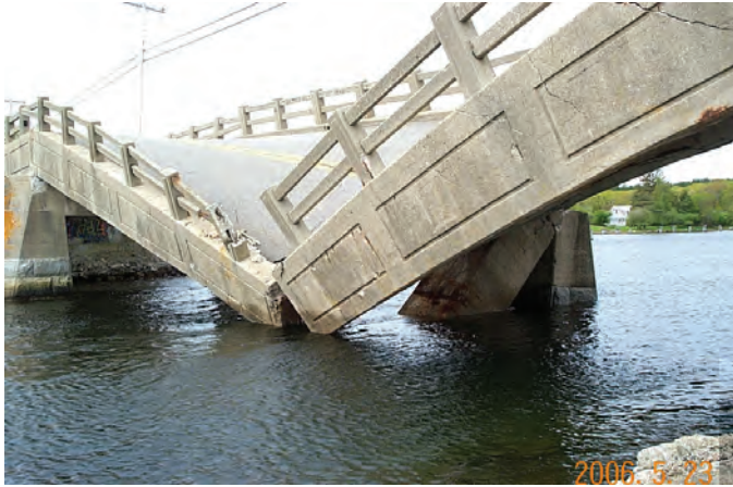
Figure 4. Bridge failure over Cape Neddick River, York County, Maine.
