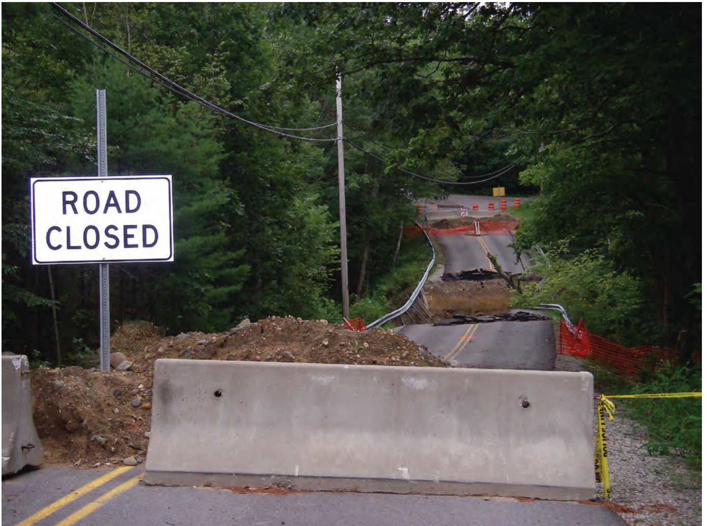
Figure 3. Logging road culvert failure over the Josias River, York County, Maine.
