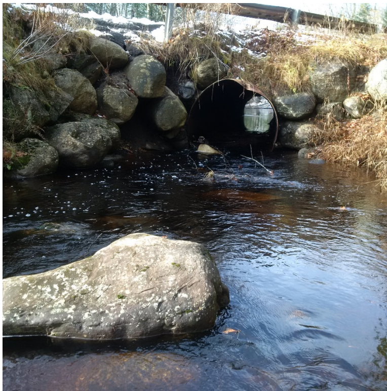
Photo 4. Culvert outlet and scour pool (A. Walsh 11/23/2015).
