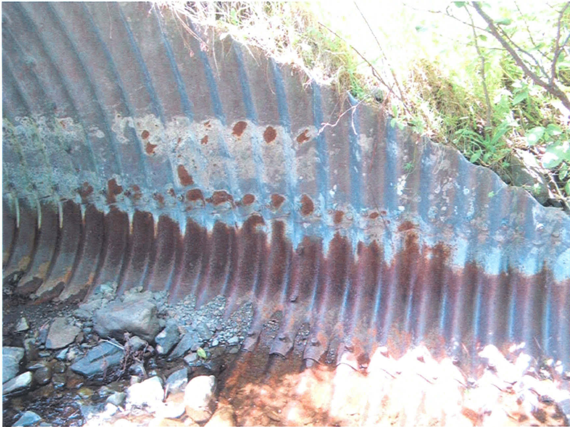
Figure 7: Upstream rust line
