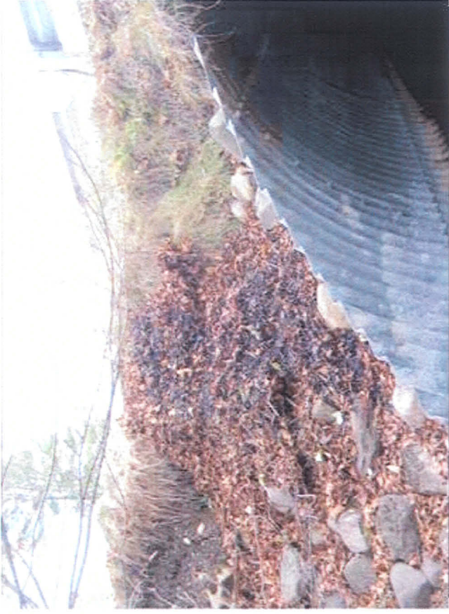
Upstream East side banking from stream to roadway is heavily eroded
