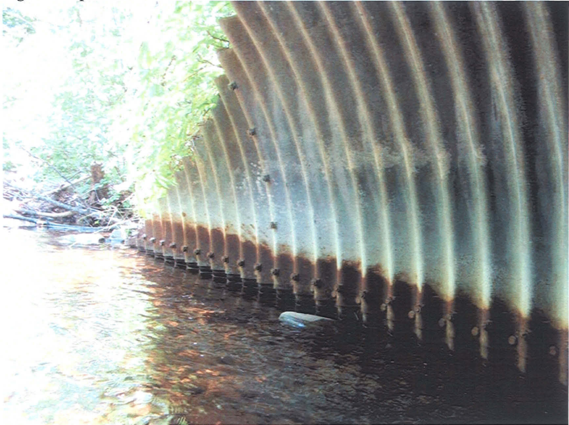
Figure 8: Downstream rust line
