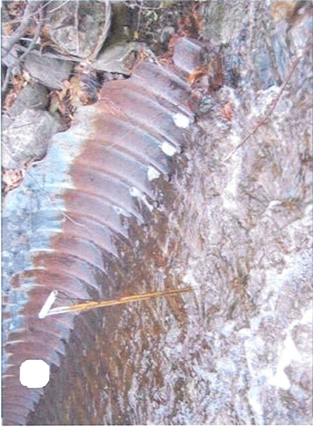
Large elongated holes were found and could be made with probe across bottoms of ribs at upstream end up to 4' into pipe
