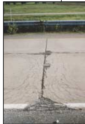
FIGURE 53 Distress Type JCP 2—High Severity “D” Cracking with Loose and Missing Material
