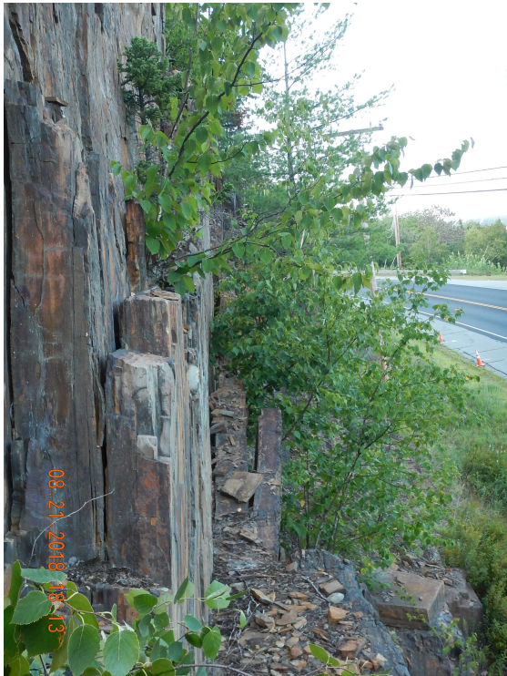
PHOTO 2 (ABOVE): SIDE VIEW (LOOKING NORTH) WITH OPEN BACK JOINT VISIBLE
