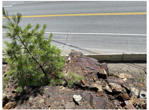
PHOTO 2 (ABOVE): TOP VIEW WITH SOIL FILLED BACK JOINT VISIBLE.
