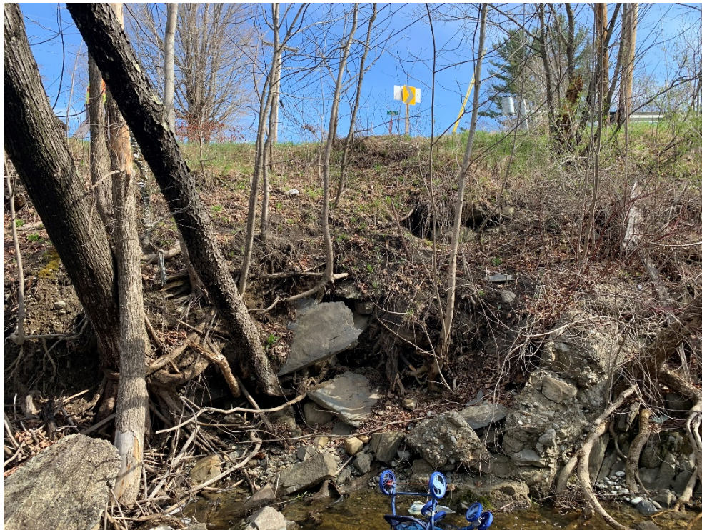
Photo 1: Slope between Fall Brook and Cross Road, approximately STA 400+50, evidence of soil loss due to probable piping erosion can be seen in the middle and toe of the slope.
