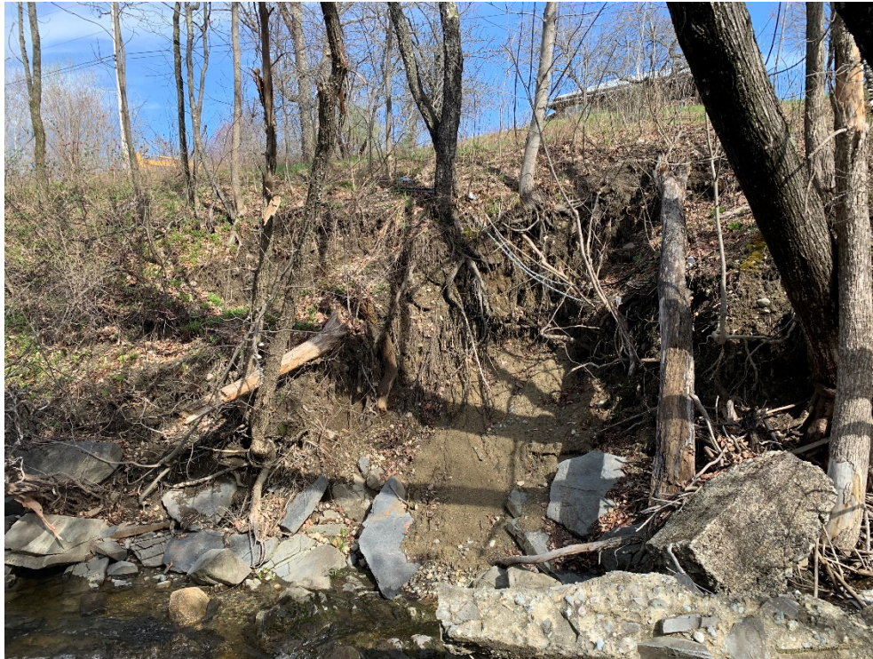
Photo 2: Slope between Fall Brook and Cross Road, approximately STA 400+75, surficial slough-type failure of the slope that may have been exacerbated by pipping erosion and tree loss.
