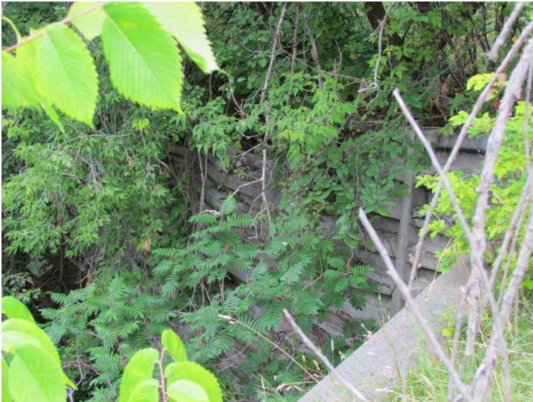
Buckled portion of bin wall
