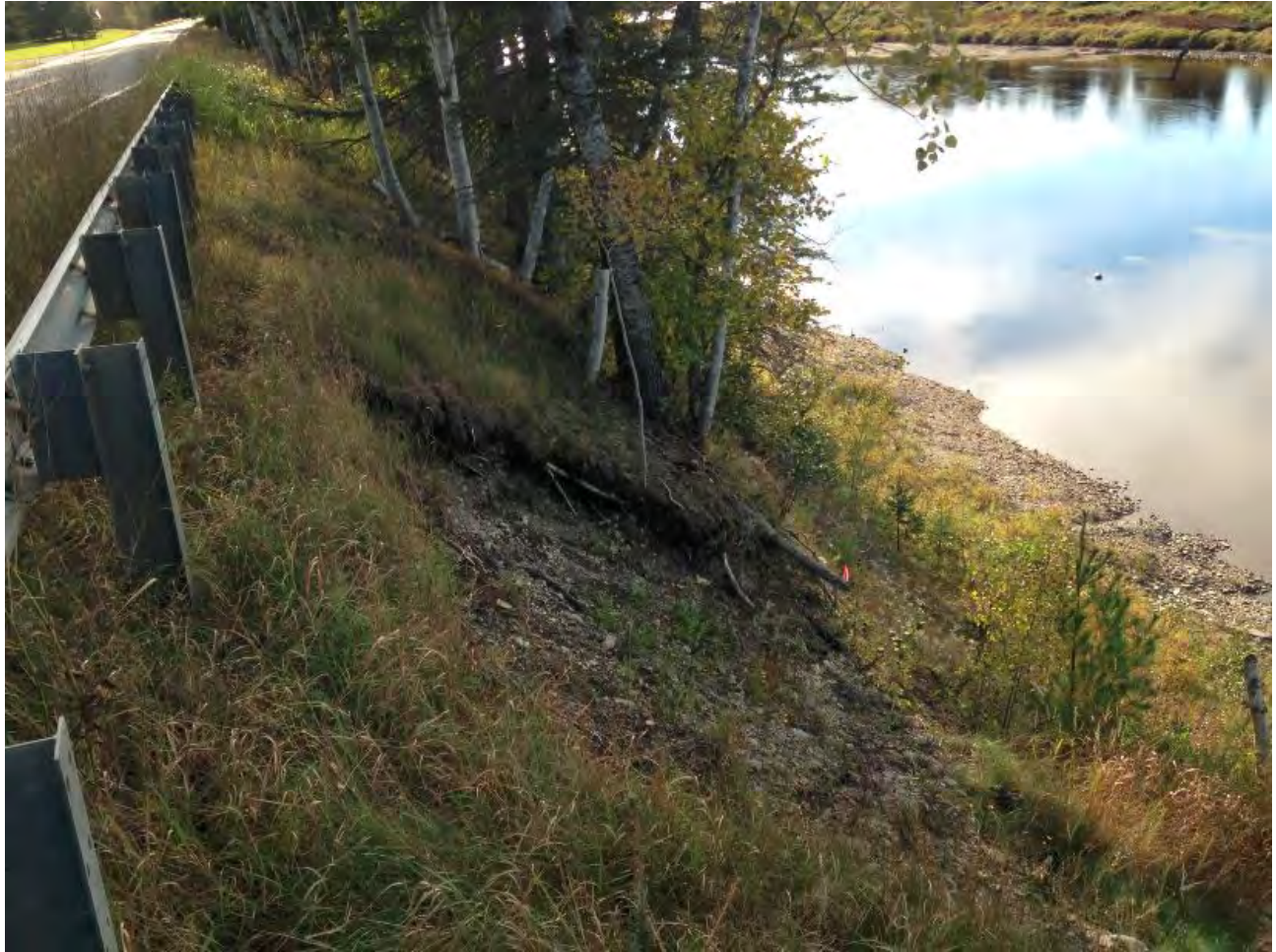
Figure 2. Planar slip bank failure at the top of the bank at the Allagash site.
