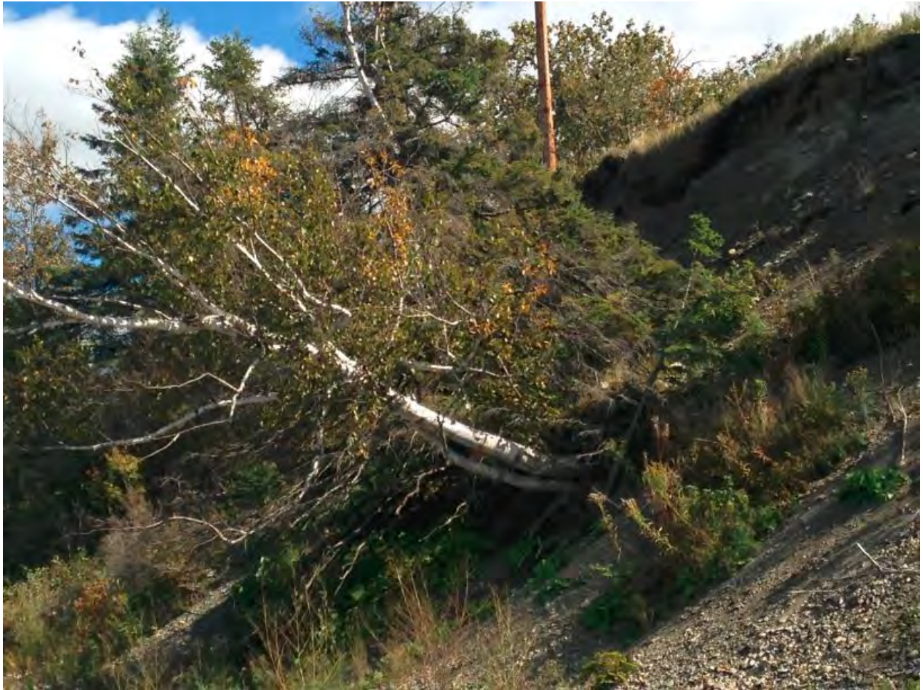
Figure 6. Leaning tree and vertical head scarp (at top of bank) are evidence of recent erosion at the St. Francis site.
