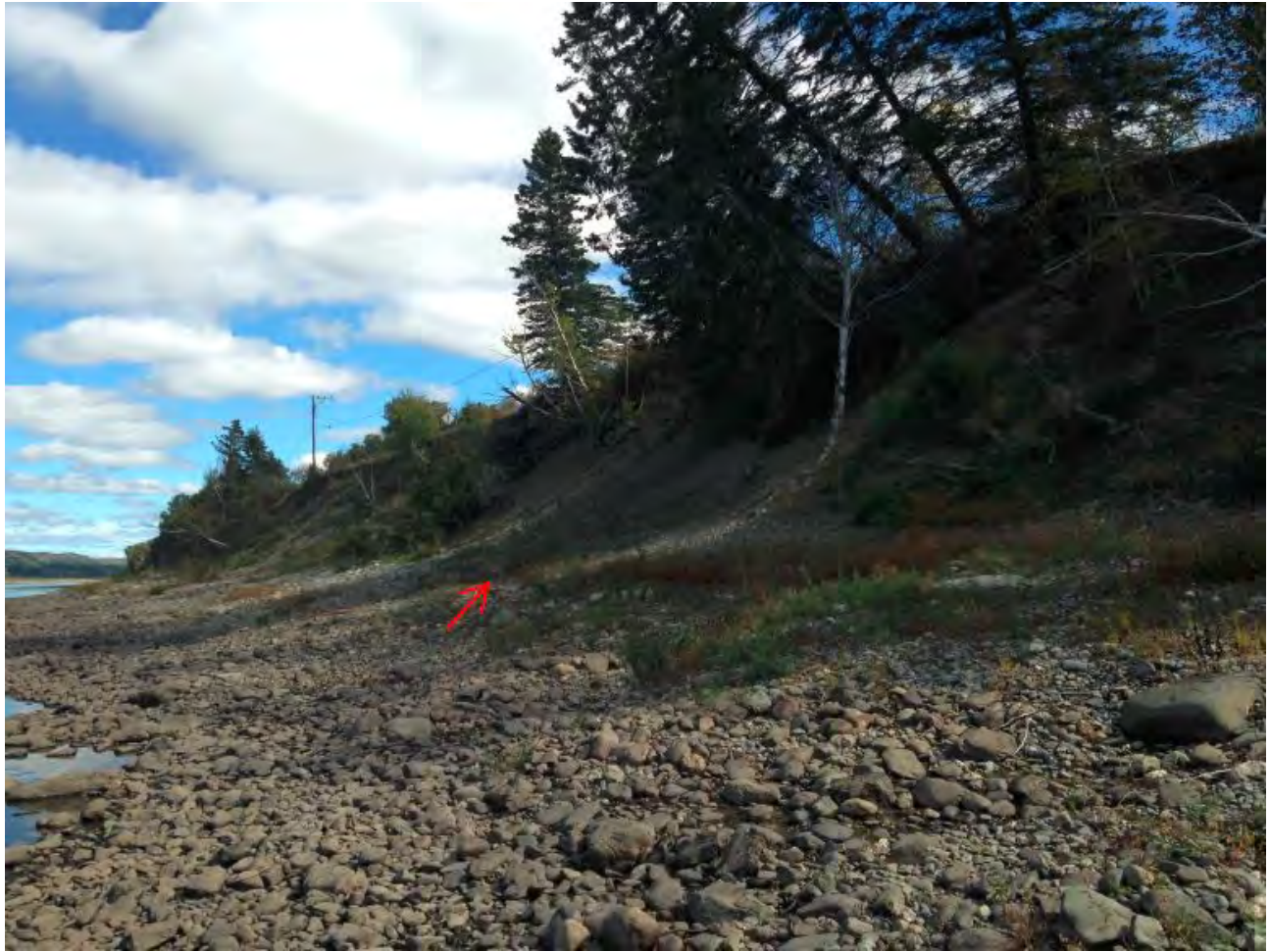
Figure 5. Eroding bank at St. Francis site.
