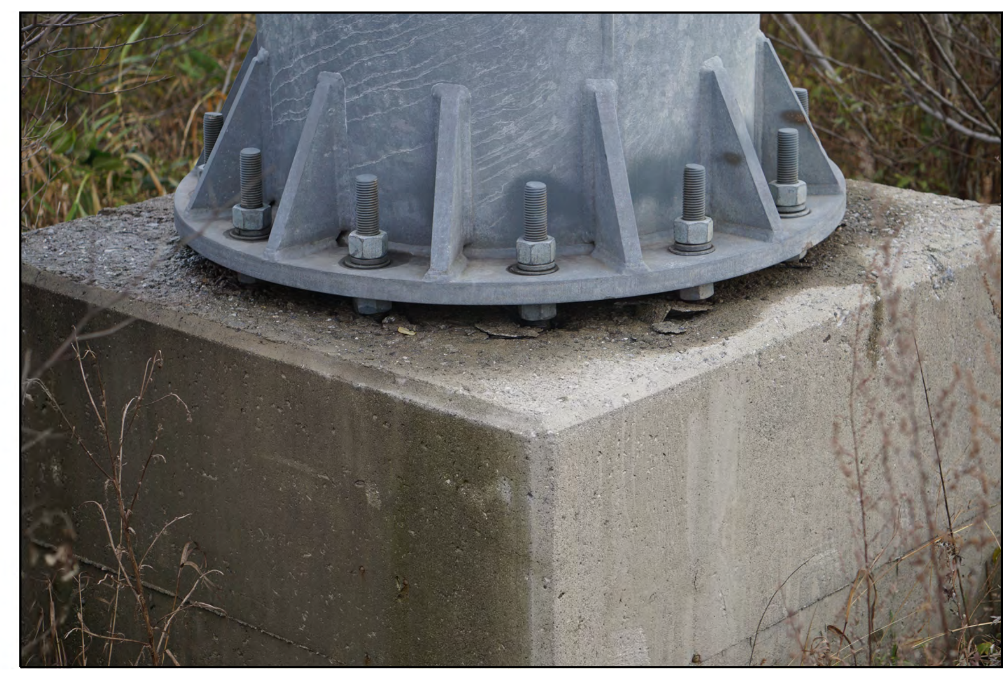
DAMAGE PHOTO - FOUNDATION VIEW
