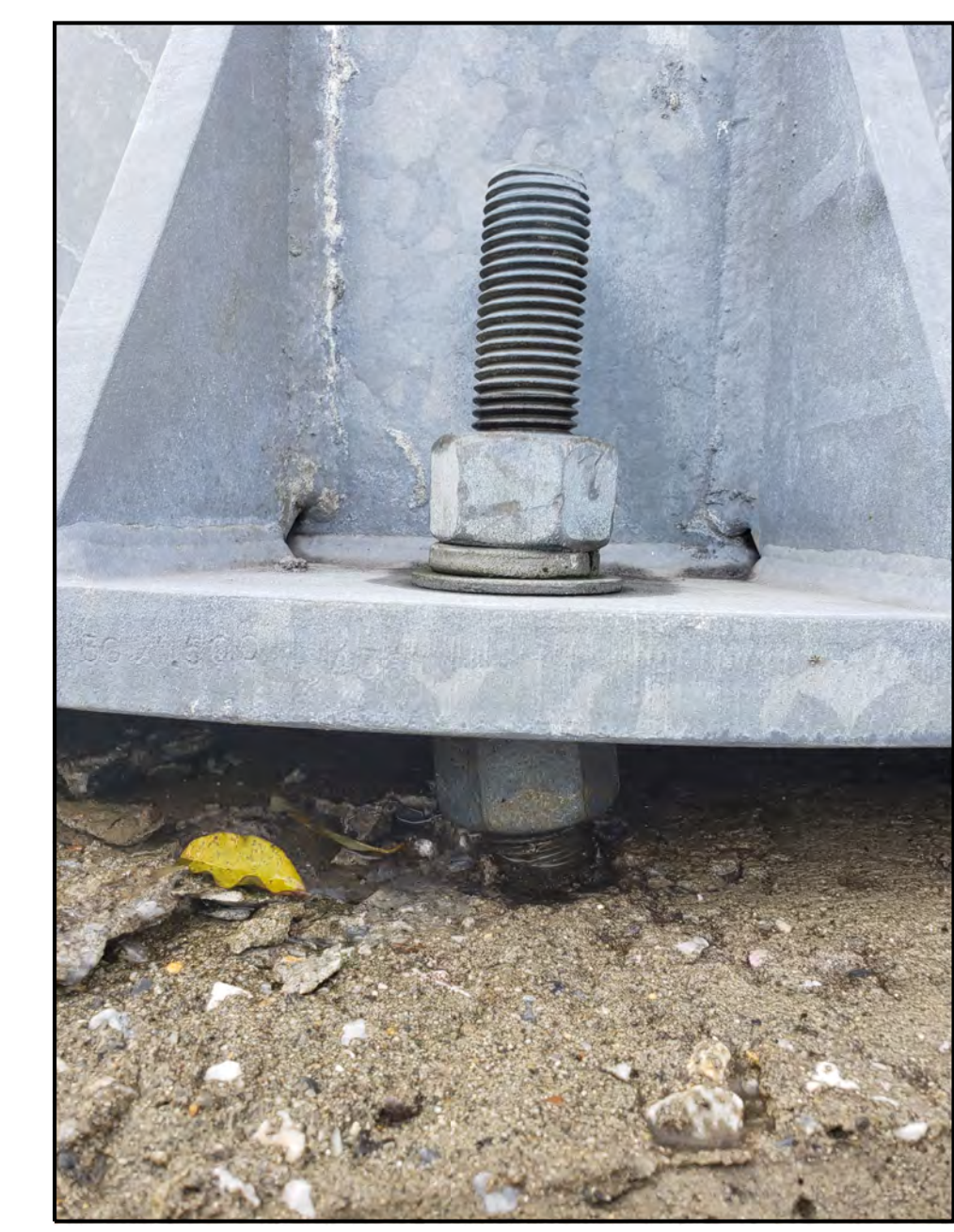
DAMAGE PHOTO - ANCHOR VIEW
