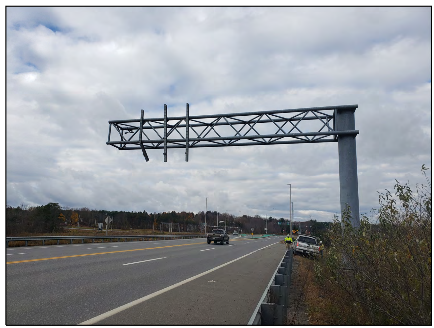
DAMAGE PHOTO - ELEVATION VIEW
