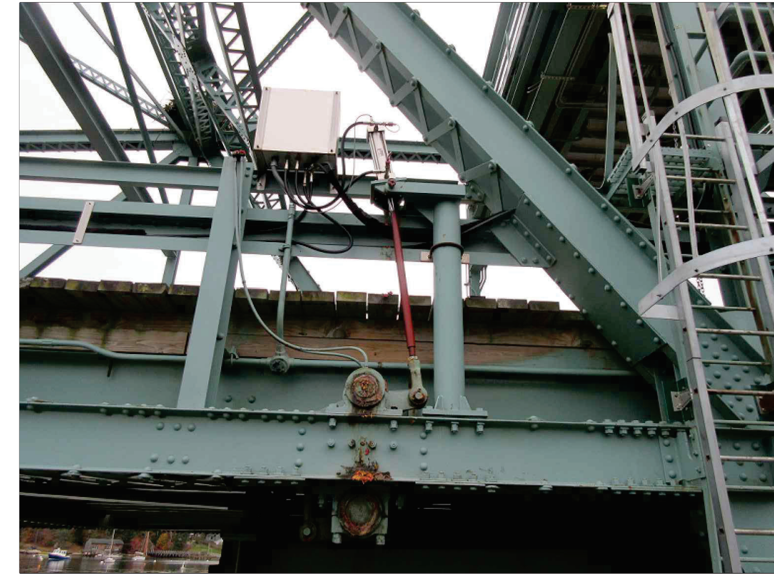
P5 CENTER WEDGE ACTUATOR & CONTROLS
