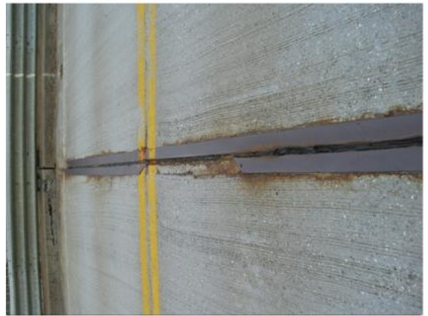
Joint seal missing and damaged armor
