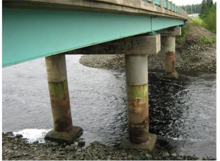
Steel piles with section loss of steel and exposed concrete
