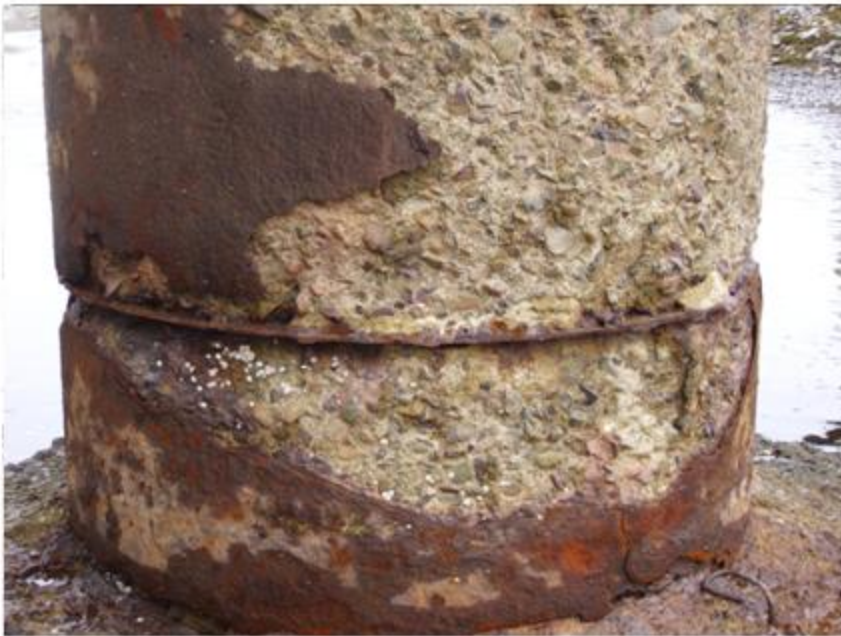
SE Pier Section loss
