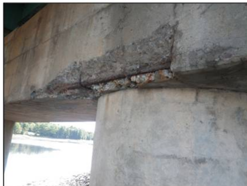
Spall concrete with exposed re-steel above column
