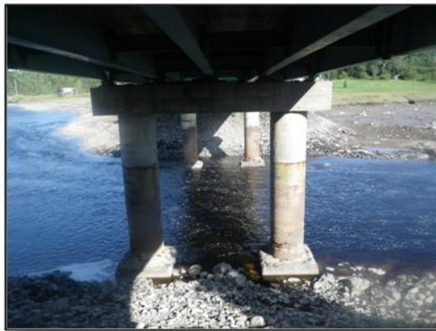
Scaling footings and section loss of steel protective casing of columns
