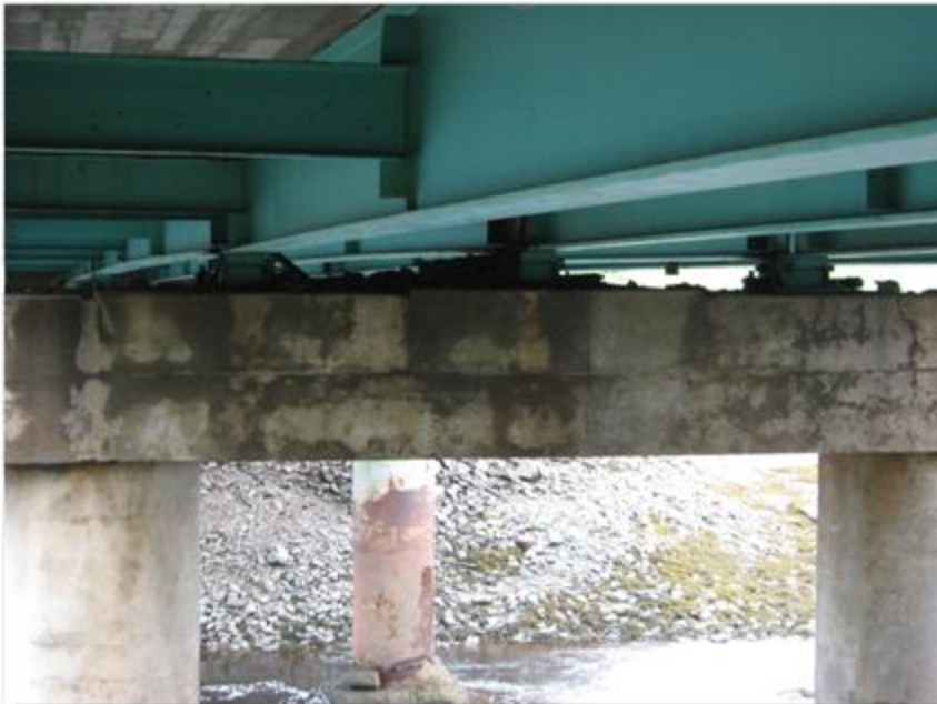
Concrete debris from haunches on pier cap
