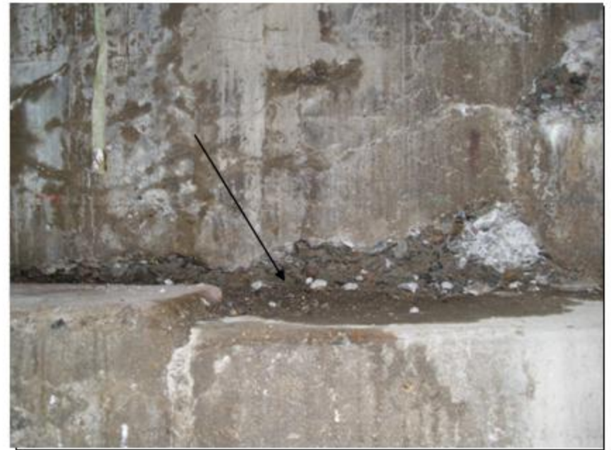
South Abutment Concrete spall 6" into Backwall
