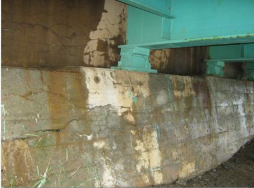
North abutment cracking
