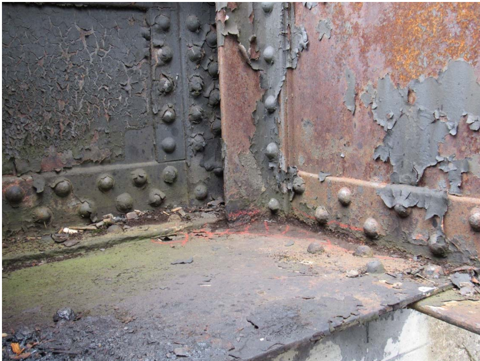
MP 139.56 – Fish River – Gusset Plate Deterioration
