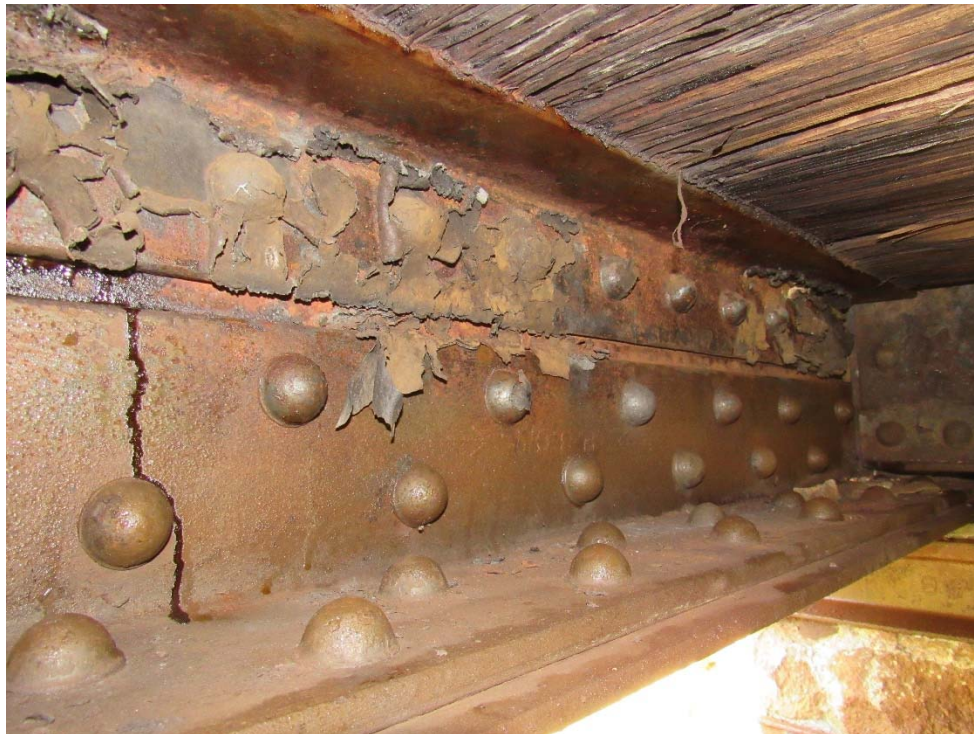
MP 154.59 – Dudley Brook – Typical Shelf Angle Assembly above Bottom Flange
