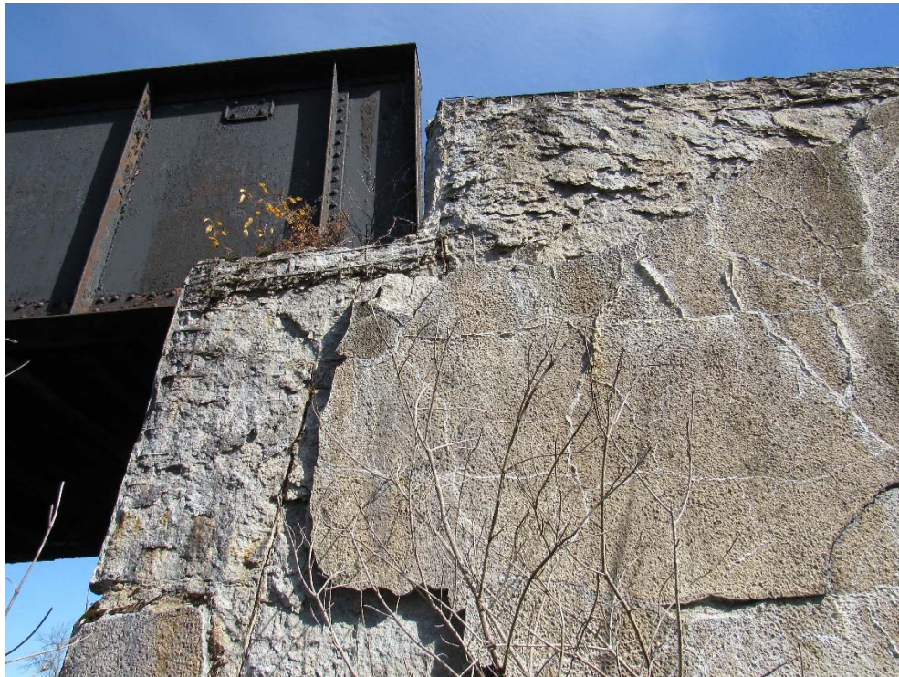
MP 236.44 – Wallagrass Stream – Deterioration at South Abutment Wingwall
