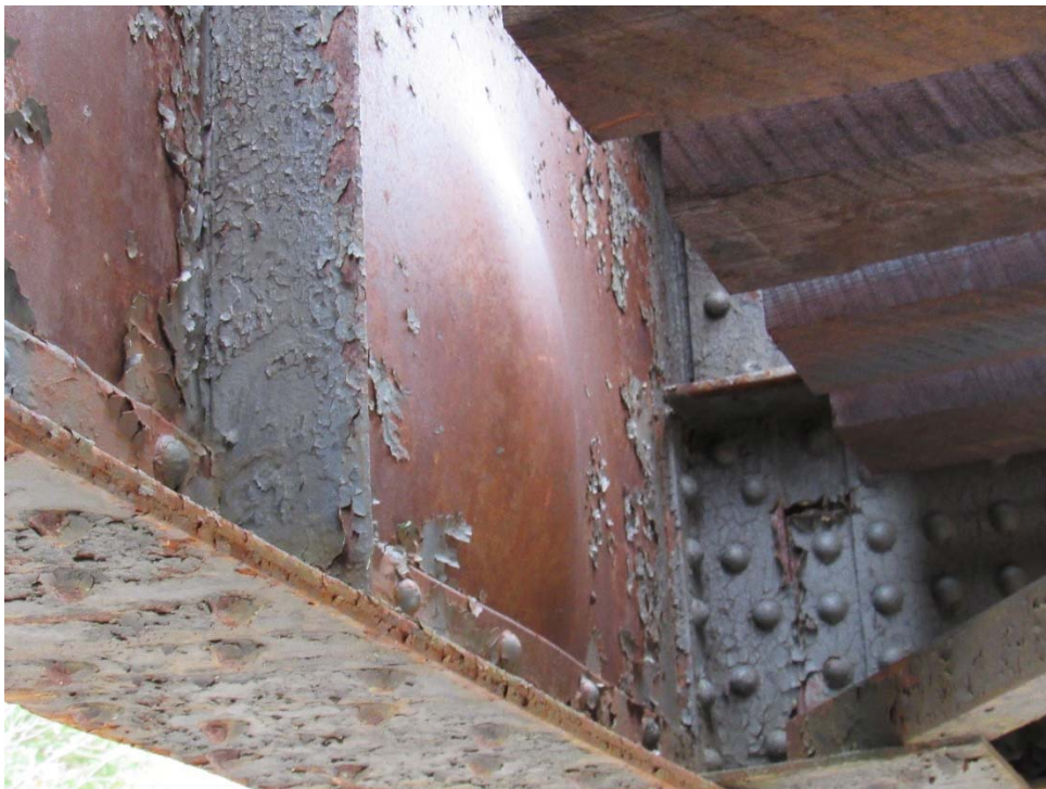
MP 113.14 – Grindstone Approach – Impact Damage
