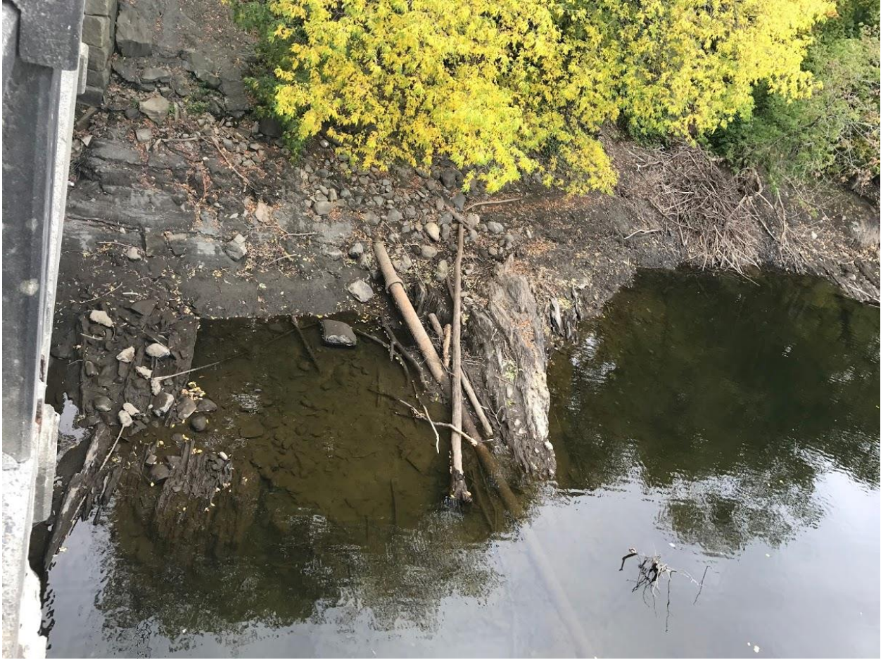
Looking at water main on upstream side of bridge near southerly abutment
