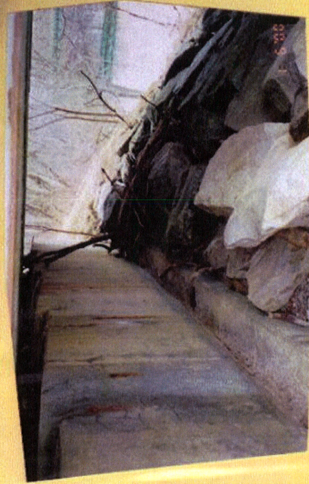
Concrete deterioration. S/ly footing exp'd \leq 0.7' vertical. Appears to be drift accum. inc. on bridge seats.
