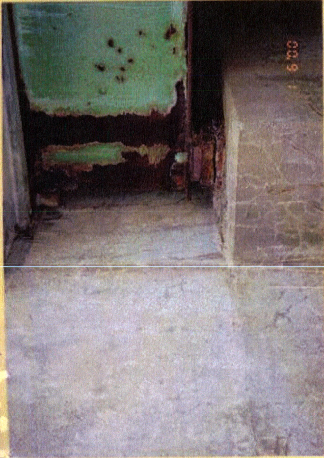
Corrosion defer. w. penetration est. \leq 3/16" .
