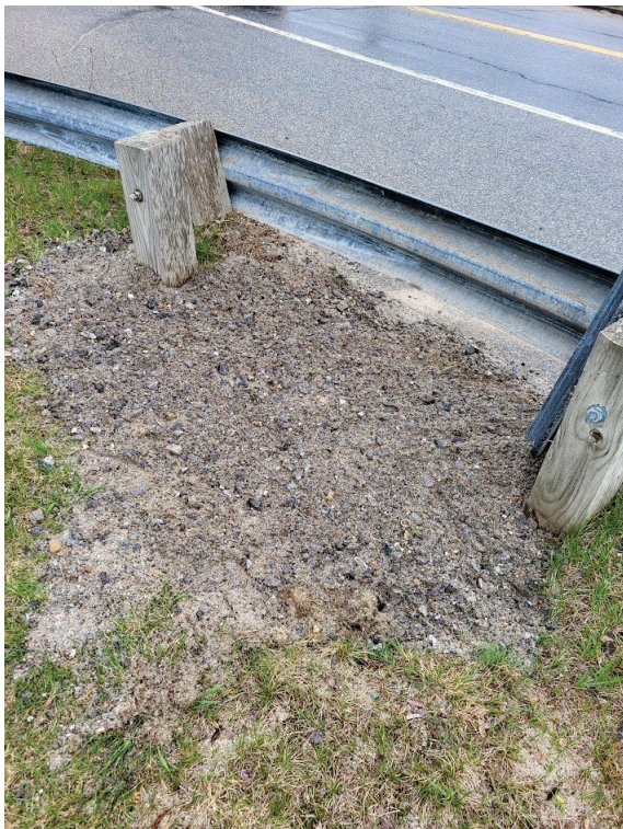
Sink hole caused by damaged outfall pipe, filled in by MDOT crew.
