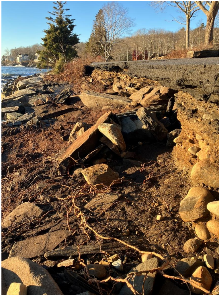
Road Shoulder Erosion
