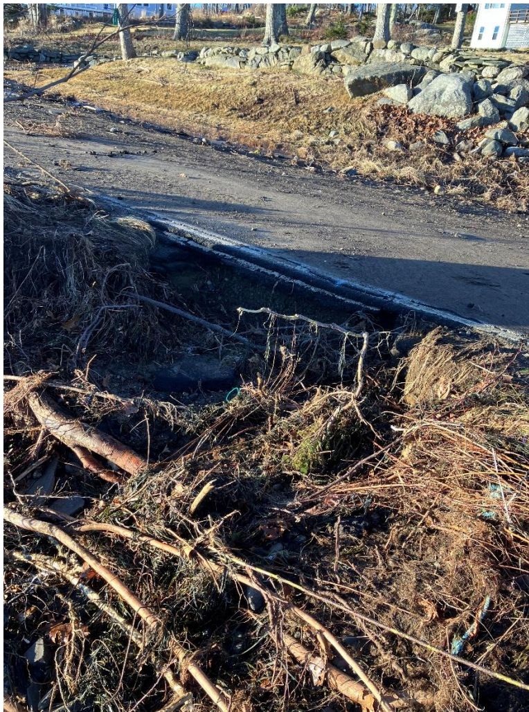
Road Shoulder Erosion
