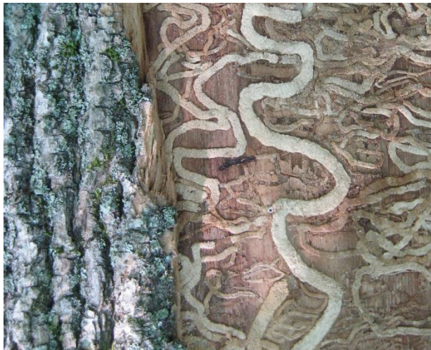
Notice EAB tracks hidden under undamaged bark
