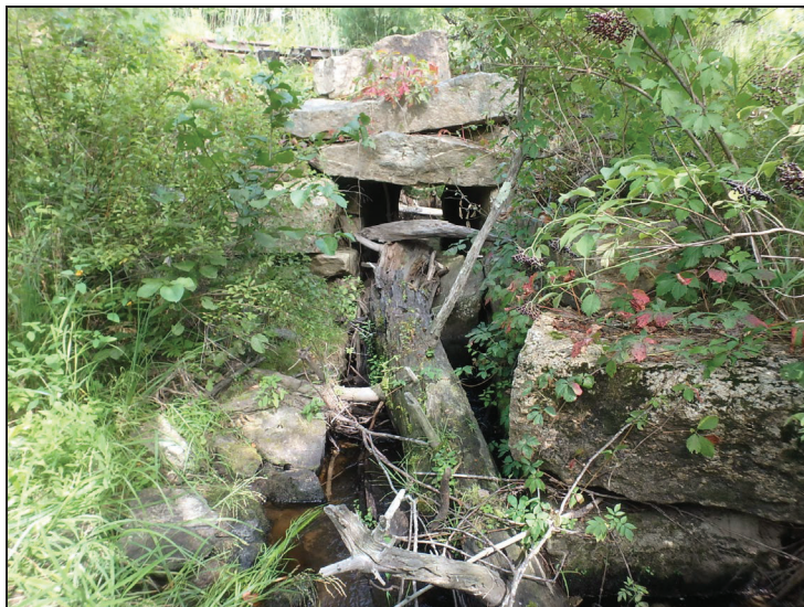
Image 2 – Debris at Culvert Inlet (Little Saco)
